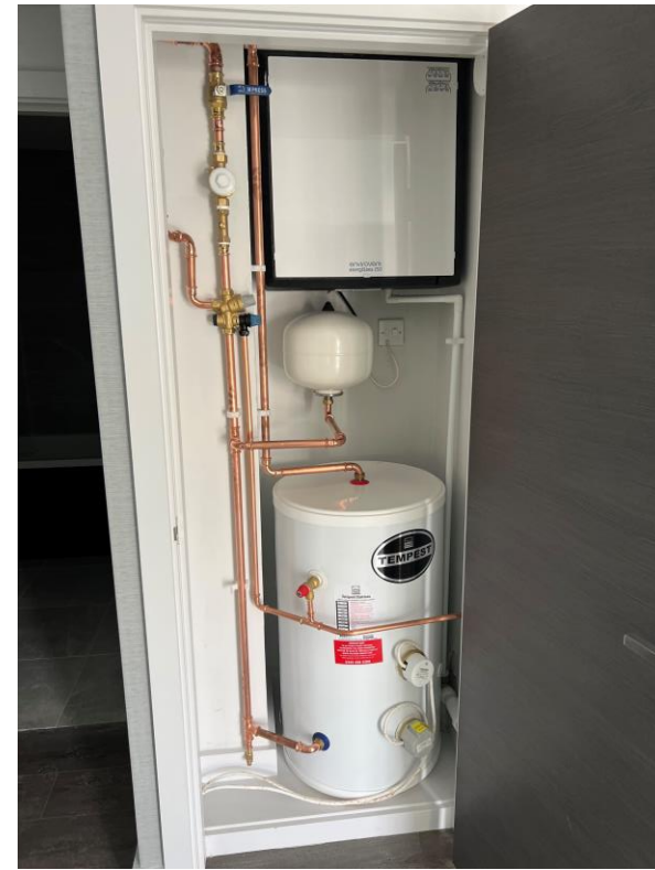
Heating ventilation system & water cylinder
