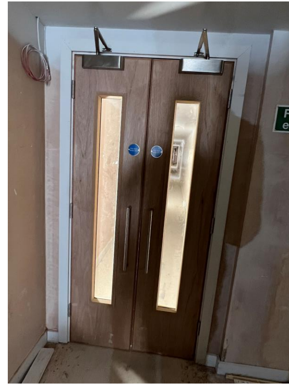
Fire doors installed to circulation areas
