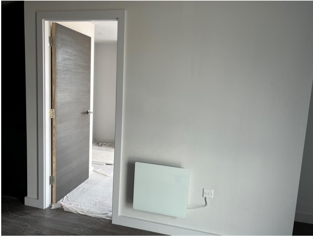
Bedroom radiators installed
