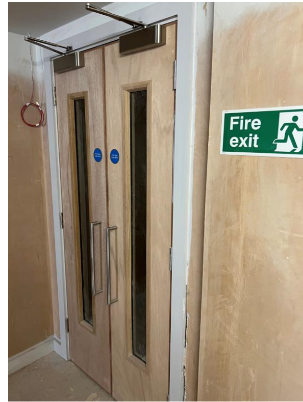
Fire doors installed to circulation areas
