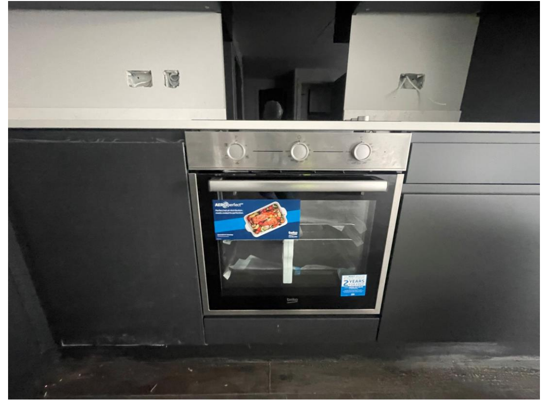
Block A – Appliances installed
