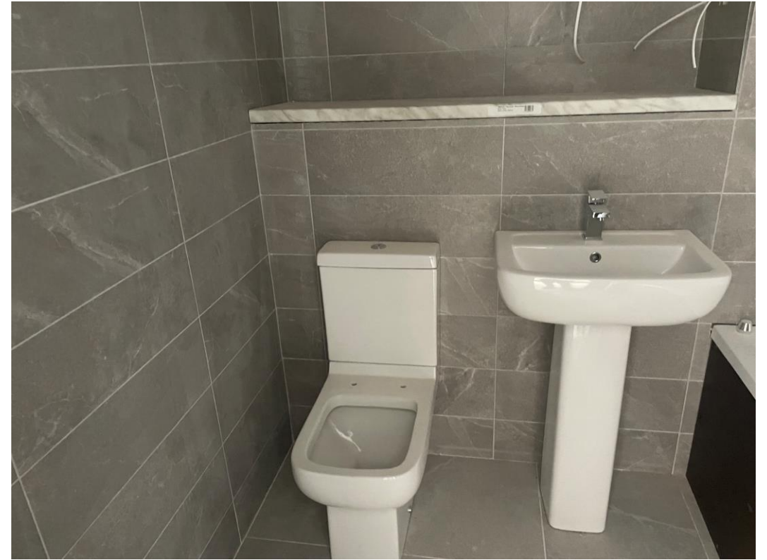
Bathroom sanitary appliances installed
