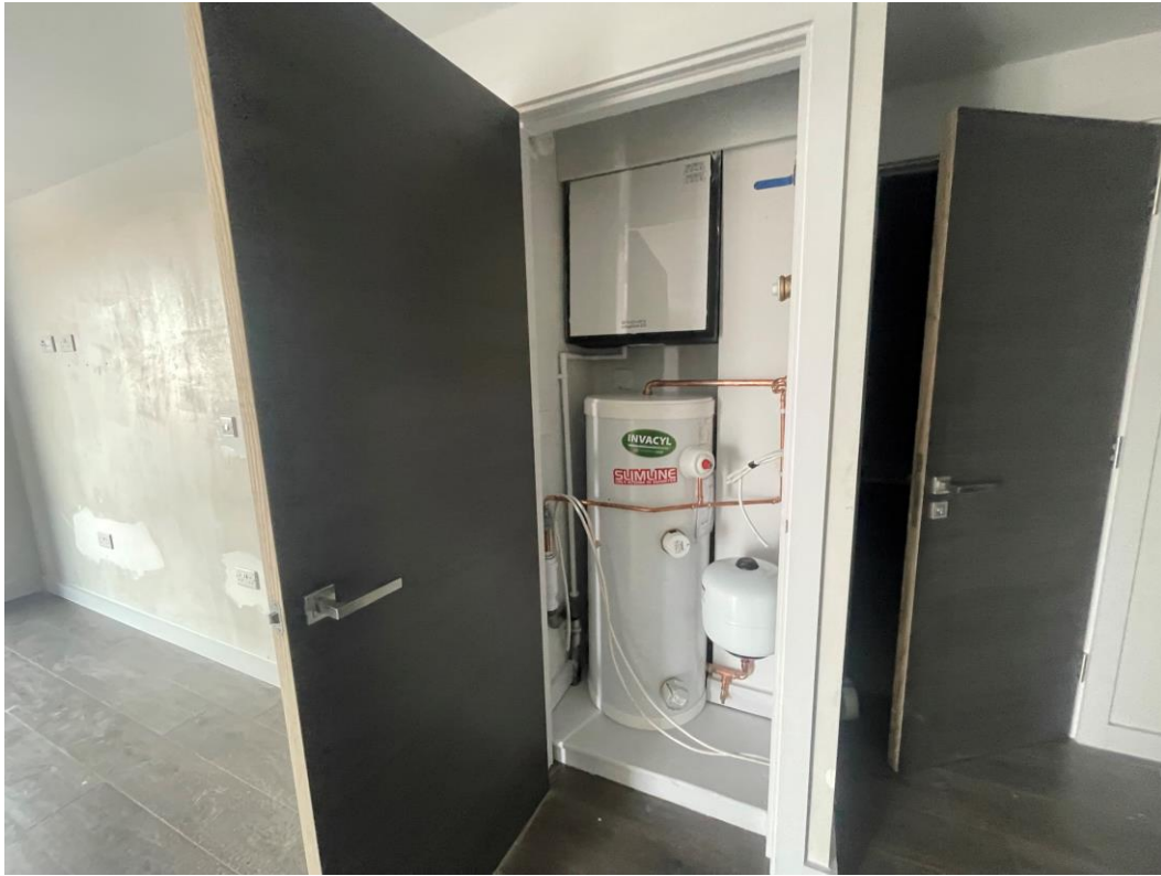
Water cylinder and ventilation unit installed
