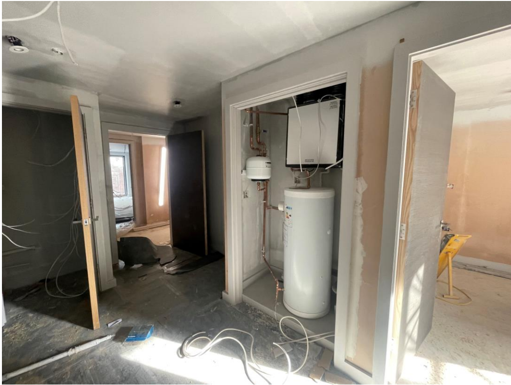
Water cylinder and ventilation unit installed
