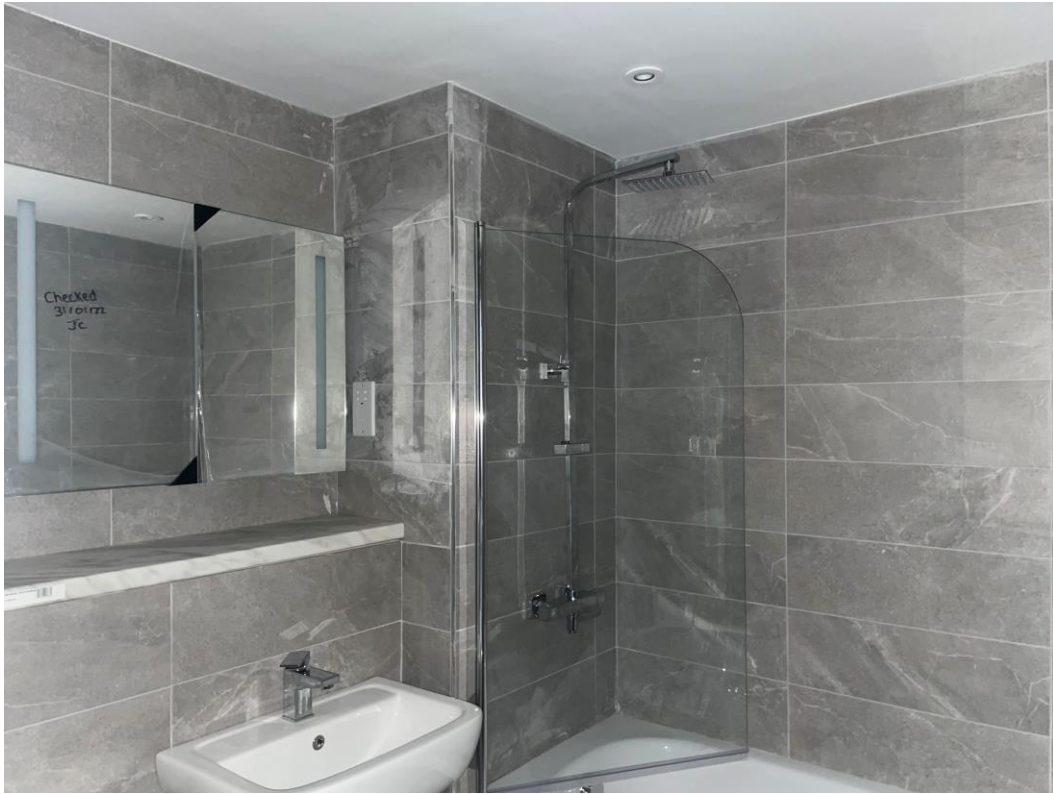
Bathroom sanitary appliances installed
