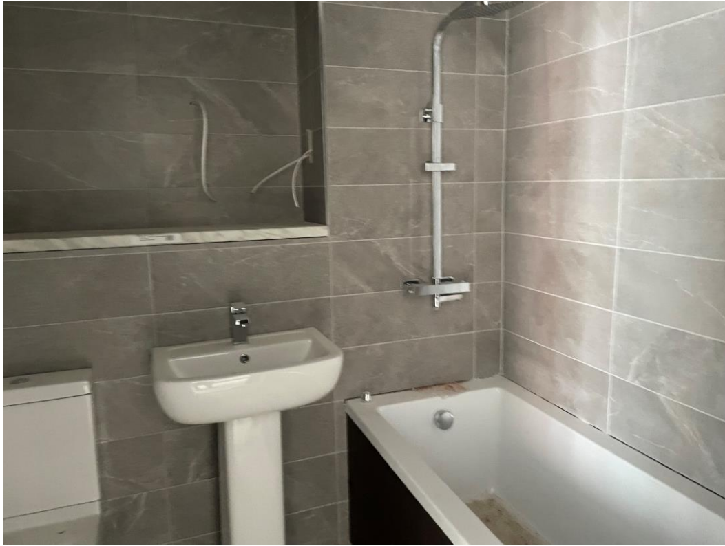
Bathroom sanitary appliances installed
