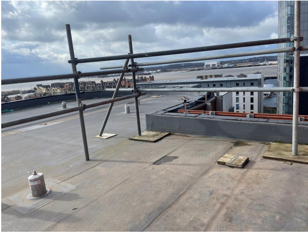
Man safe system in place
