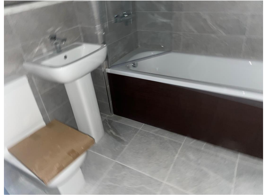
Bathroom sanitary appliances installed
