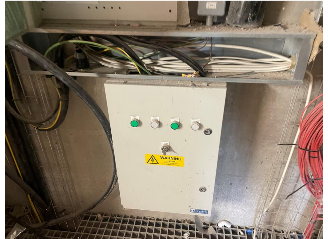
Electrics isolation unit
