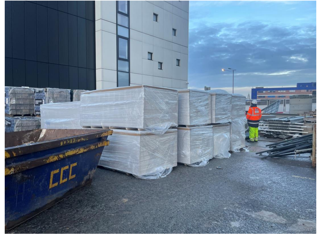
Plasterboard stored onsite
