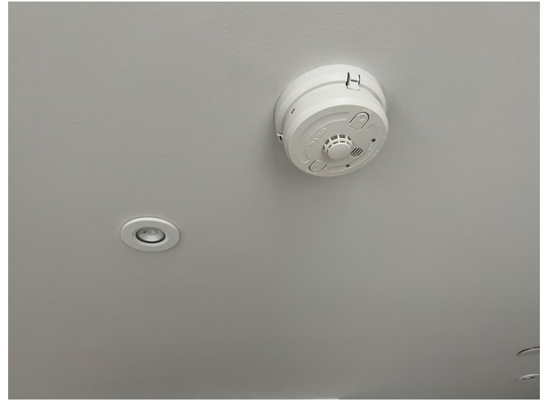
Spotlights & smoke detectors installed
