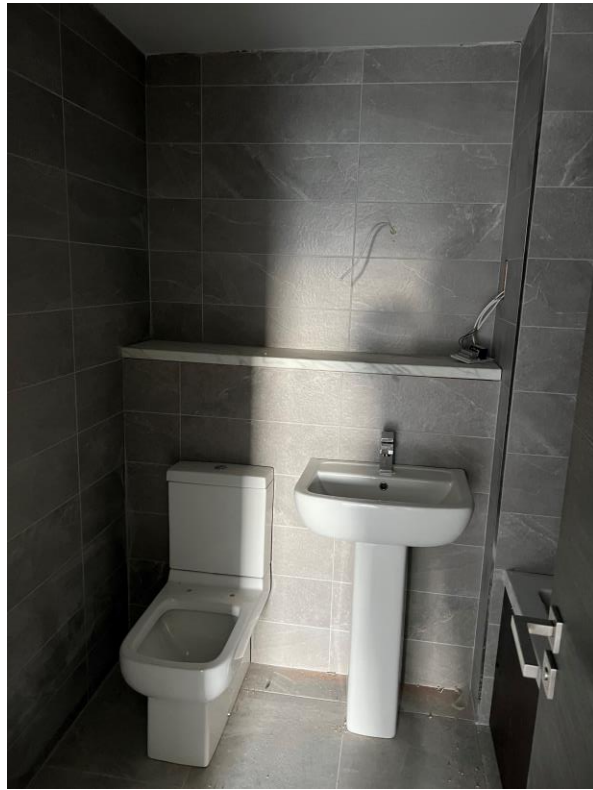
Bathroom sanitary appliances installed
