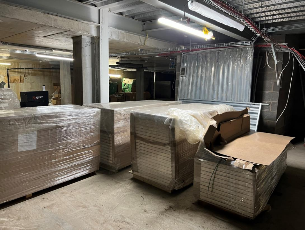
Plasterboard stored onsite
