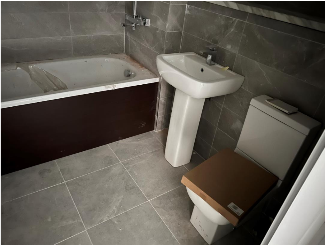
Bathroom sanitary appliances installed
