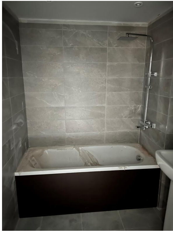
Bathroom sanitary appliances installed
