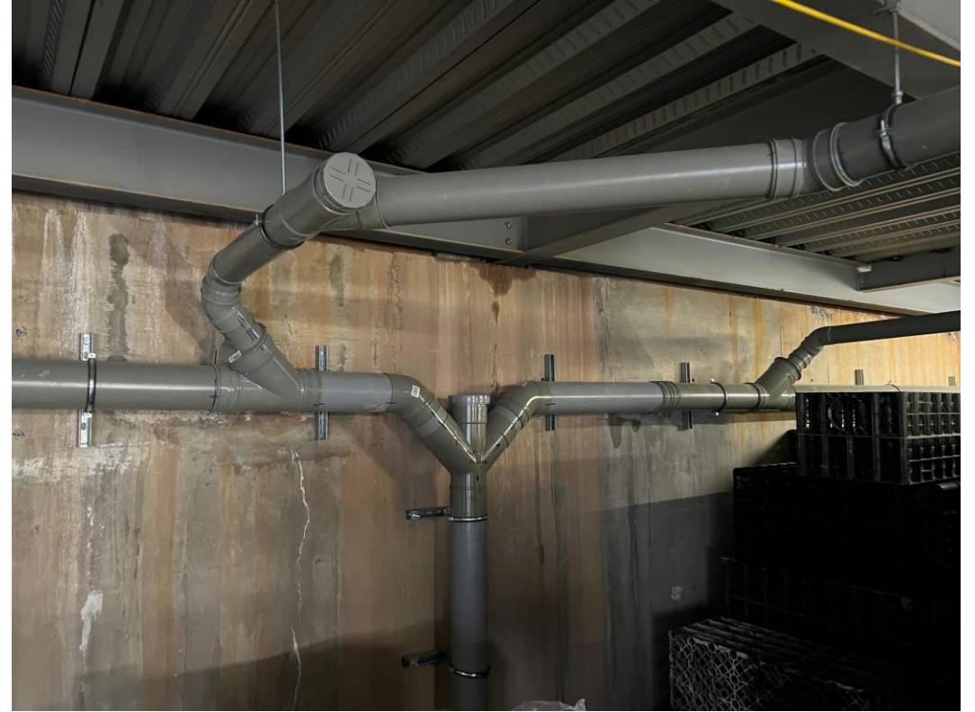
Above ground drainage system
