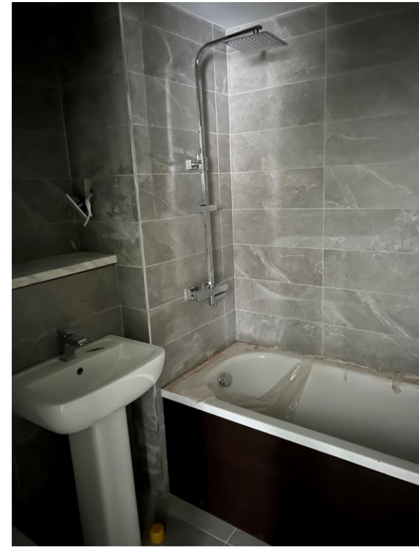
Bathroom sanitary appliances installed
