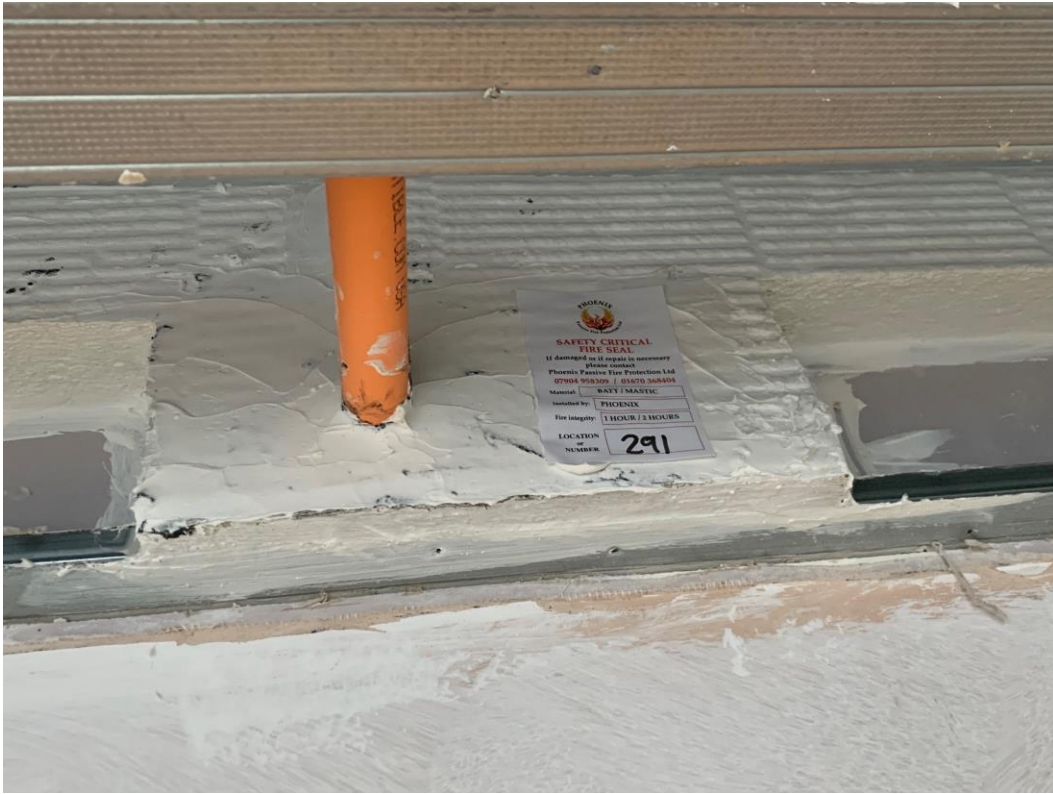
Fire stopping in apartment areas
