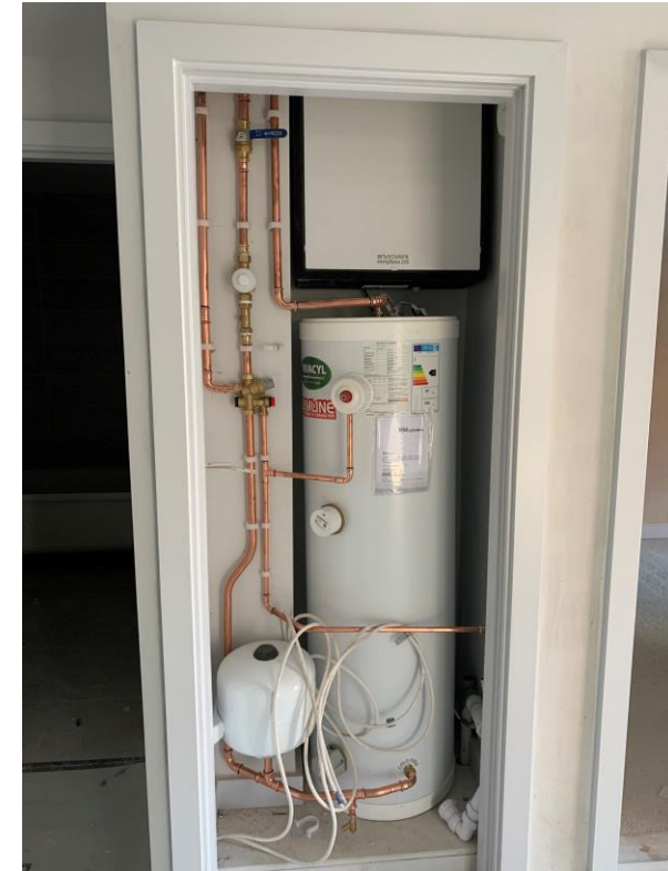
Heating ventilation & cylinder system
