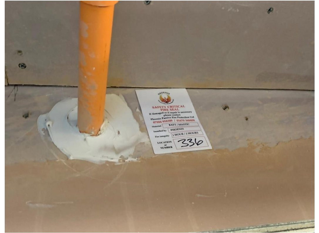
Fire stopping in apartment areas
