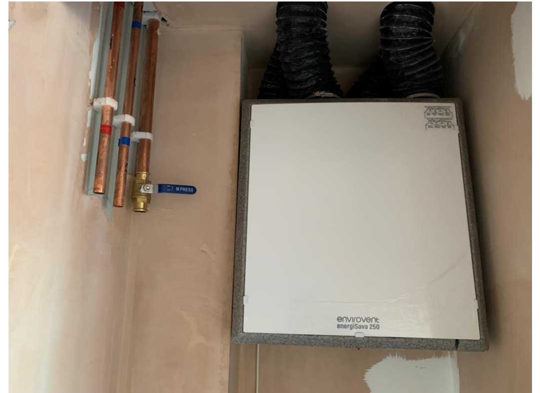
New heating ventilation system
