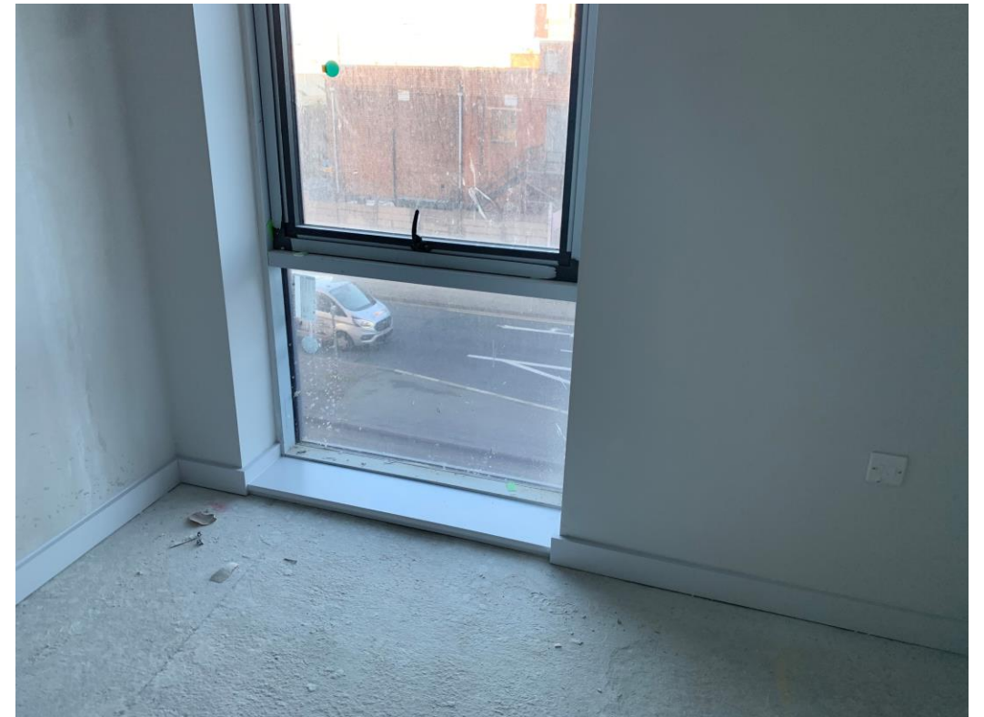
Skirting boards and window board installed. 1 st coat decoration to woodwork complete
