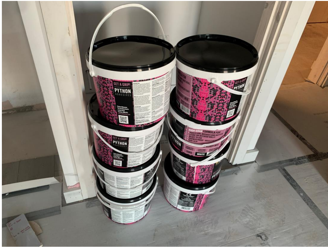
Fire stopping in apartment areas
