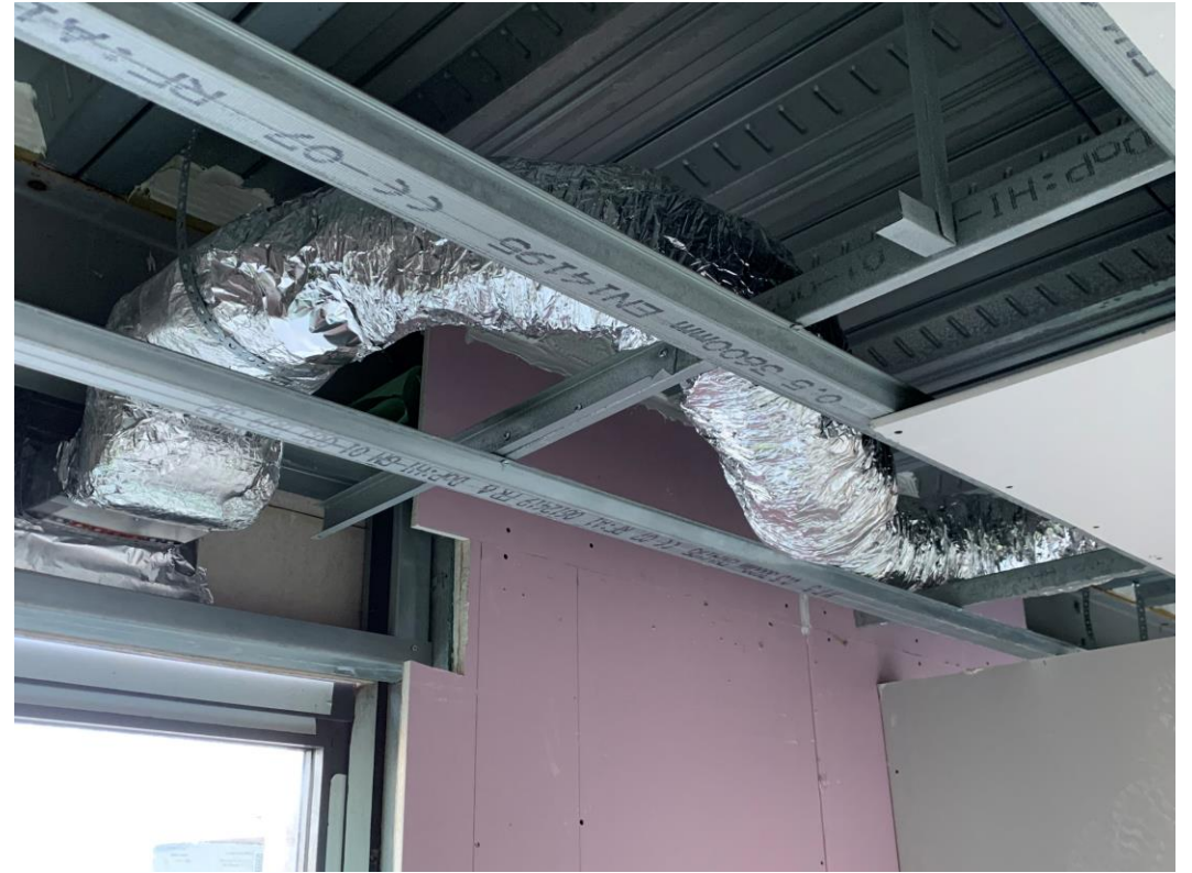
Air ventilation system
