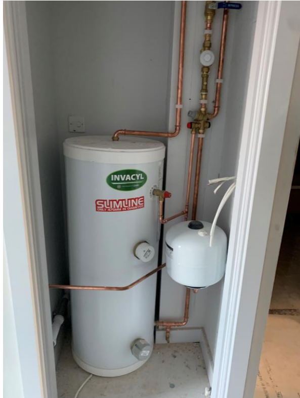
New water cylinder
