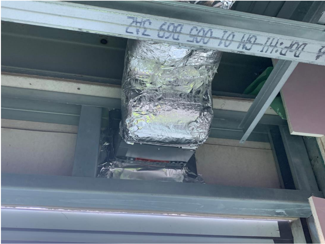
Air ventilation system
