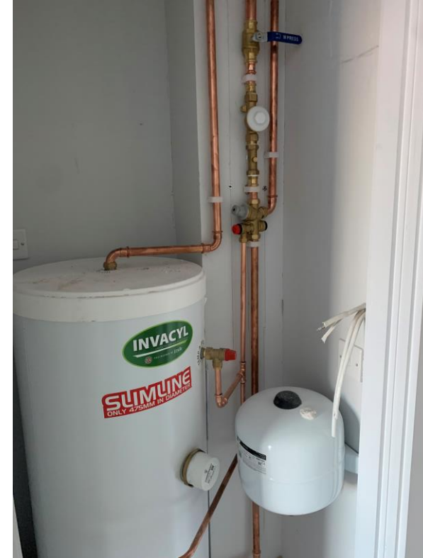
New water cylinder
