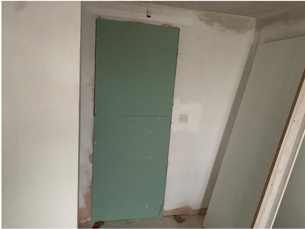
Jack & Jill bathroom door block ed up and boarded
