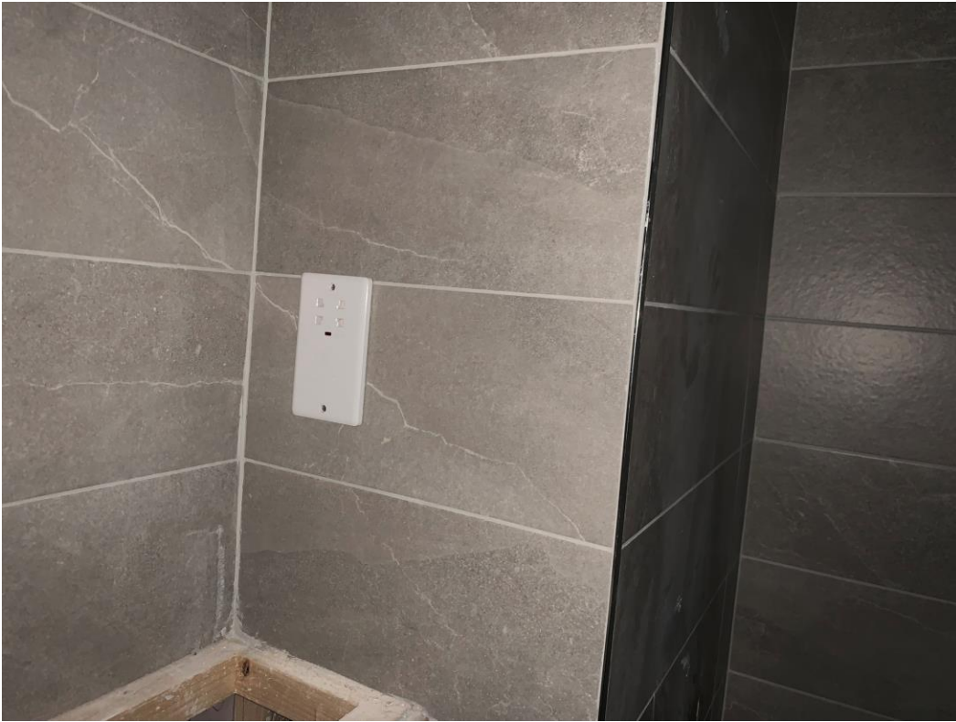
Shaving socket installed
