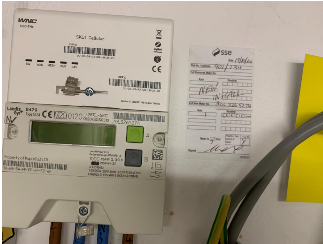
Electrics metre room
