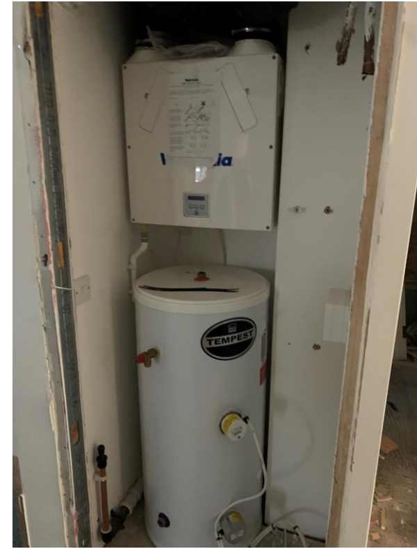
Old heating ventilation and cylinder system
