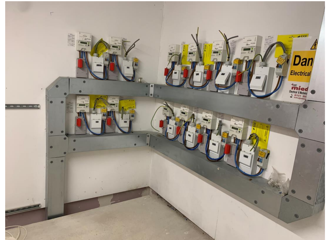
Electrics metre room
