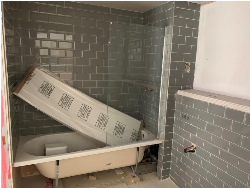
Old bathroom sanitary fittings & tiling variation
