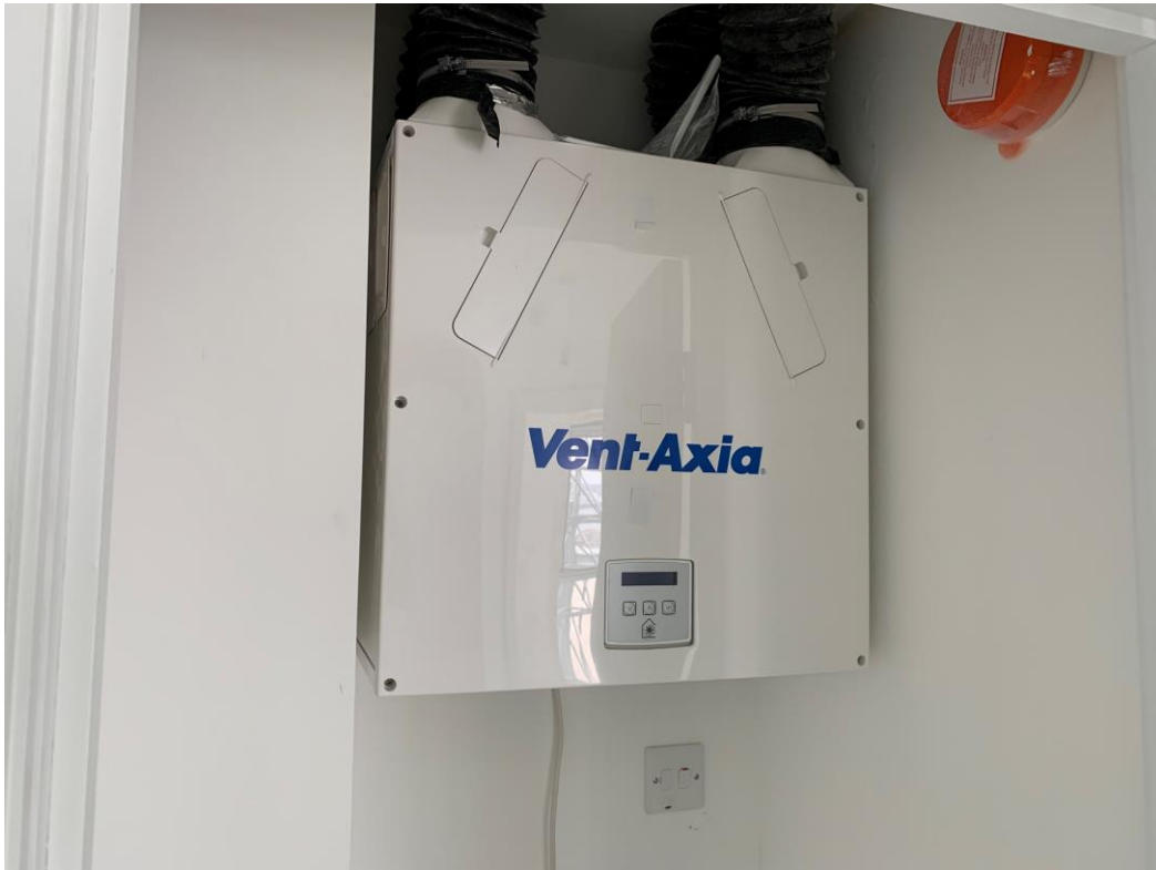
Old Vent-Axia heating unit
