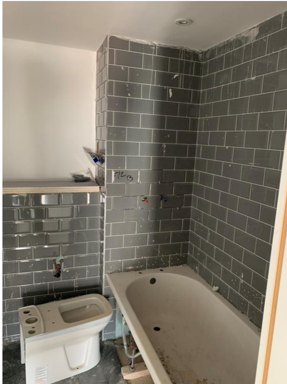
Old bathroom sanitary fittings & wall tiling variation
