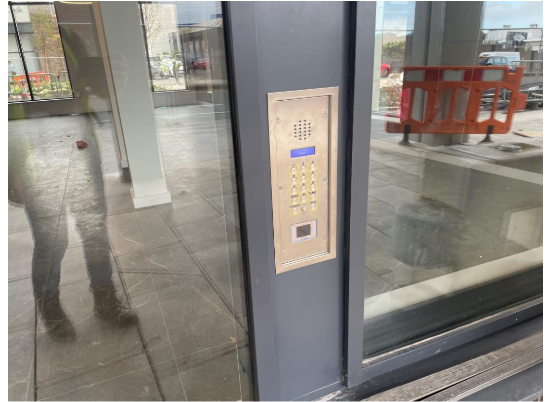
Main entrance intercom installed
