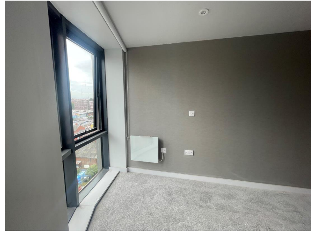
Bedroom radiators installed
