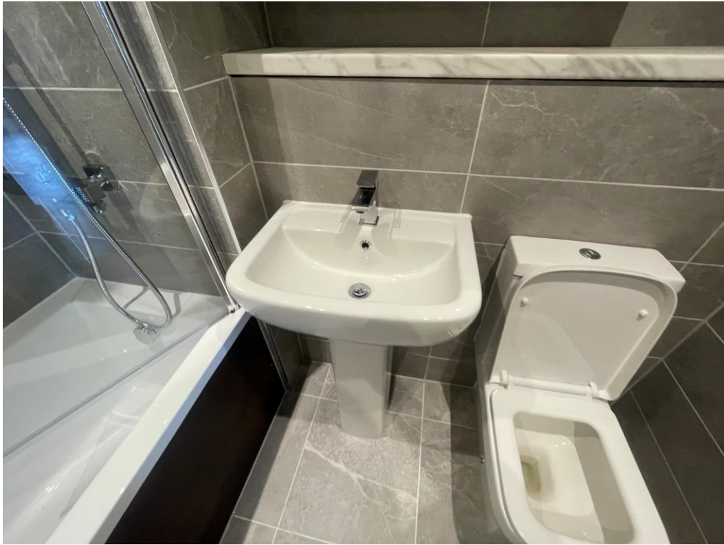
Bathroom sanitary appliances installed
