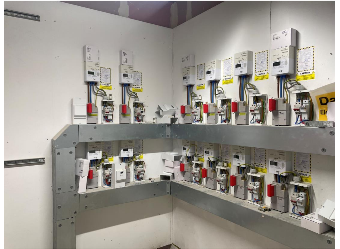
Apartment electrical meters installed
