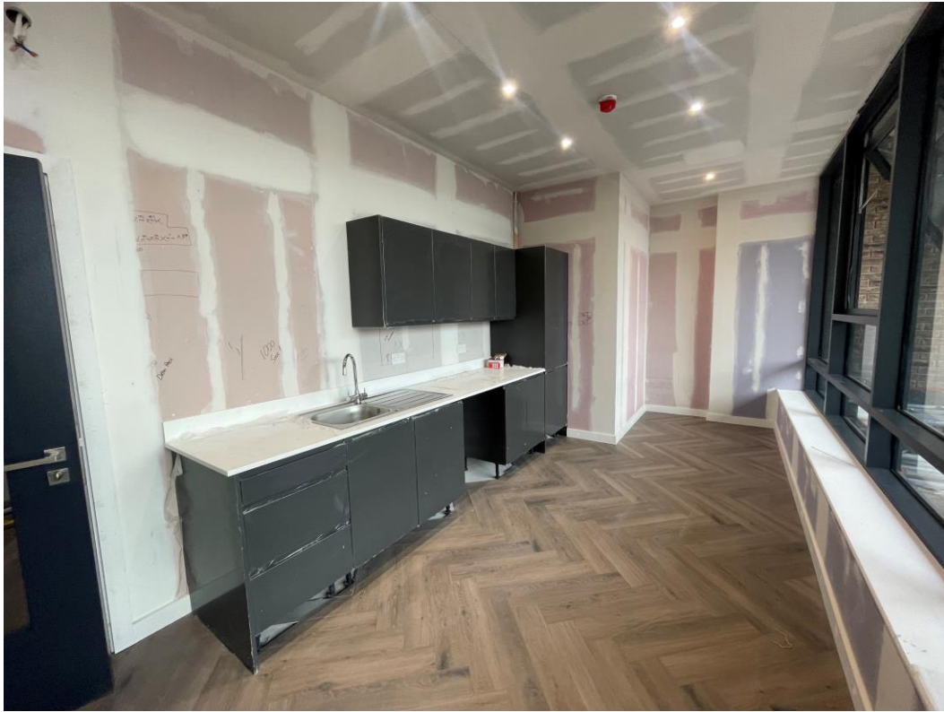
Communal kitchen installed
