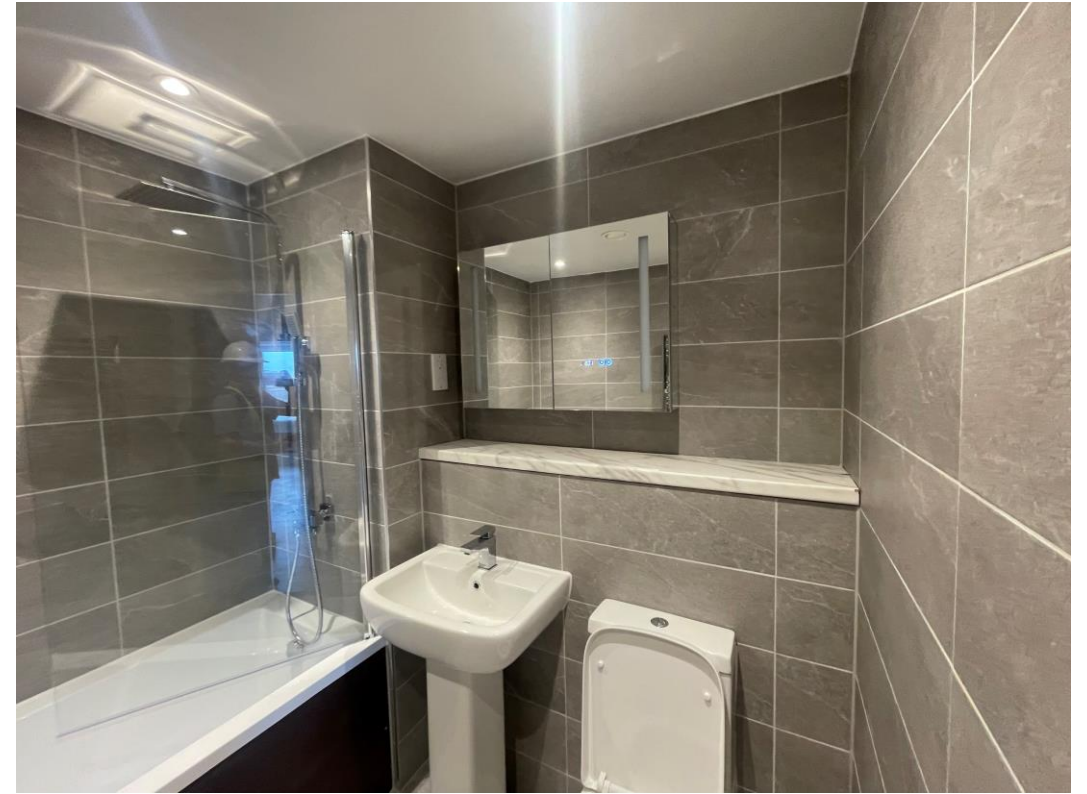
Bathroom sanitary appliances installed
