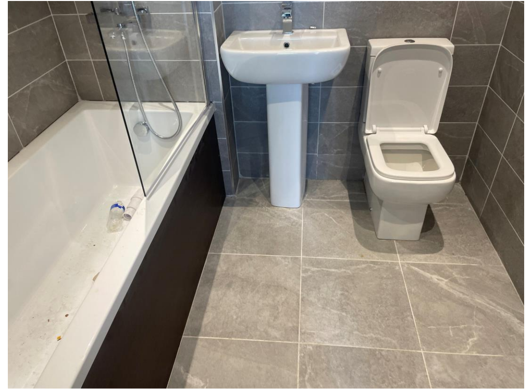
Bathroom sanitary appliances installed
