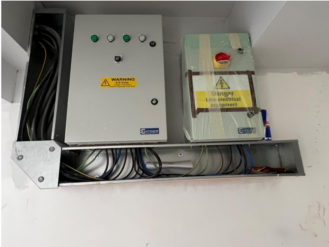
Power isolation for lift
