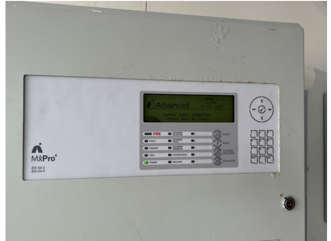
Fire alarm panel installed
