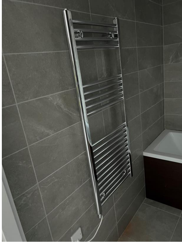
Show Flat – Bathroom Radiator
