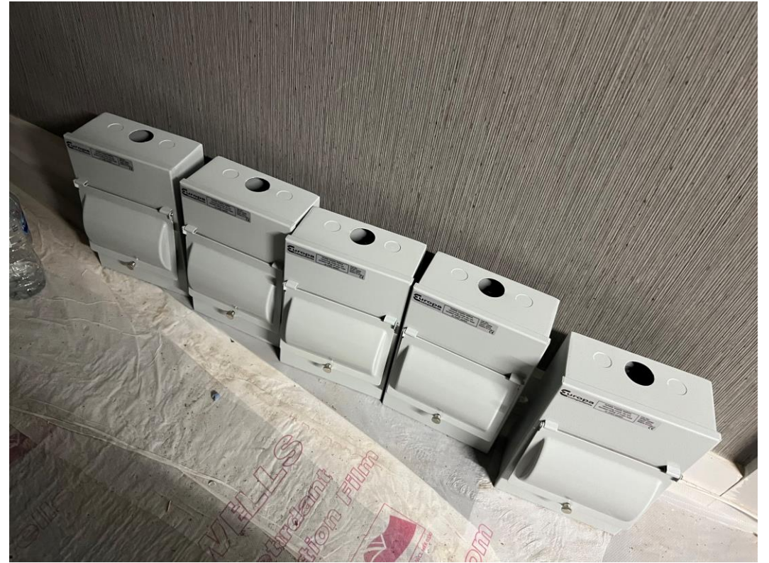
Service room consumer unit boxes
