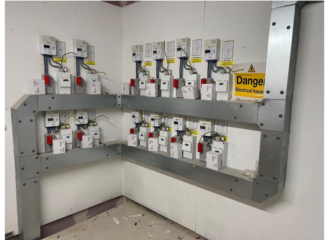
Apartment electrical meters installed
