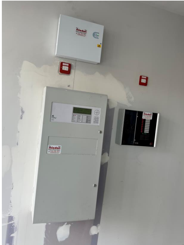
Fire alarm panel installed
