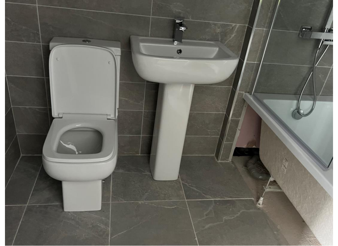
Ground Floor - Bathroom sanitary items
