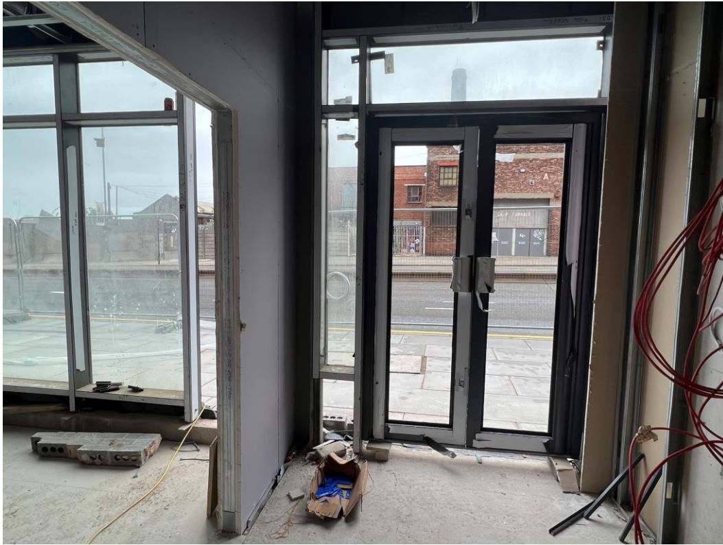
Electrical cable onsite for installation
