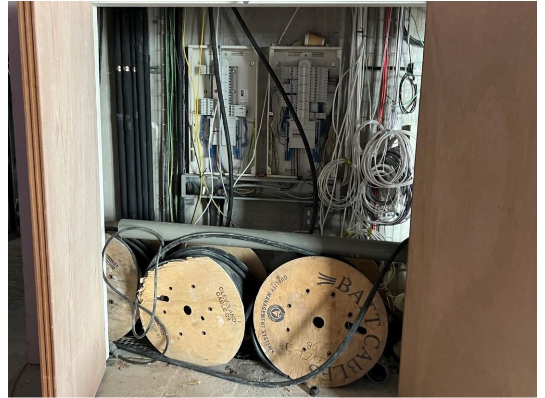
Electrical cable onsite for installation
