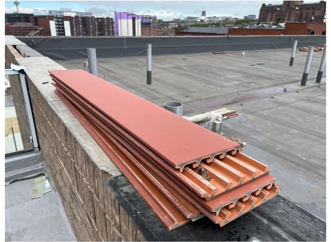
Terracotta rainscreen cladding panels
