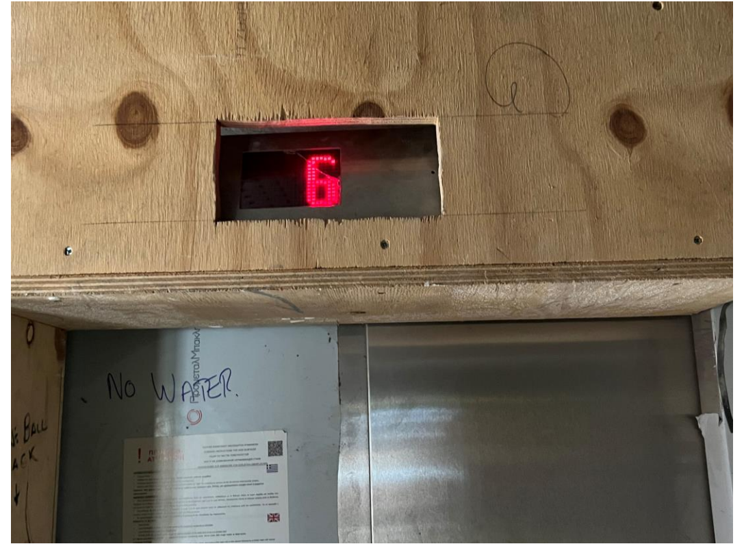
Internal lift in operation
