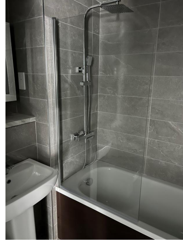
Show Flat – Bathroom Sanitary Items
