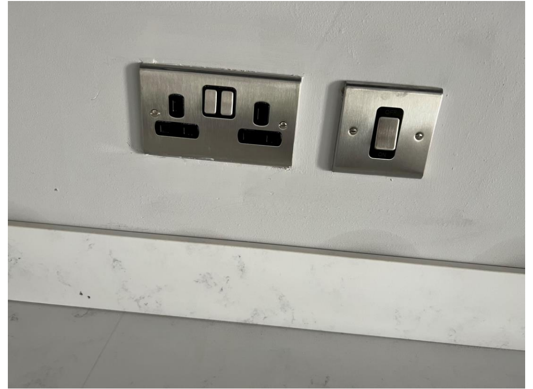
Chrome kitchen sockets & switch
