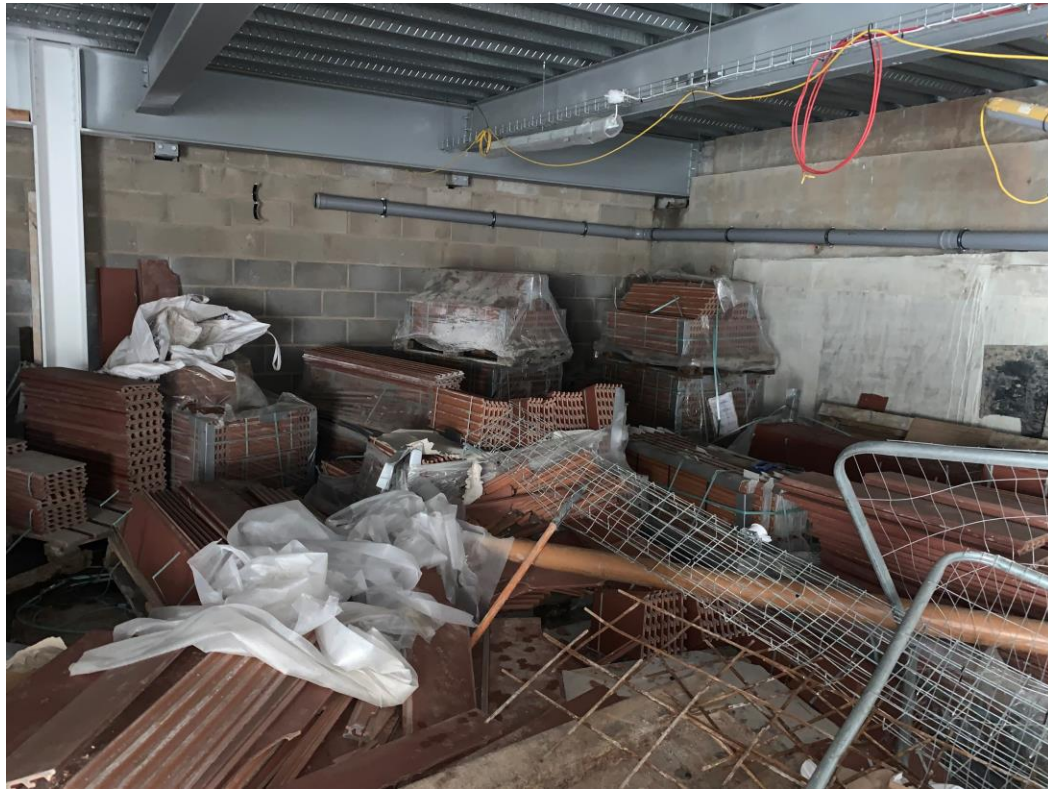
Basement cladding materials stored
