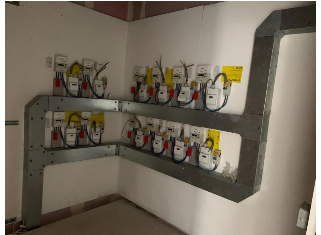
Apartment electrical meter room upper floors
