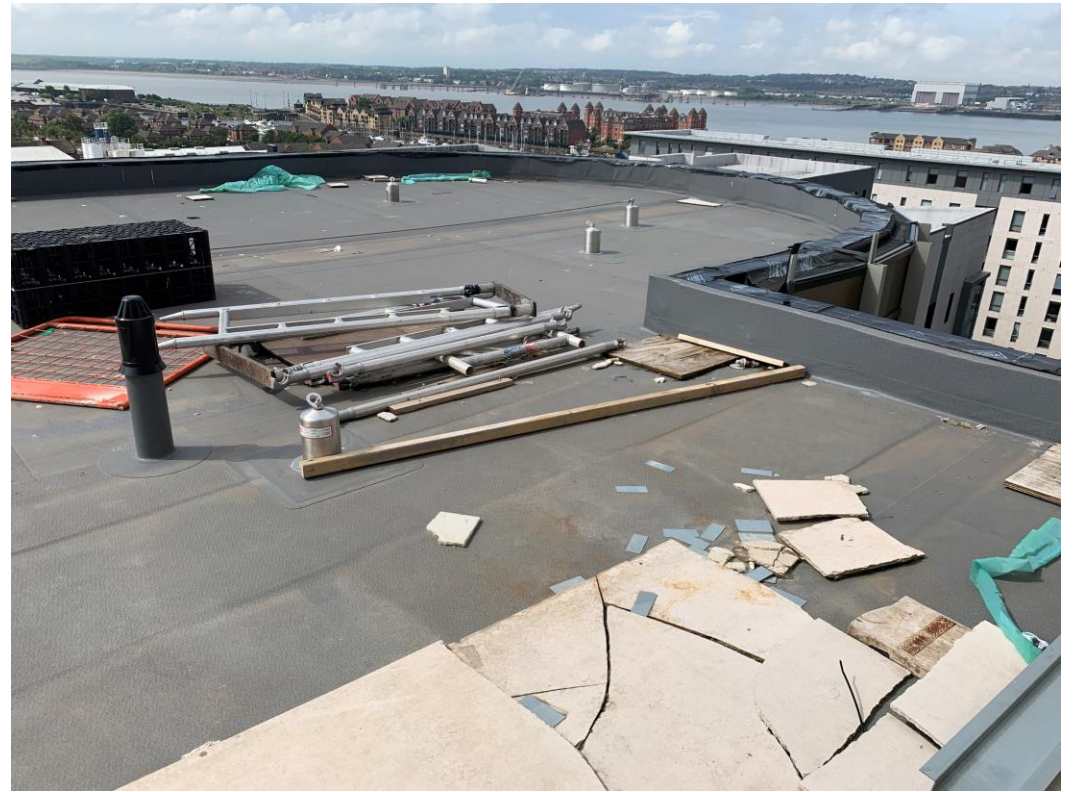
Roof mansafe system
