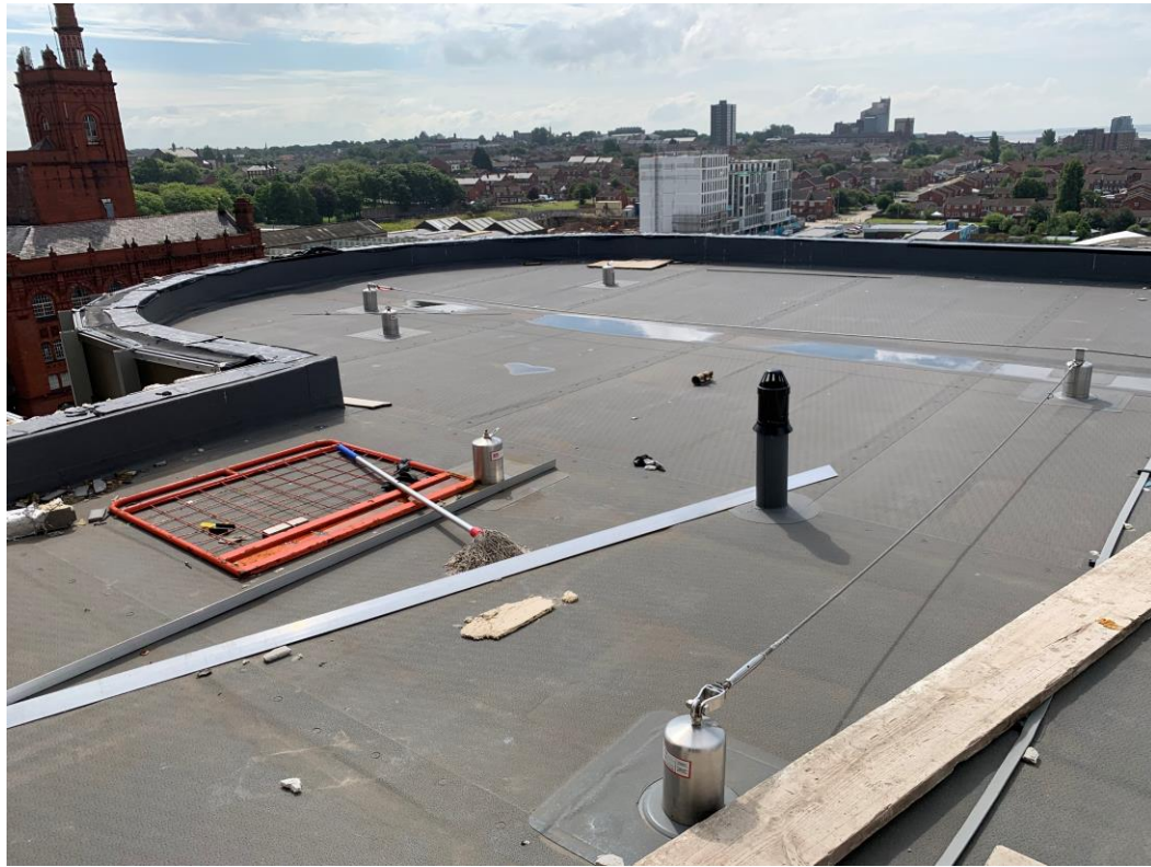
Roof mansafe system
