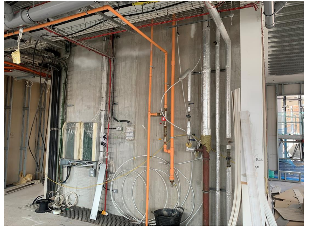
Ground Floor mains electrical services
