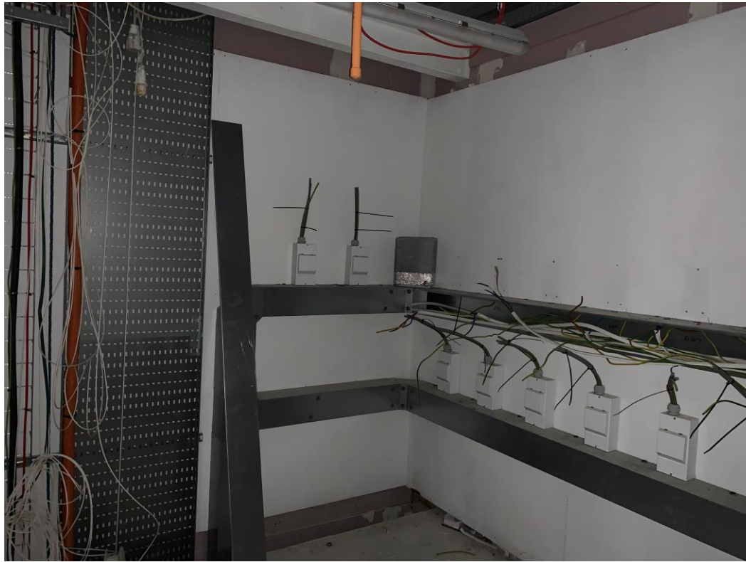
Apartment electrical meter room upper floors
