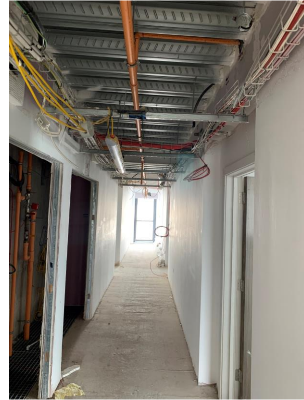
Sprinkler system installed corridor upper floors
