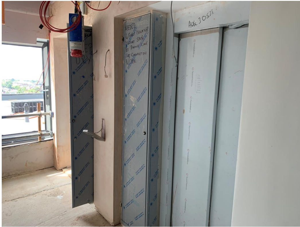
Lifts installed upper floors
