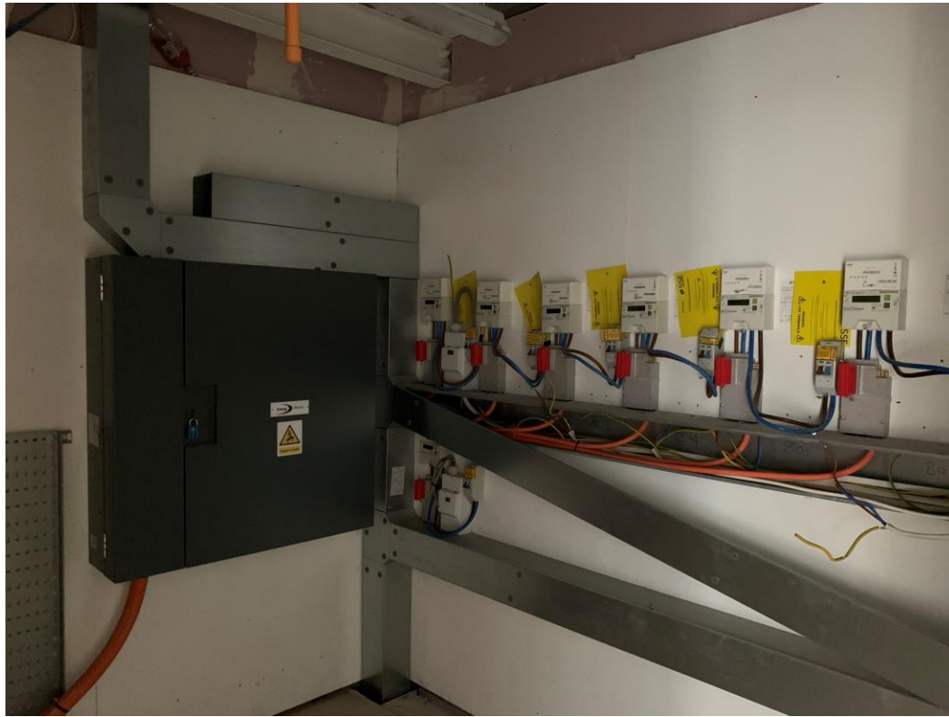
Apartment electrical meter room upper floors
