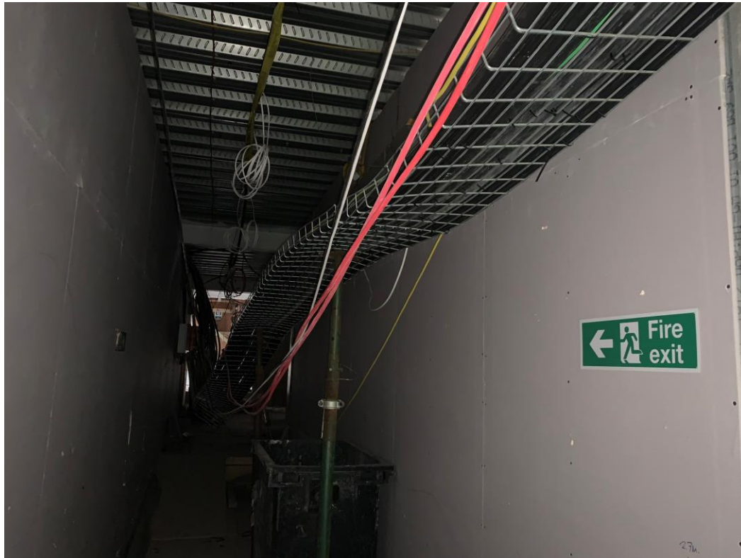
Ground Floor mains electrical services
