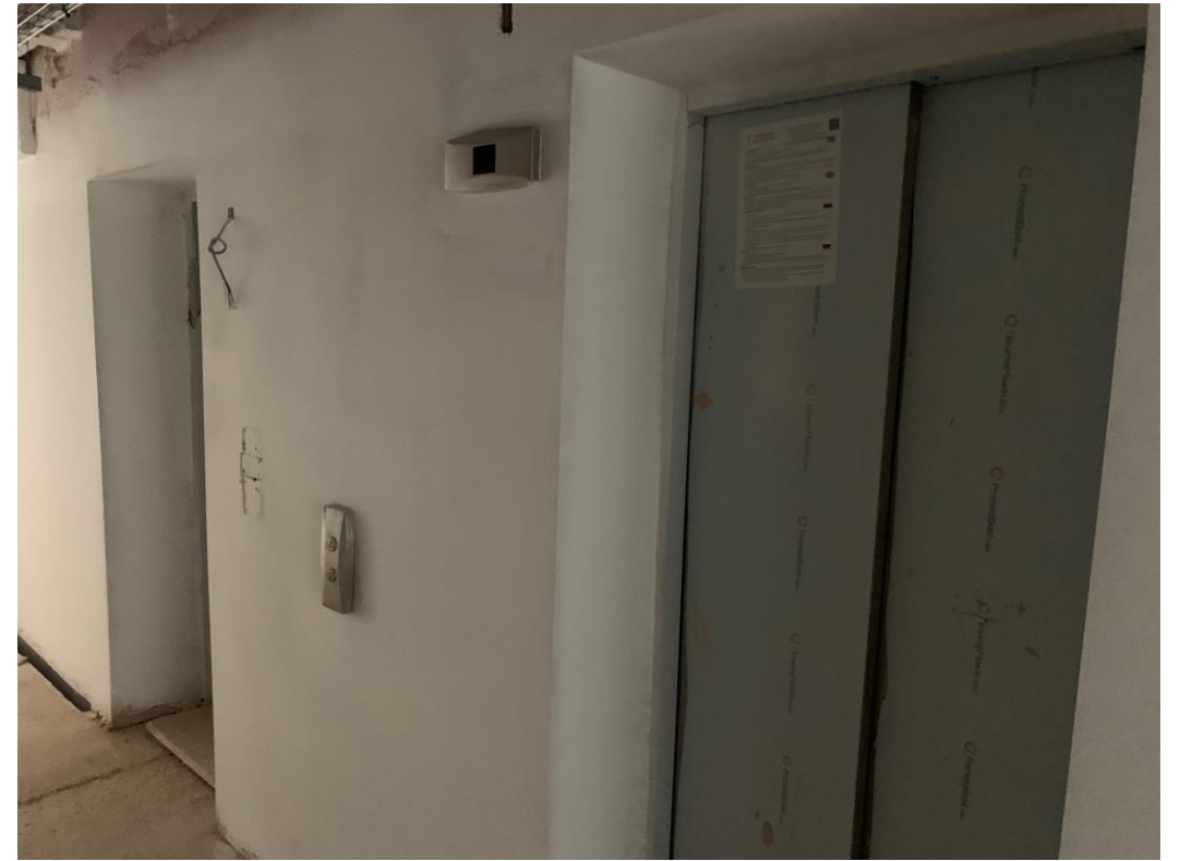
Lifts installed upper floors
