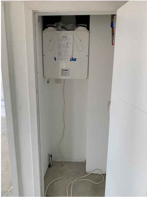
Mechanical ventilation unit installed
