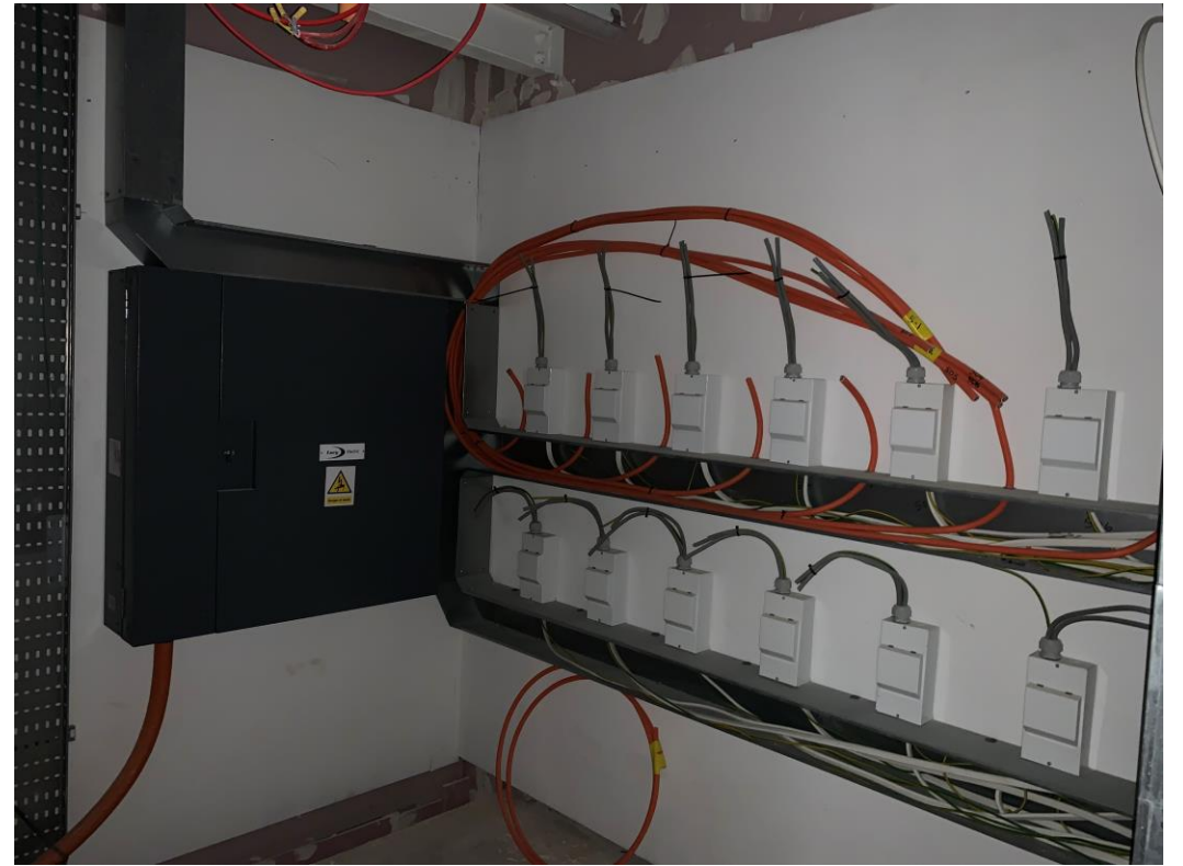
Apartment electrical meter room upper floors
