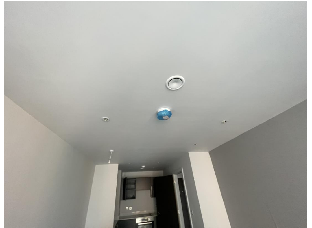
Level 5 – Kitchen smoke heads installed
