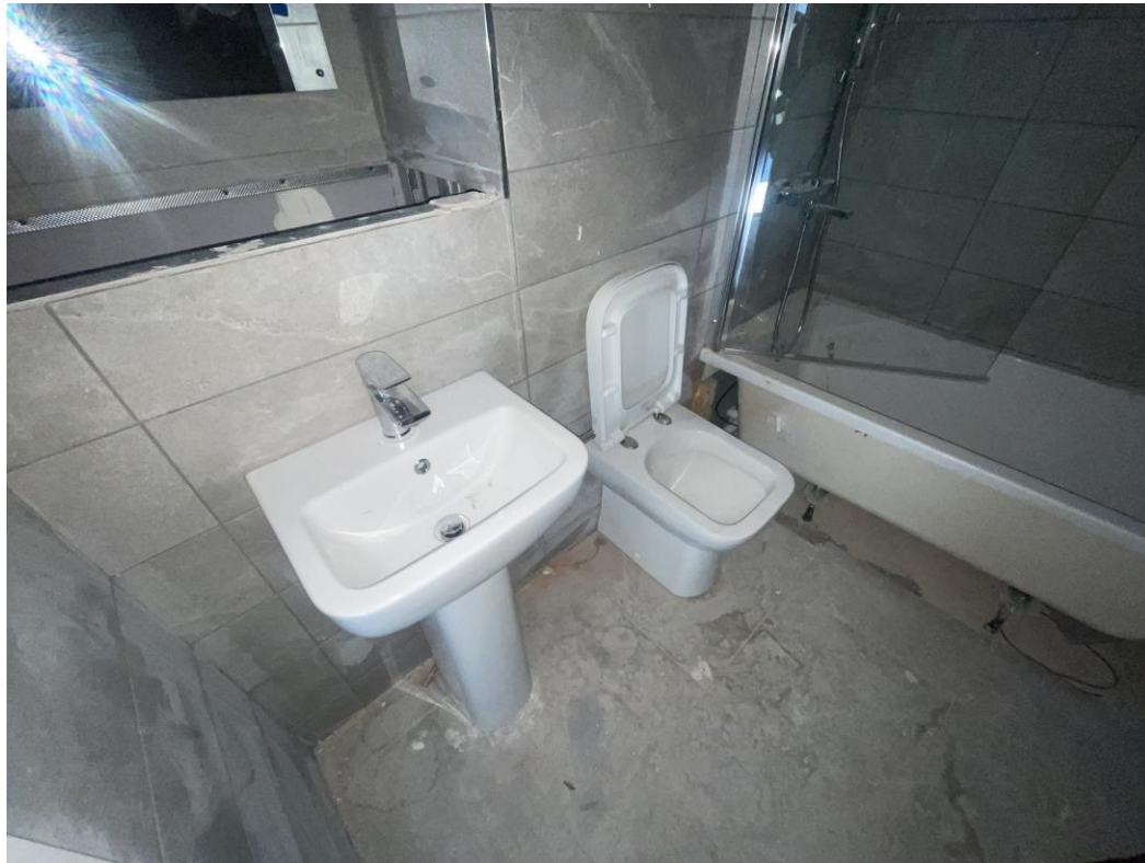
Level 8 – Bathroom sanitary appliances
