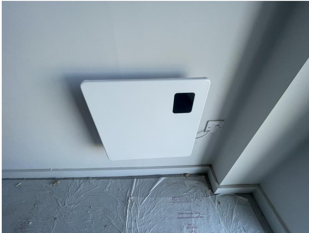
Level 5 – Heating panel
