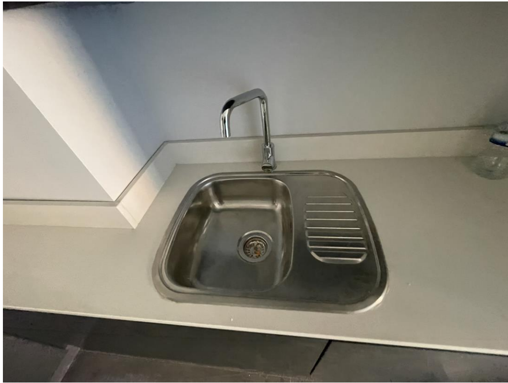
Level 2 – kitchen sink installed
