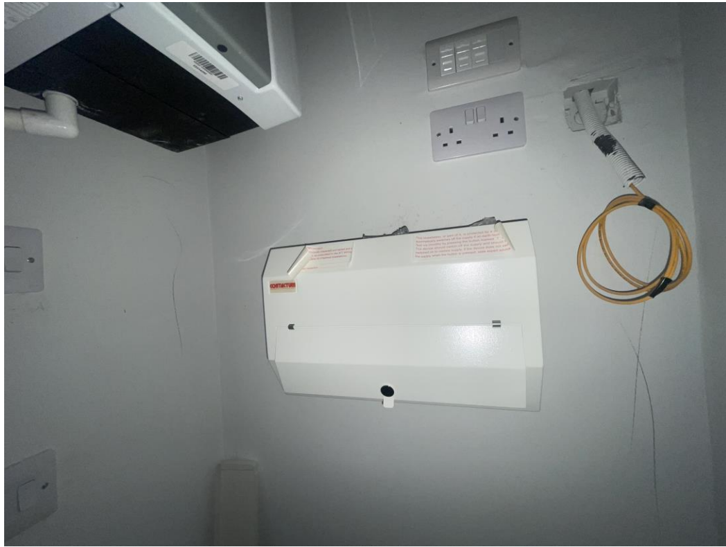
Level 2 – Electrical consumer unit installed
