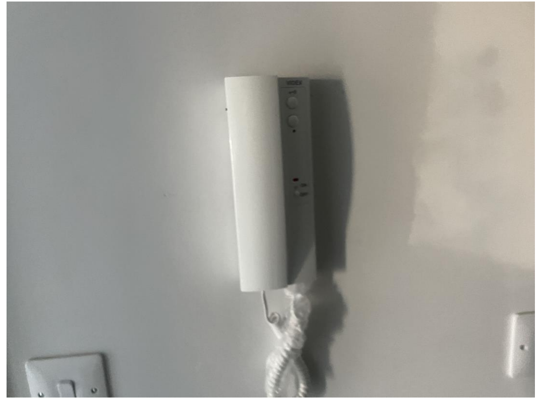
Level 3 – Apartment telecom installed
