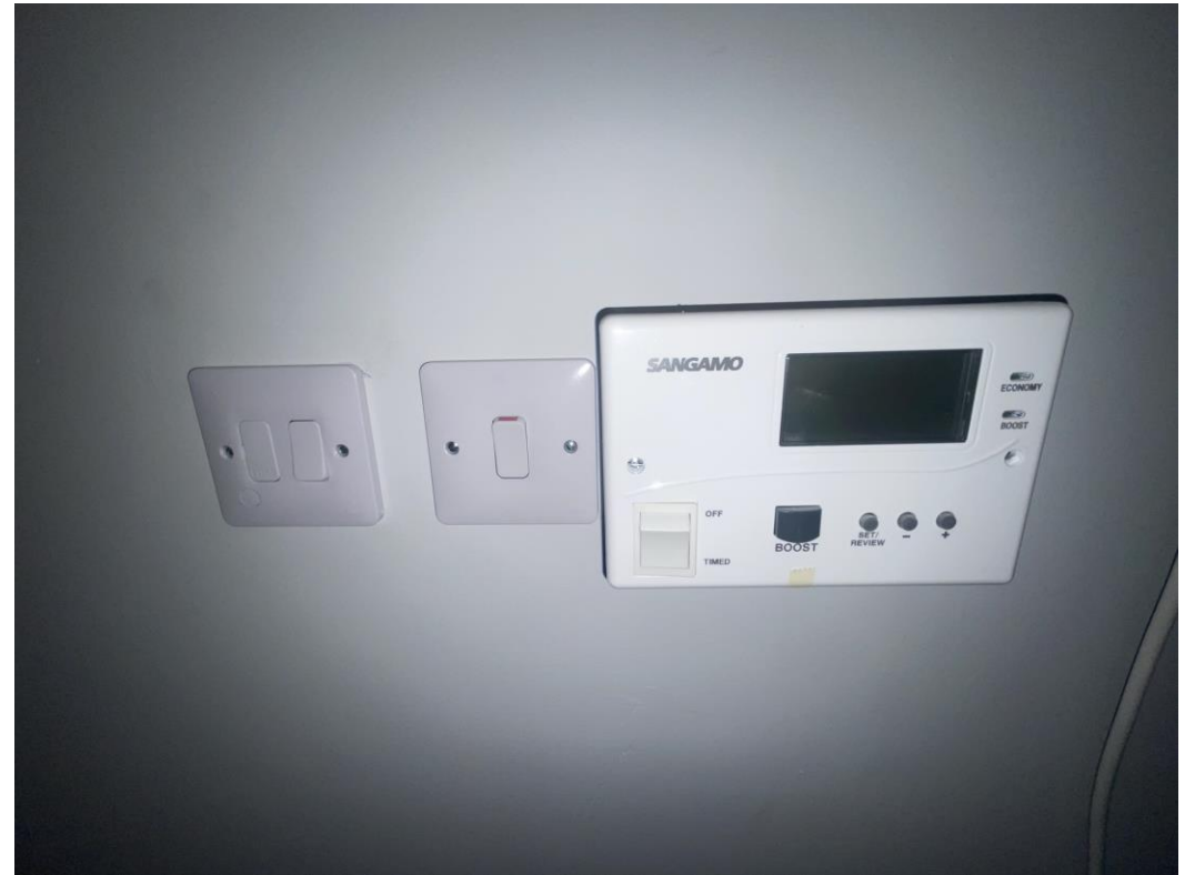
Level 6 – Heating controls
