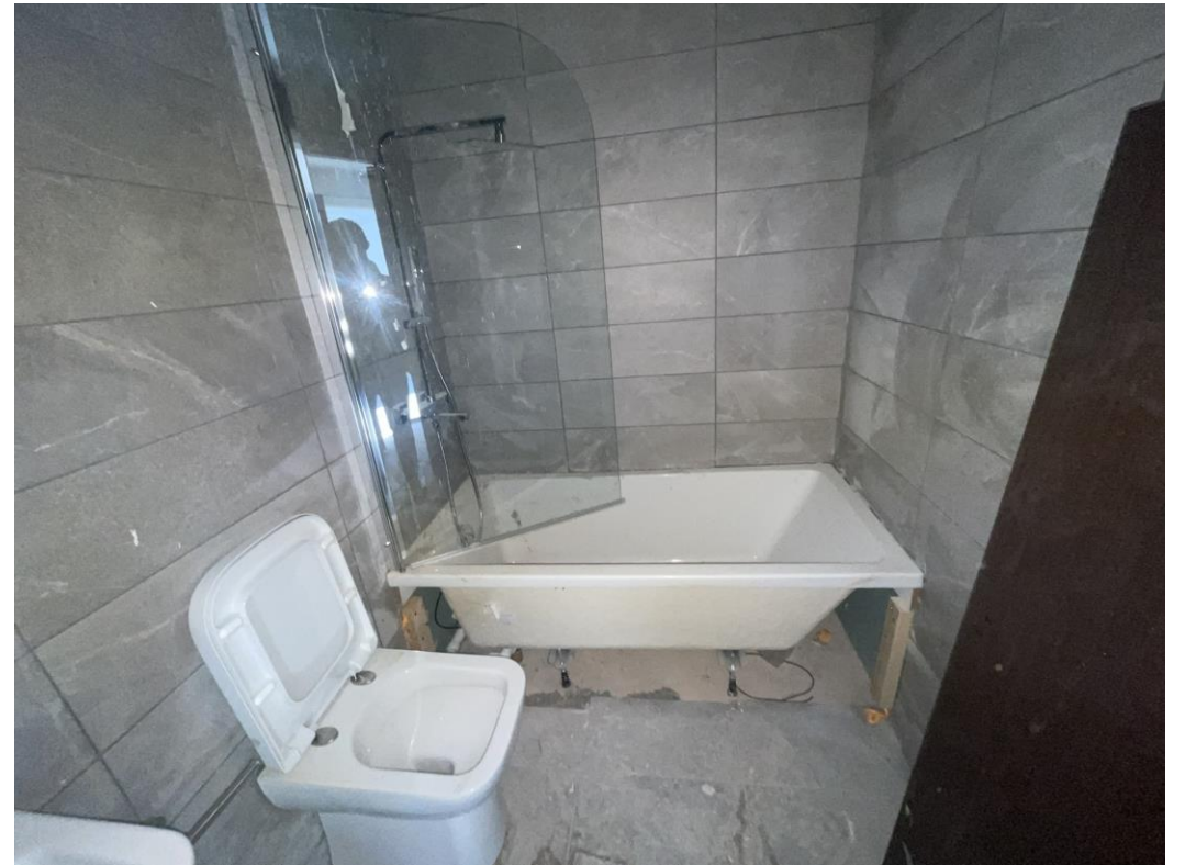
Level 8 – Bathroom sanitary appliances
