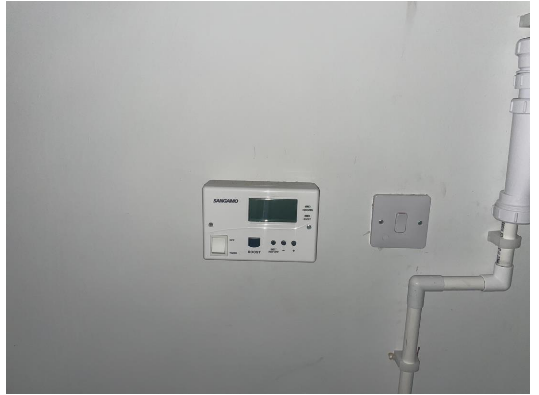
Level 2 – Heating controls installed
