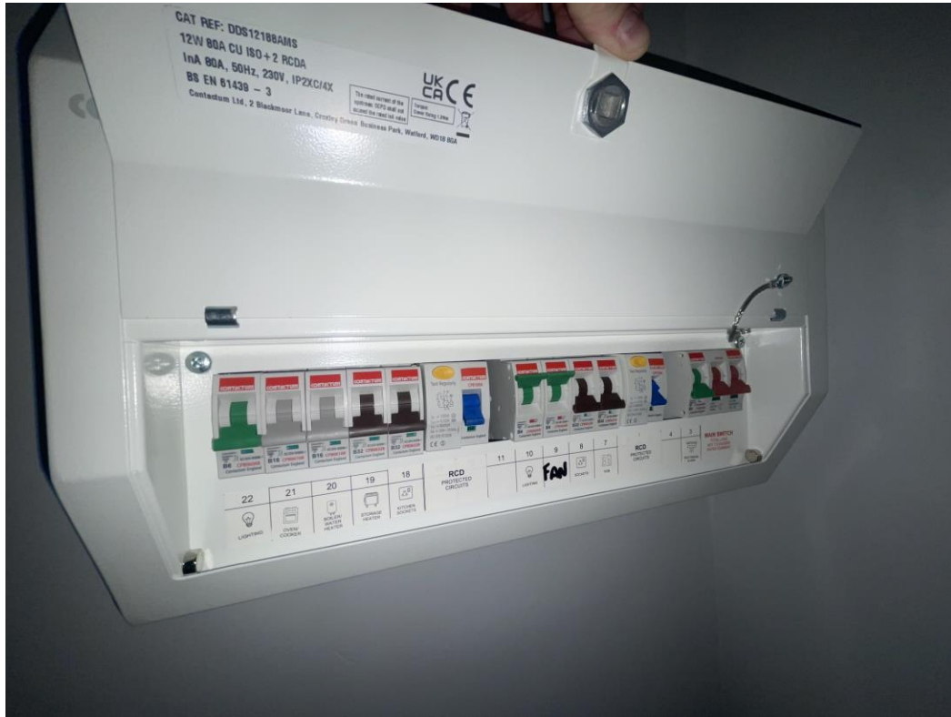
Level 6 – Electrical consumer unit
