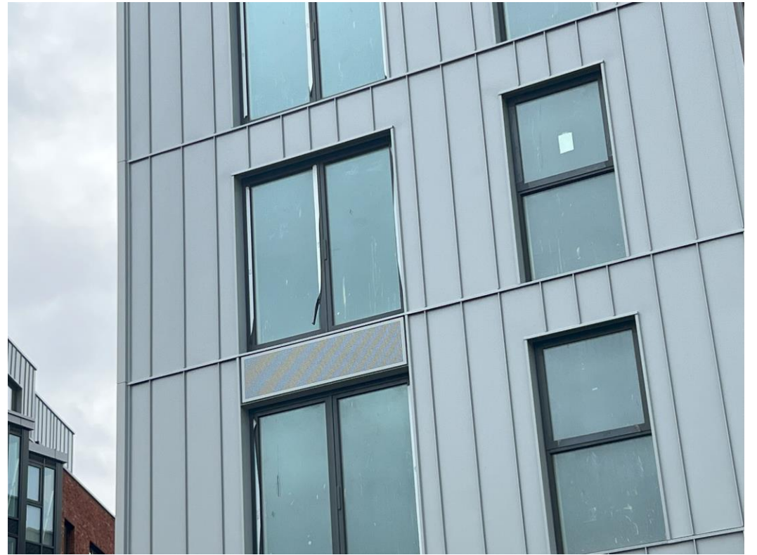
Block A Rainscreen cladding
