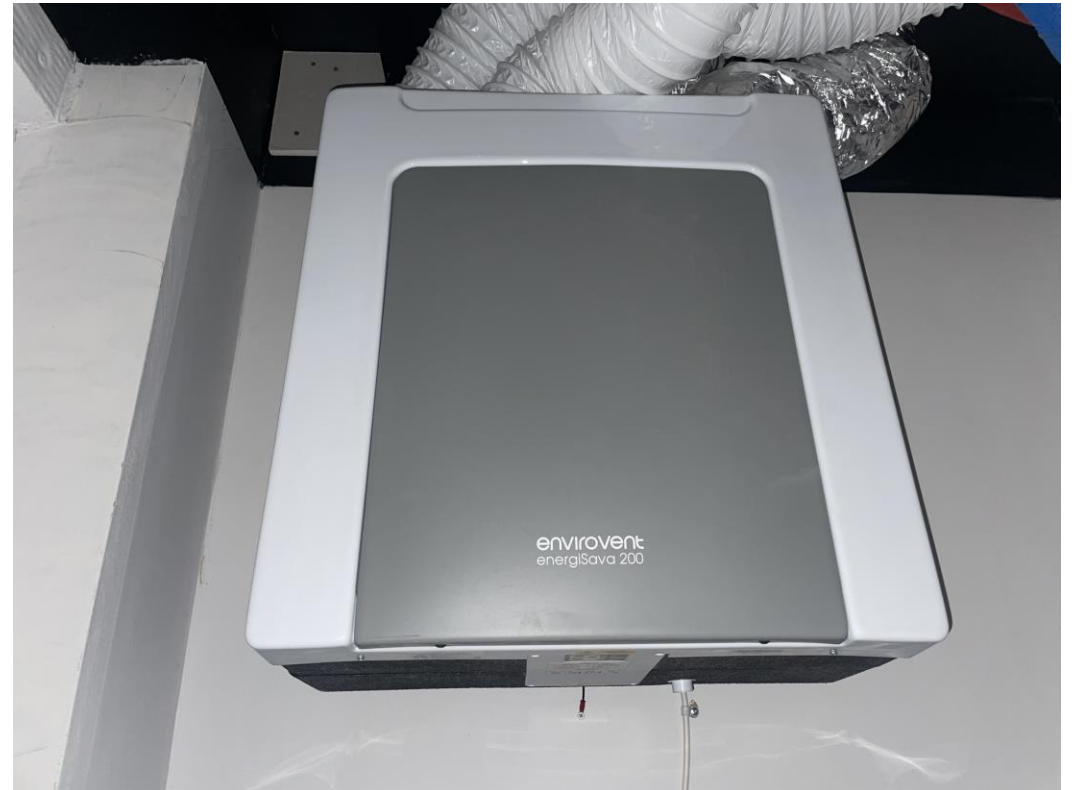
Level 6 – Mechanical appliances
