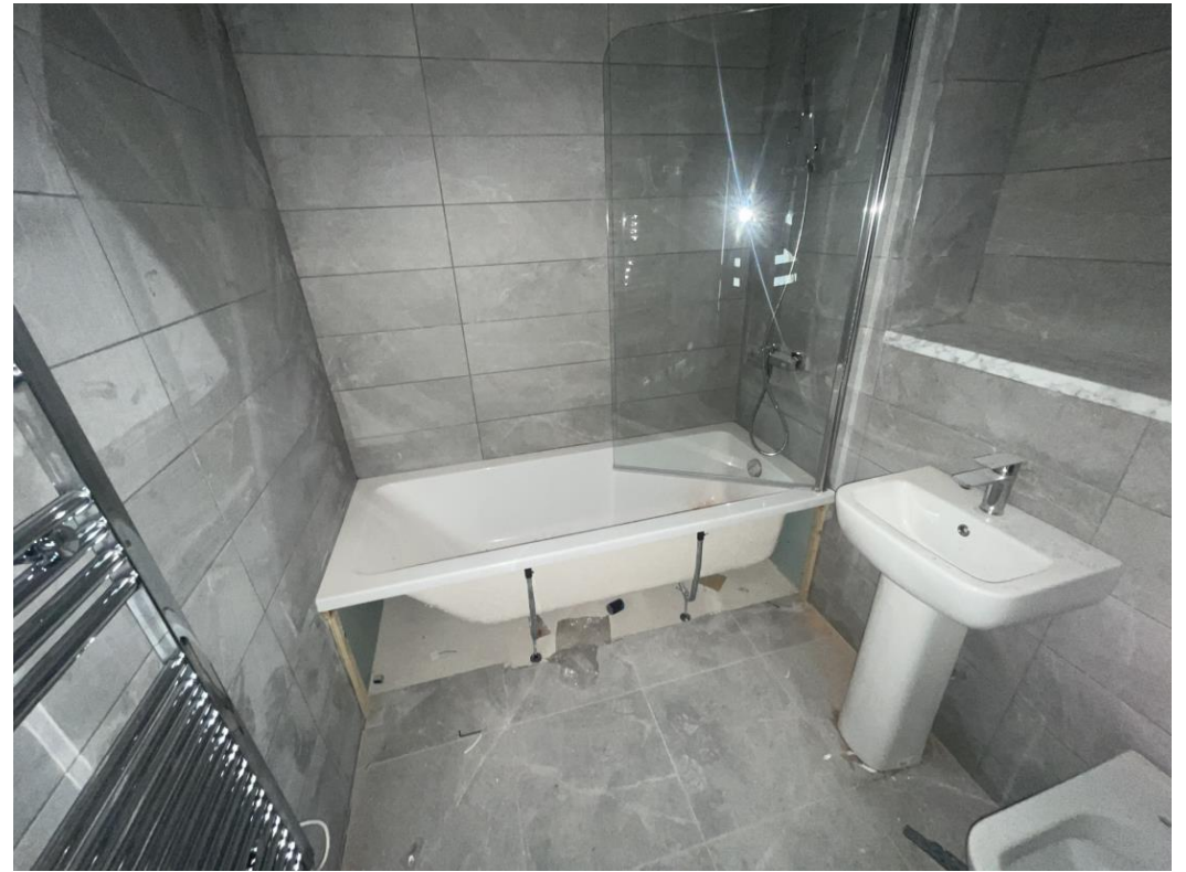
Level 8 – Bathroom sanitary appliances
