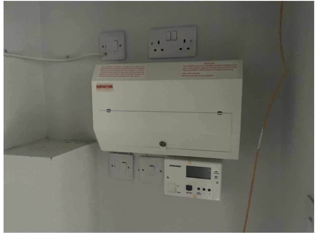
Level 6 – Electrical consumer unit
