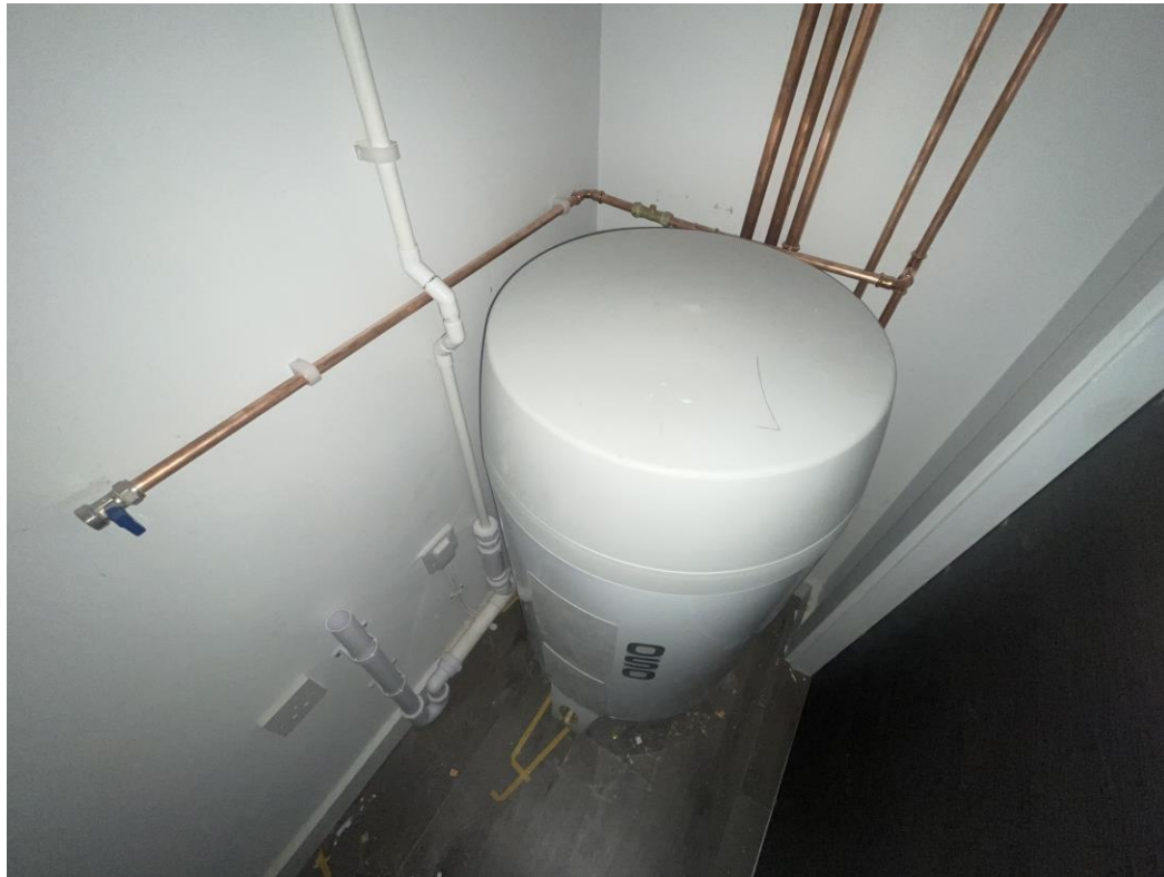
Level 2 – Mechanical appliances
