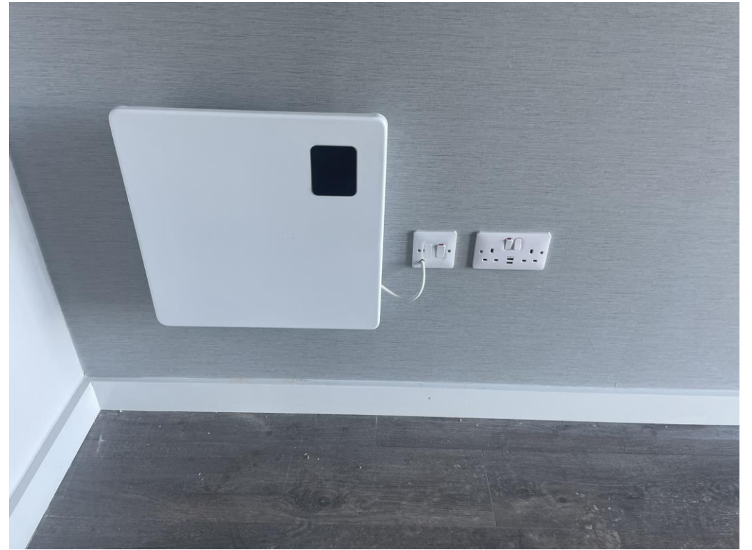
Level 1 – Wall panel heater
