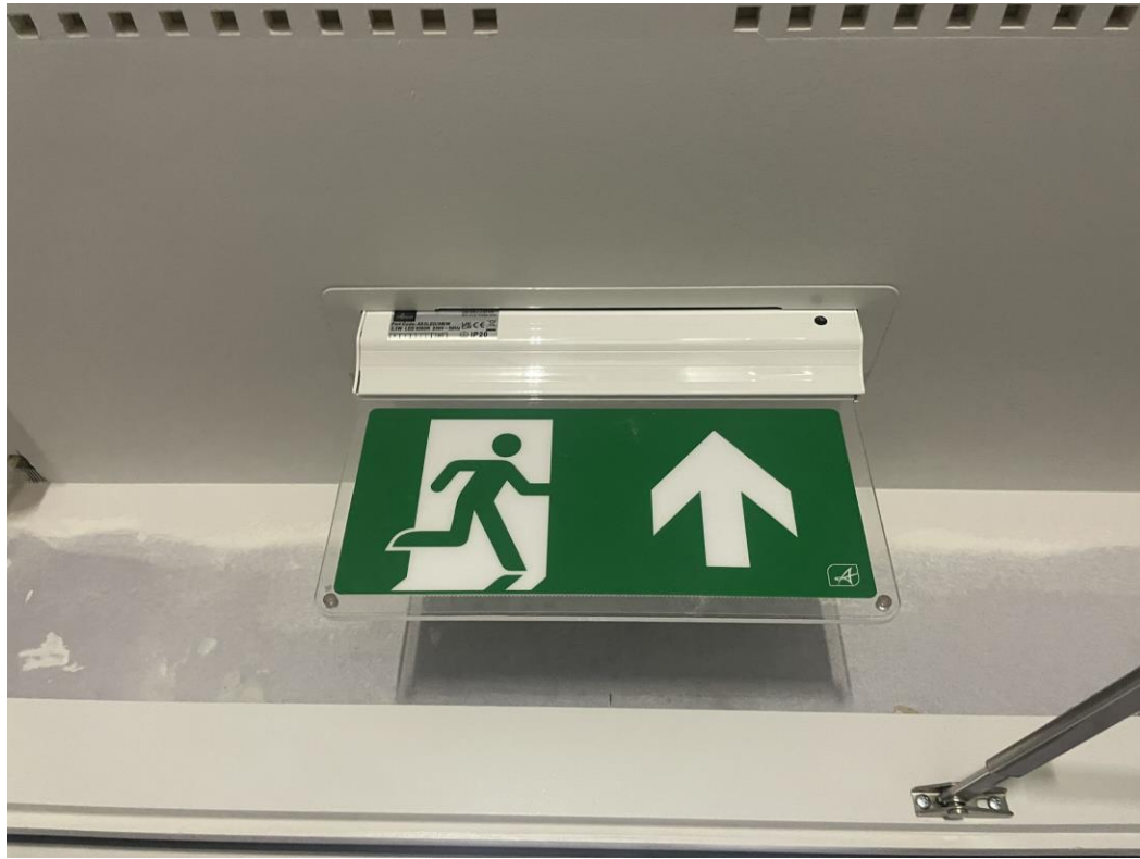
Level 6 – Way finding signage
