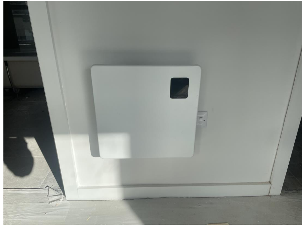
Level 4 – Wall panel heater
