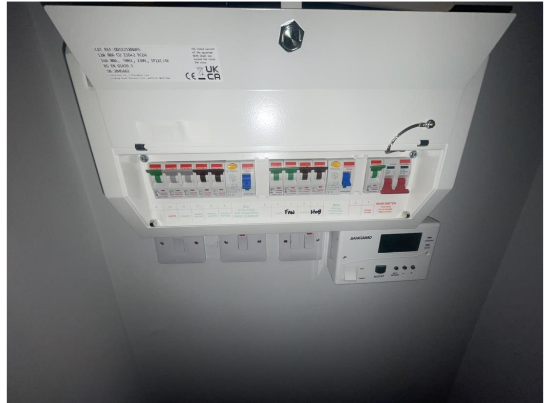
Level 2 – Electrical consumer unit
