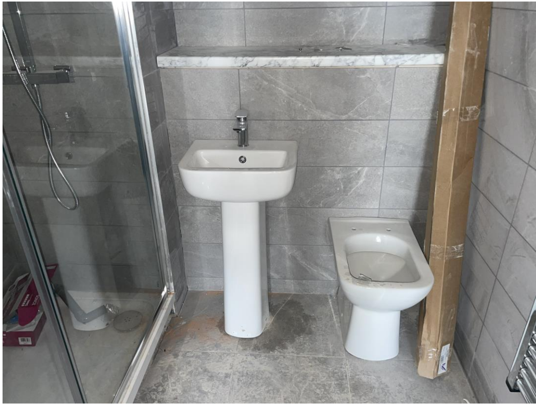
Level 8 – Bathroom sanitary appliances
