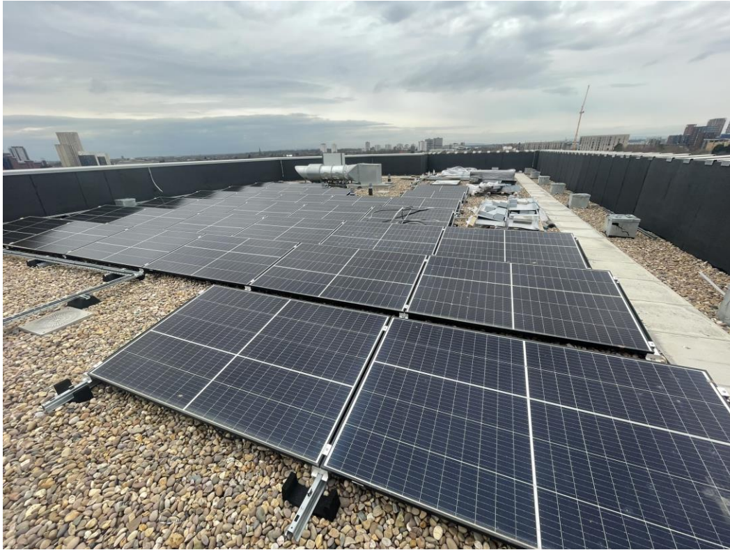
Block A – PV installed
