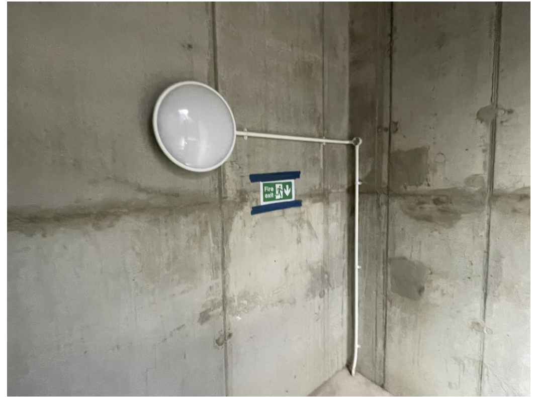
Level 6 - Stairwell lighting
