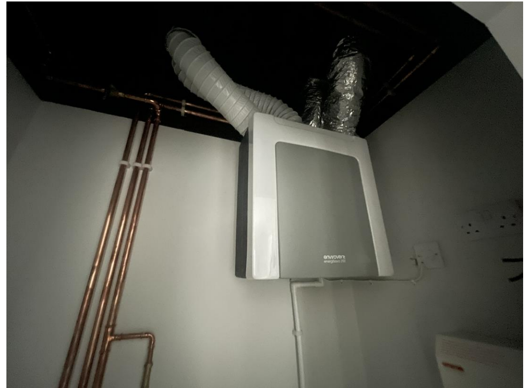
Level 1 – Mechanical appliances
