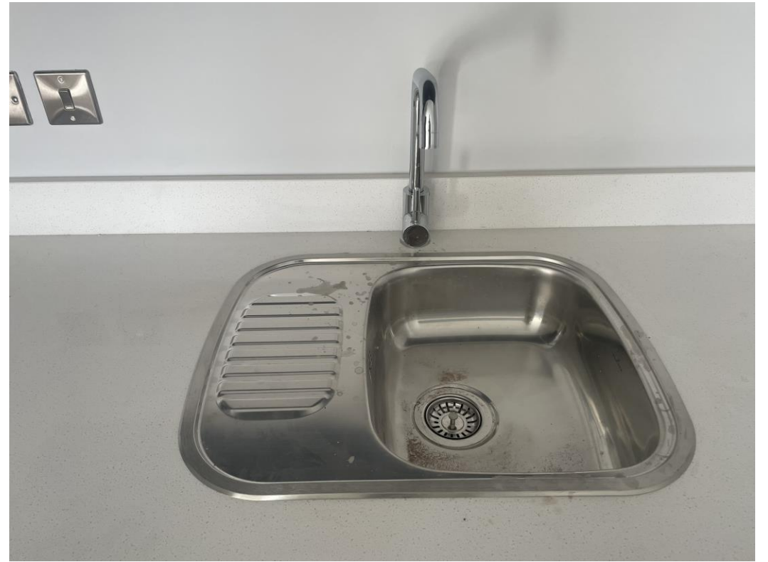
Level 6 – Kitchen sink and tap
