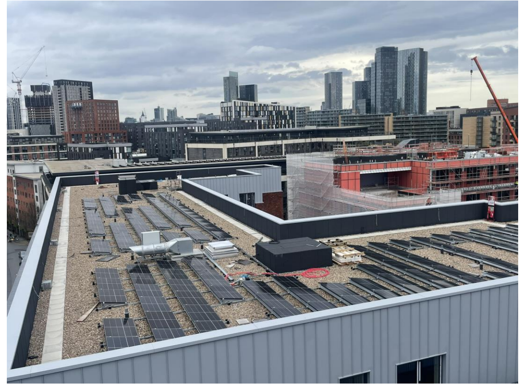
Block B – PV installed
