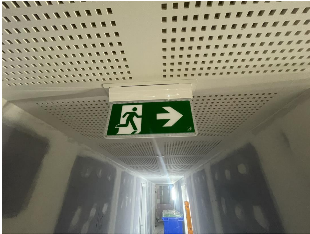
Level 4 – Way finding signage
