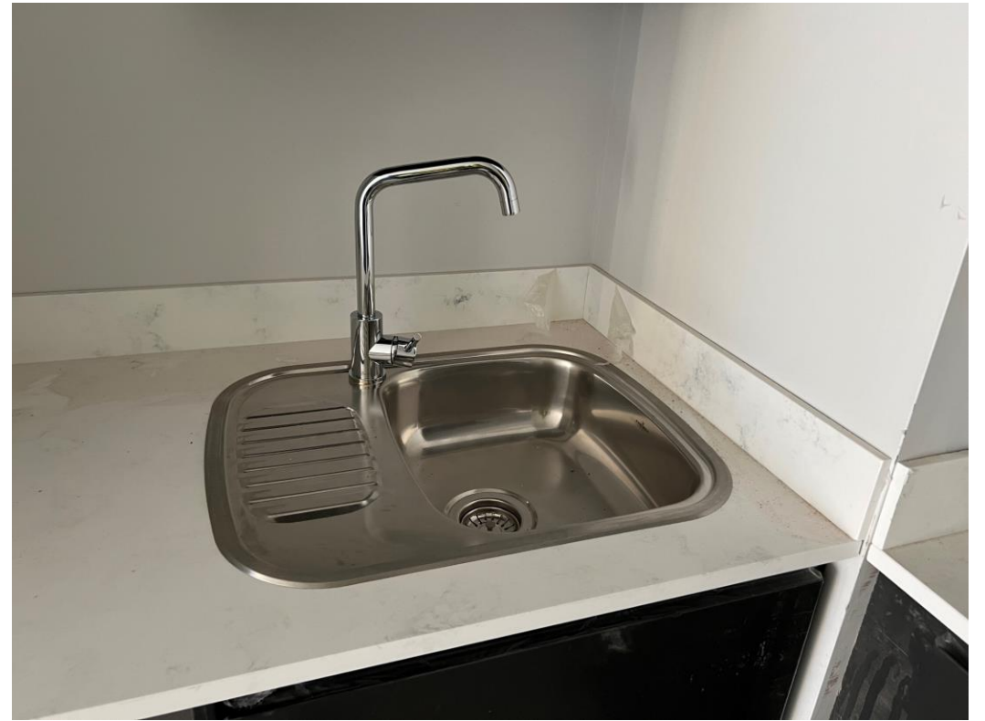
Level 5 – kitchen sink and tap
