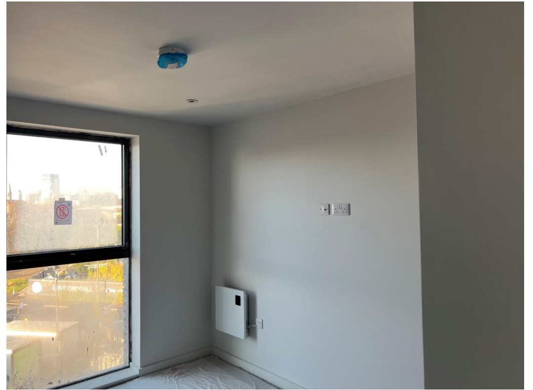
Level 4 – wall panel heating
