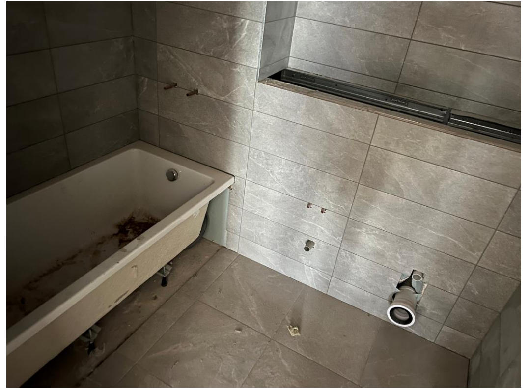
Ground Level - Sanitary fittings
