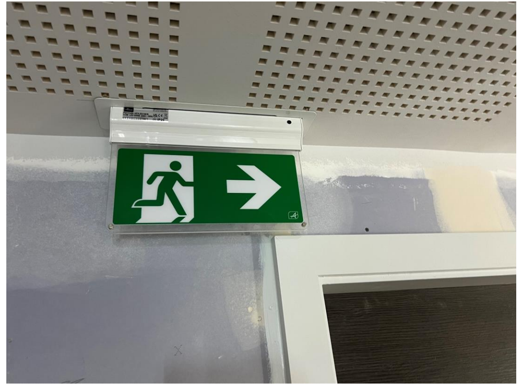
Level 6 – means of escape signage
