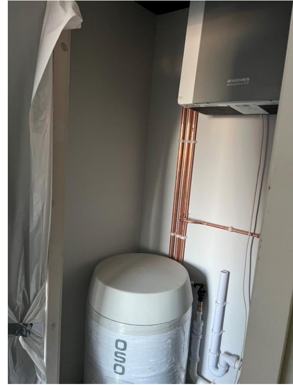
Level 8 – Mechanical appliances
