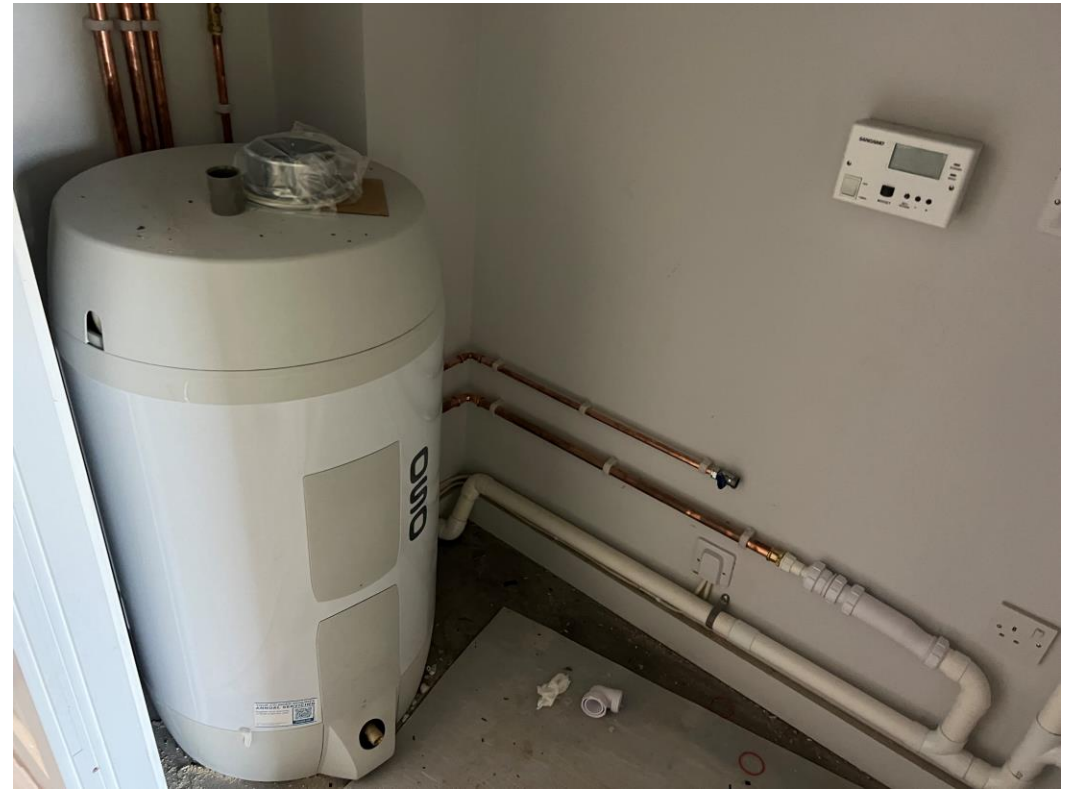
Level 2 – mechanical water heater
