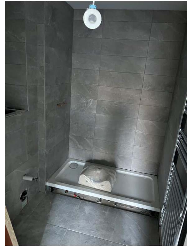
Level 1 – Sanitary fittings
