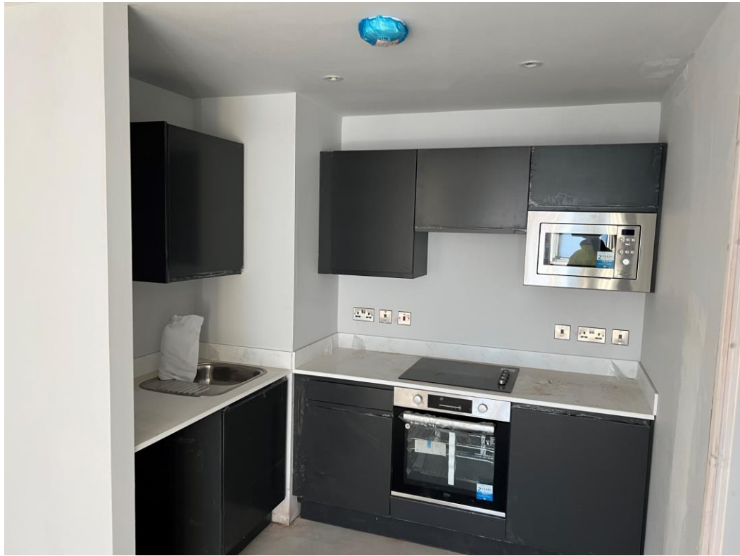
Level 5 – kitchen sink and tap
