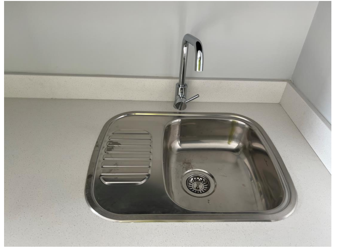
Level 6 – Kitchen sink installed
