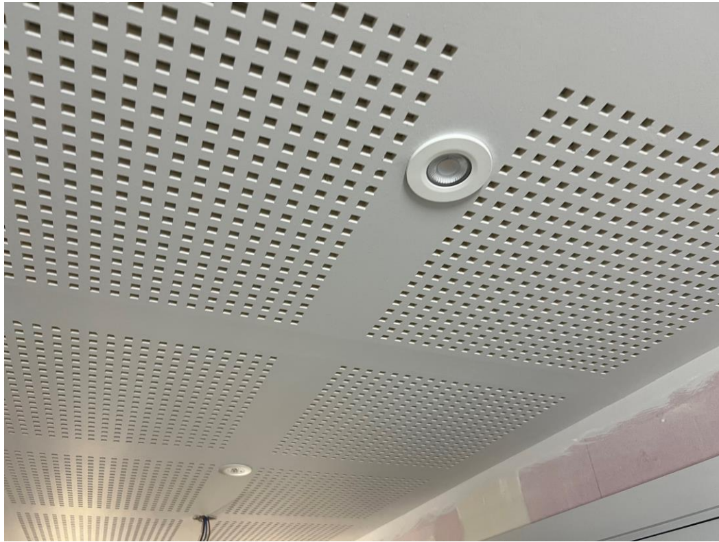
Level 6 – corridor lighting
