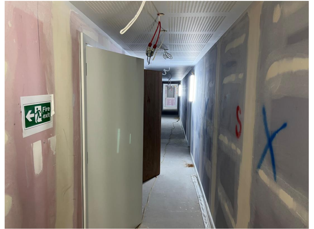
Level 6 – Fire doors to services cupboard
