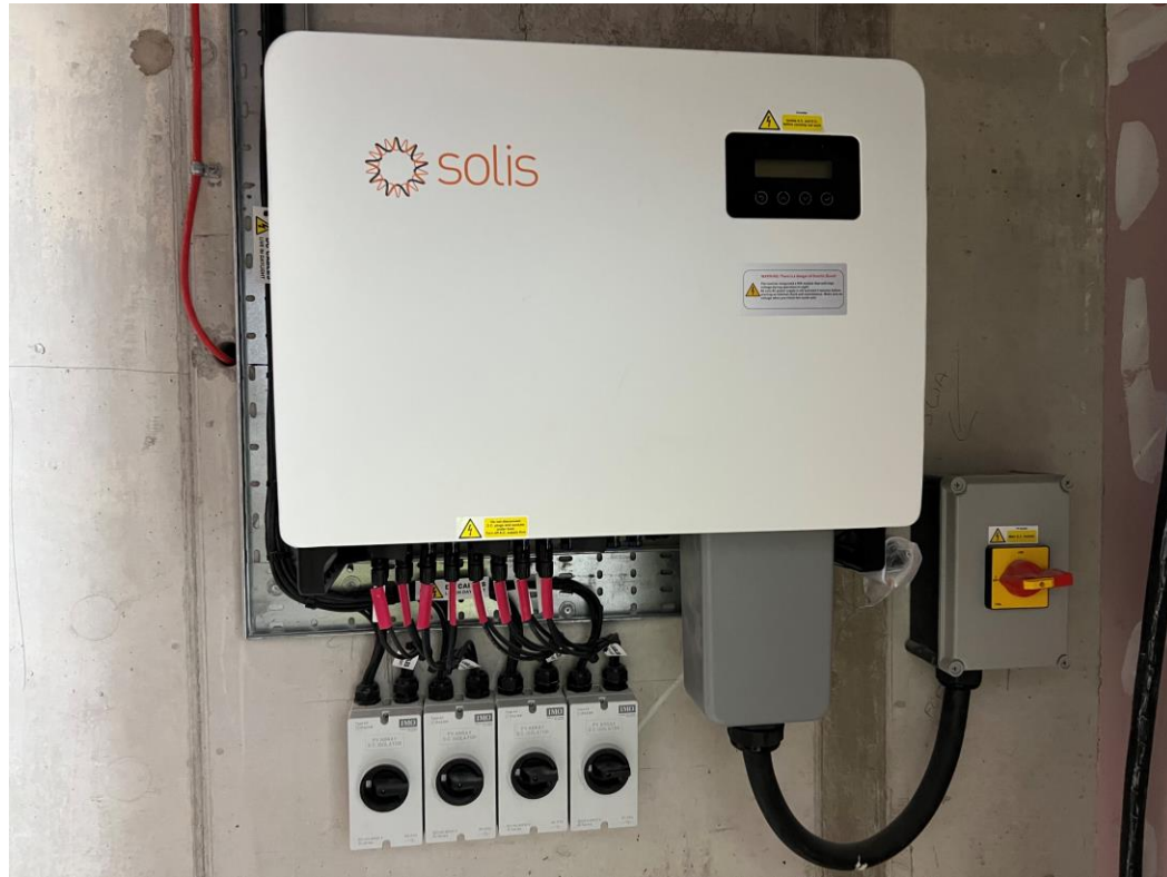
Level 6 – PV controls
