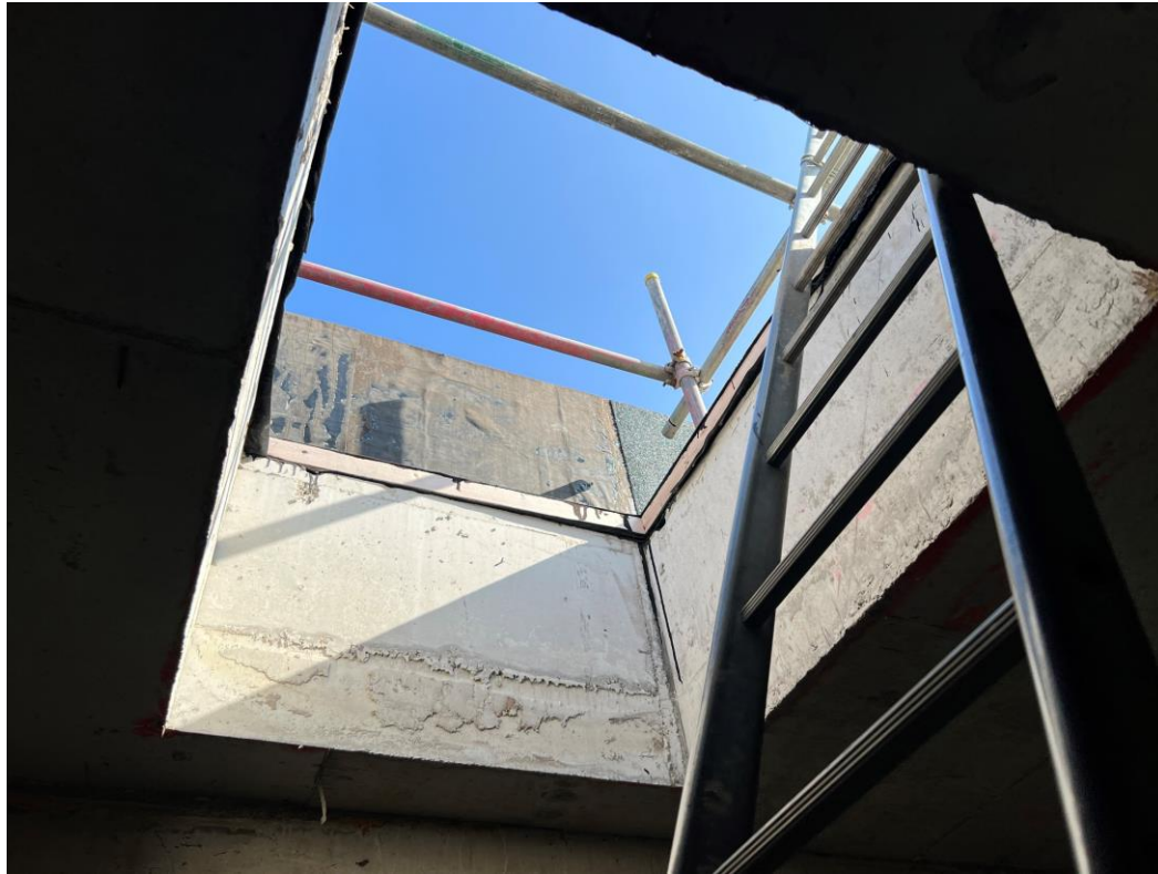
Level 8 – Smoke vent opening
