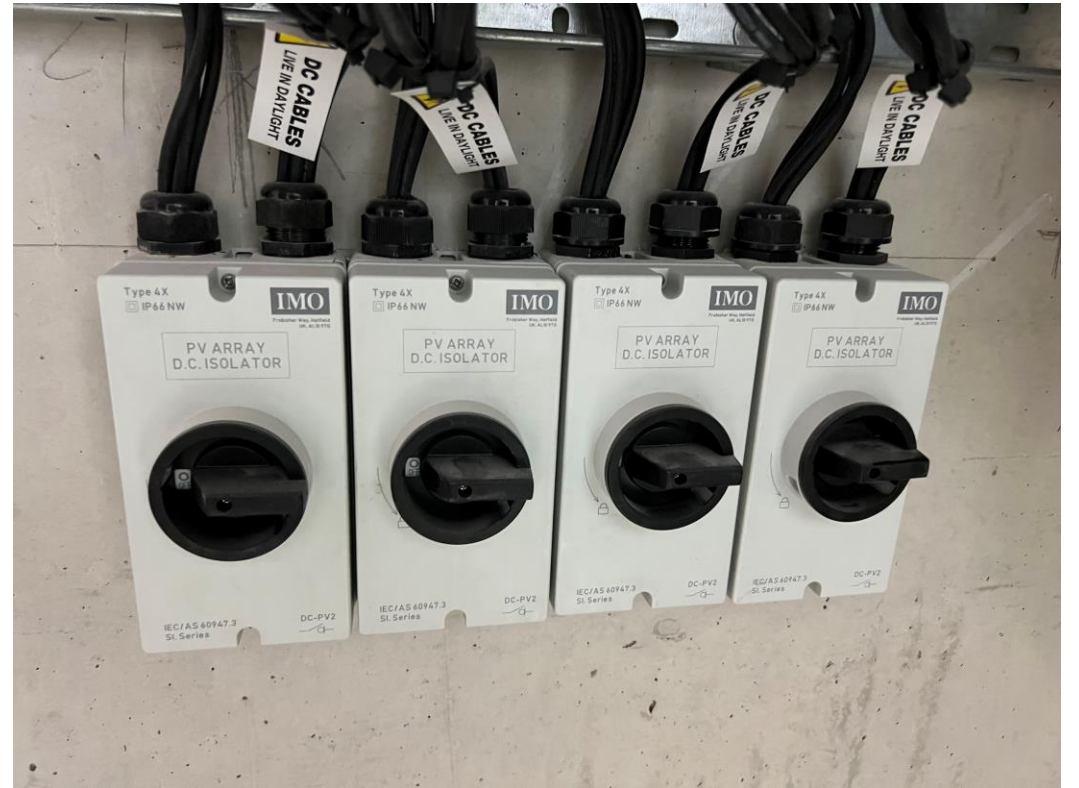
Level 6 – PV controls
