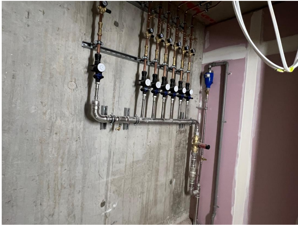
Level 6 – Water meter pipework
