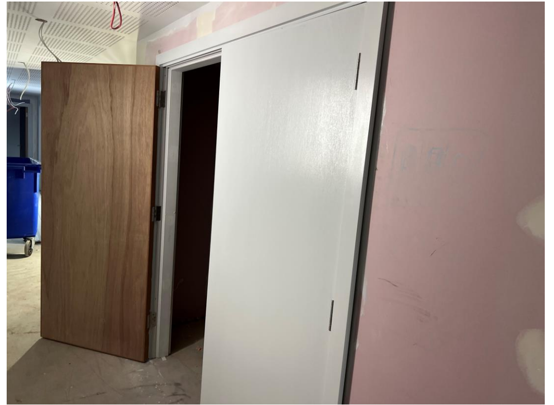
Level 6 – Fire doors to services cupboard
