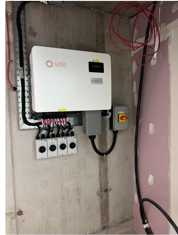
Level 6 – PV controls
