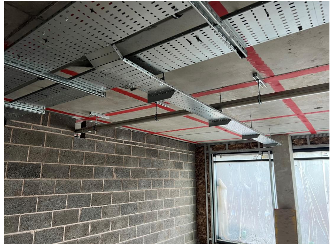
Ground Level – Electrical containment
