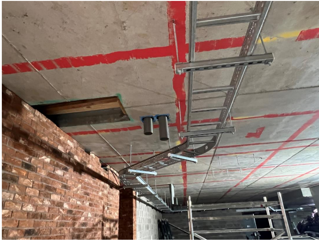
Ground Level – Electrical containment
