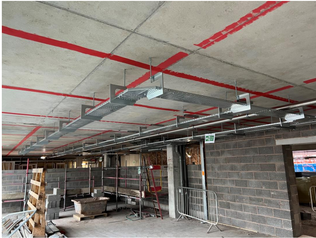
Ground Level – Electrical containment
