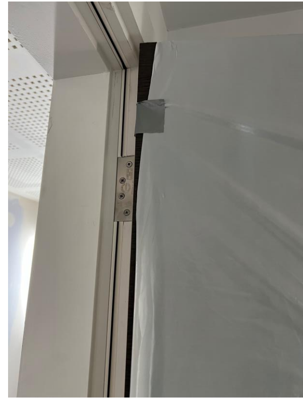
Level 6 – doorframe smoke seal
