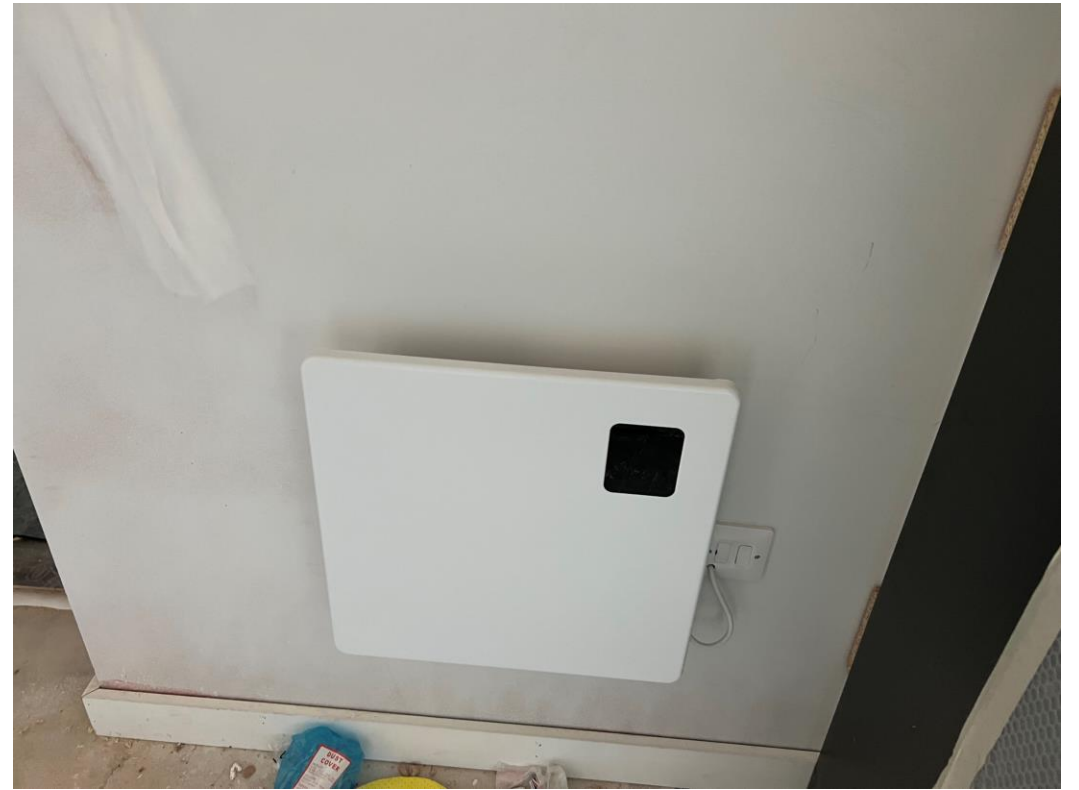
Level 6 – 2 nd fix electrical panel heater
