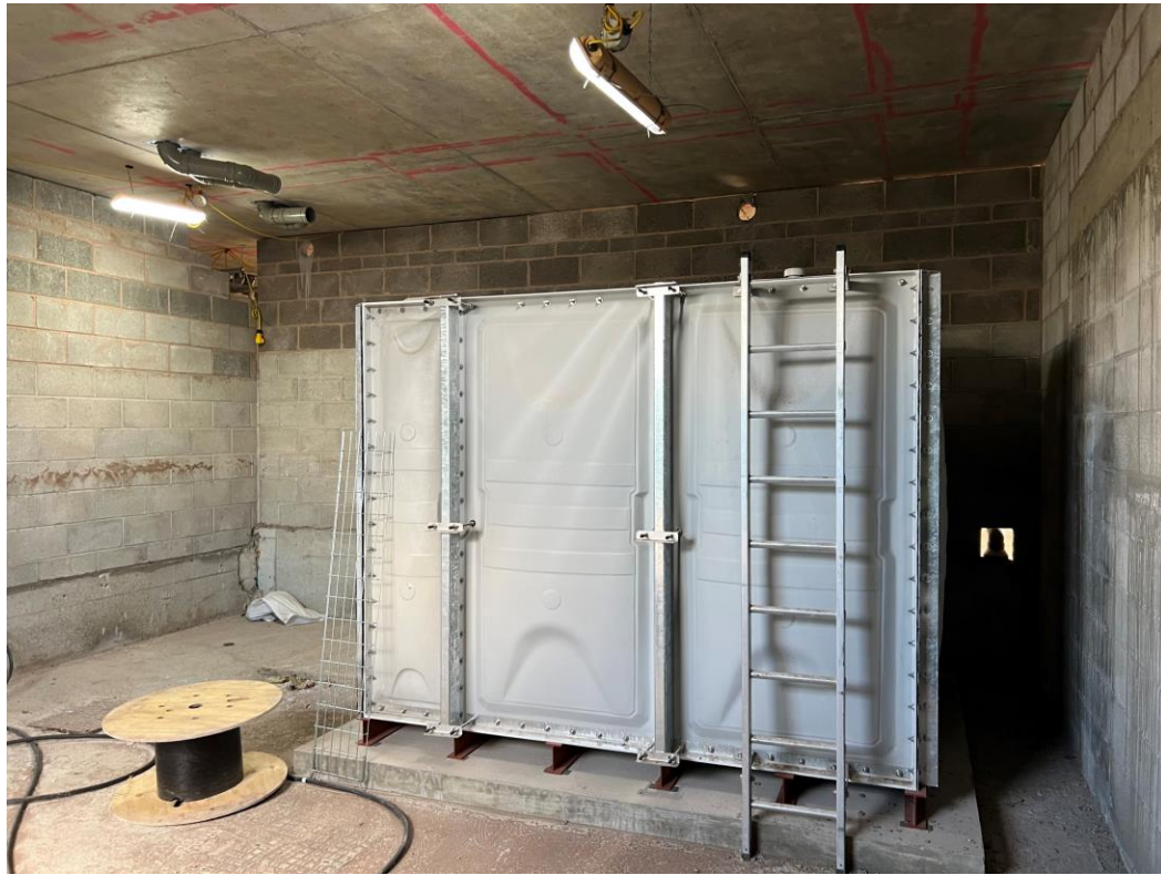
Ground Level – water storage tank
