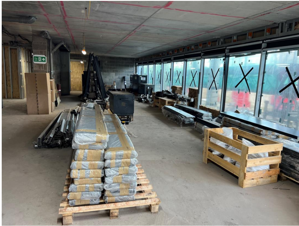
Ground Level – window and curtain walling materials stored
