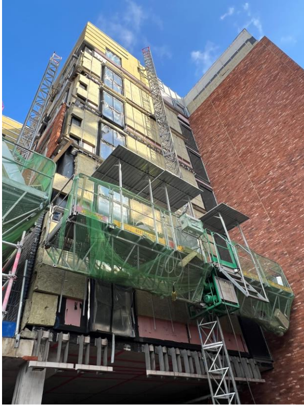
Block B brick anchor support
