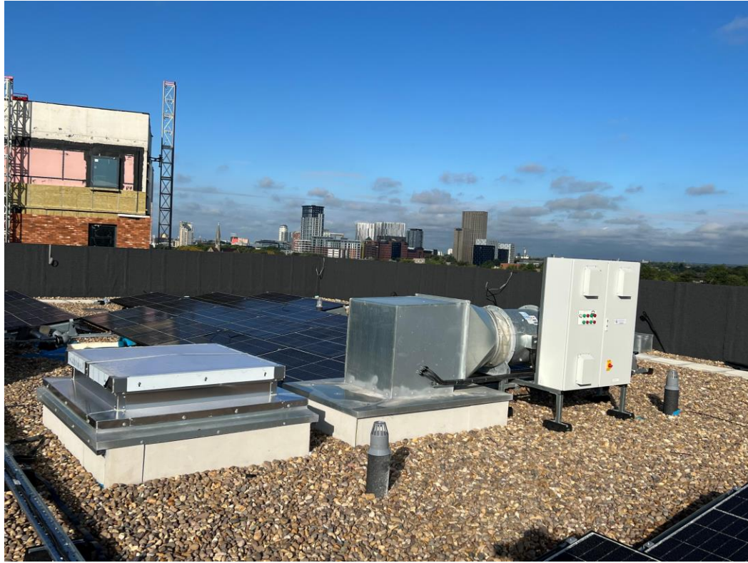
Block B AO and ventilator unit
