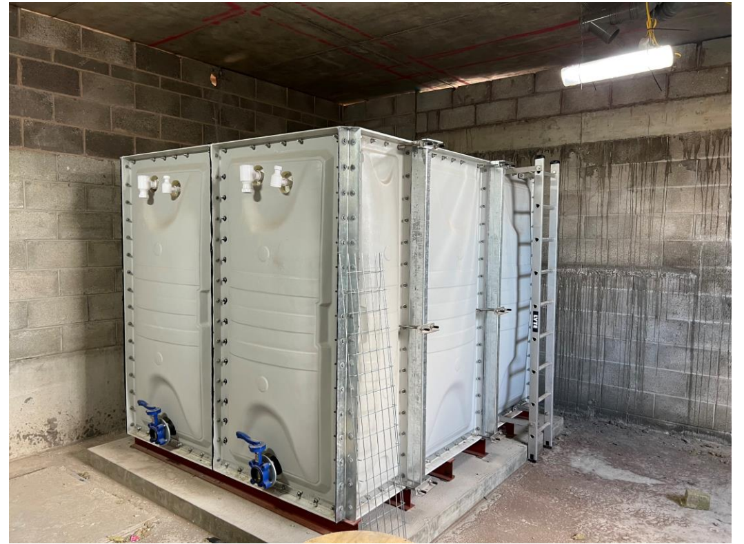
Ground Level – water storage tank
