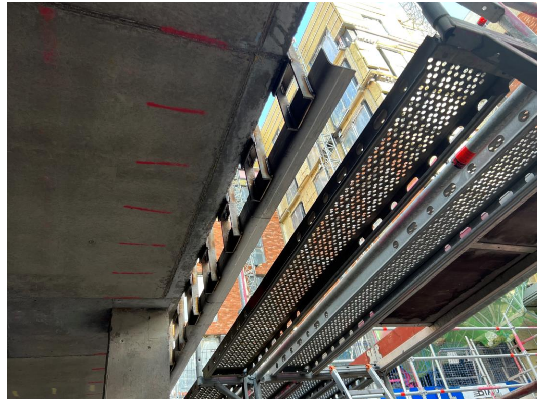
Block B brick anchor support
