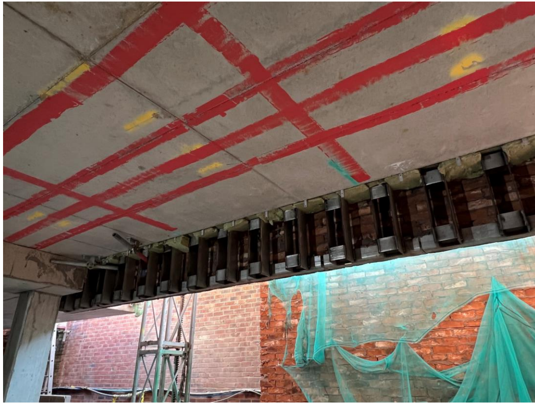
Block B brick anchor support
