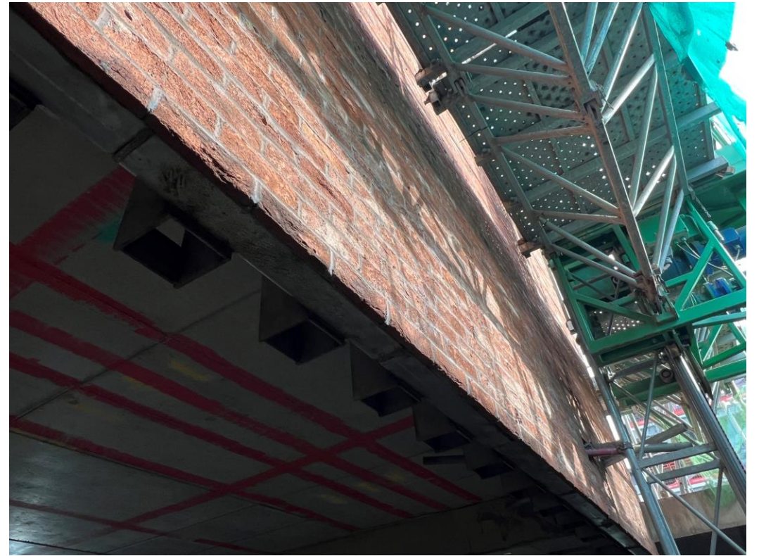
Block B brick anchor support
