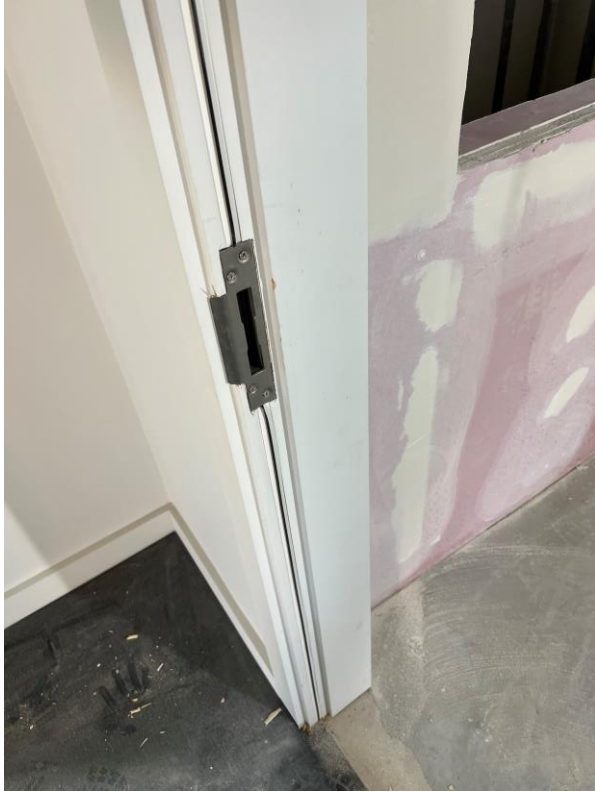
Level 6 – doorframe smoke seal
