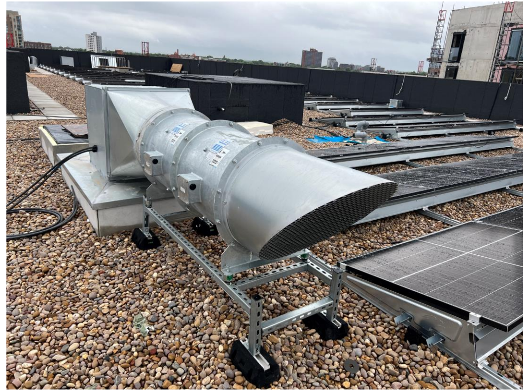
Block B ventilator unit
