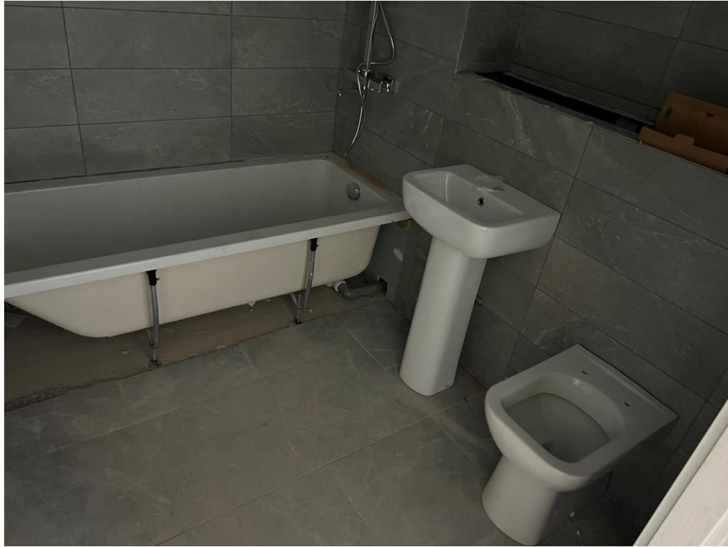
Level 3 – sanitary fittings
