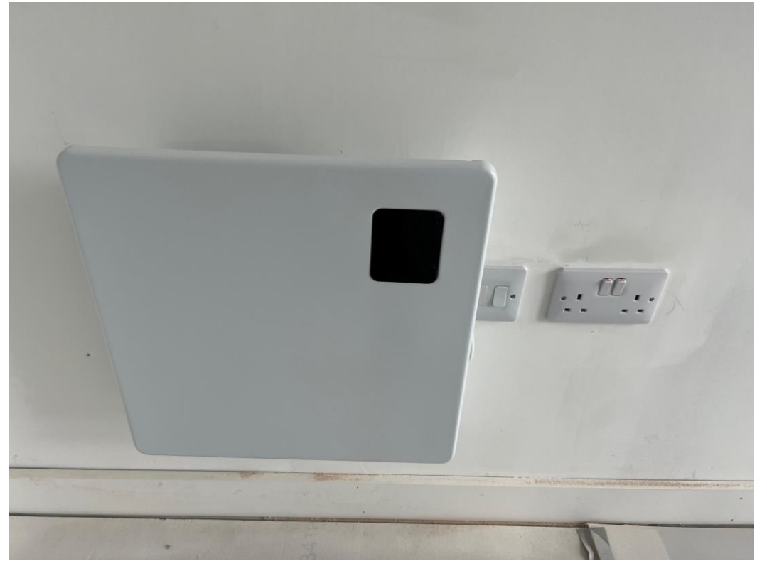
Level 2 – electric wall heater
