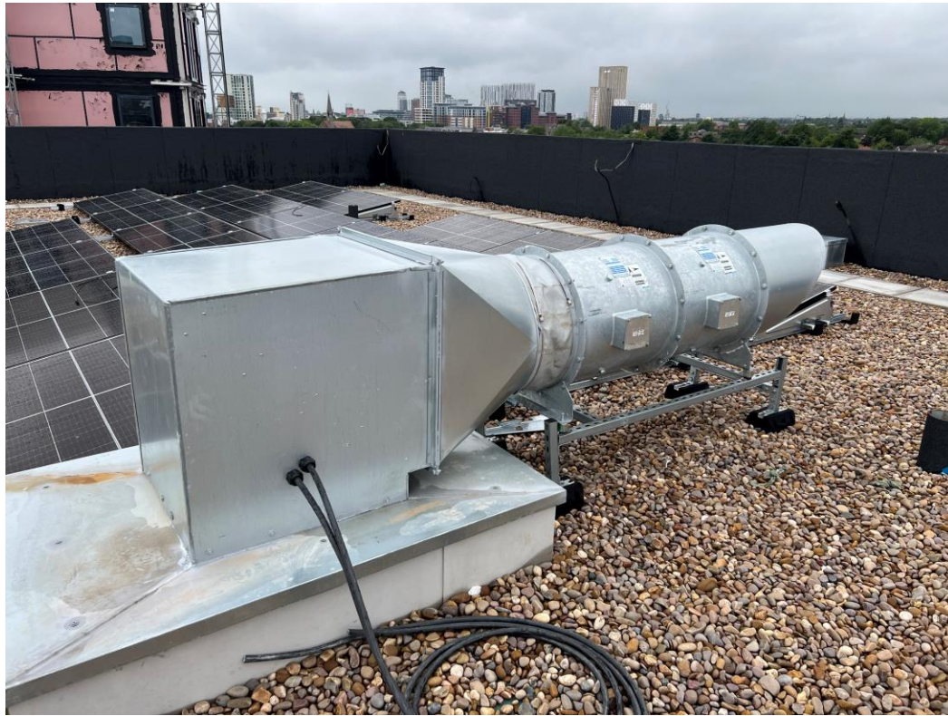
Block B ventilator unit
