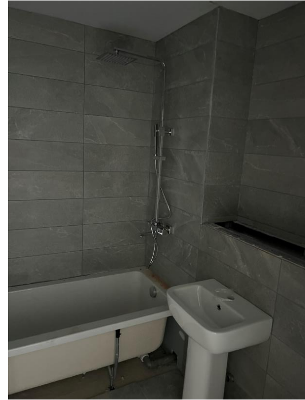
Level 3 – sanitary fittings
