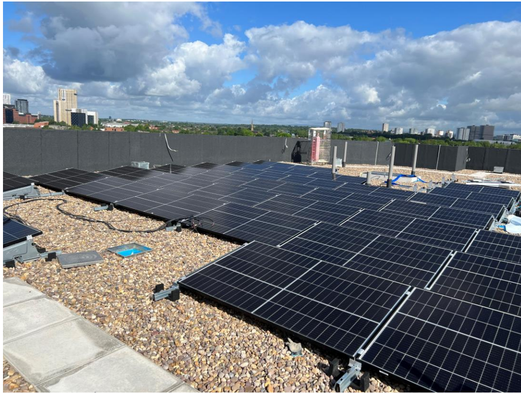
Block A PV panels installed
