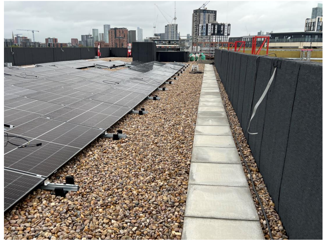
Block B PV solar panels
