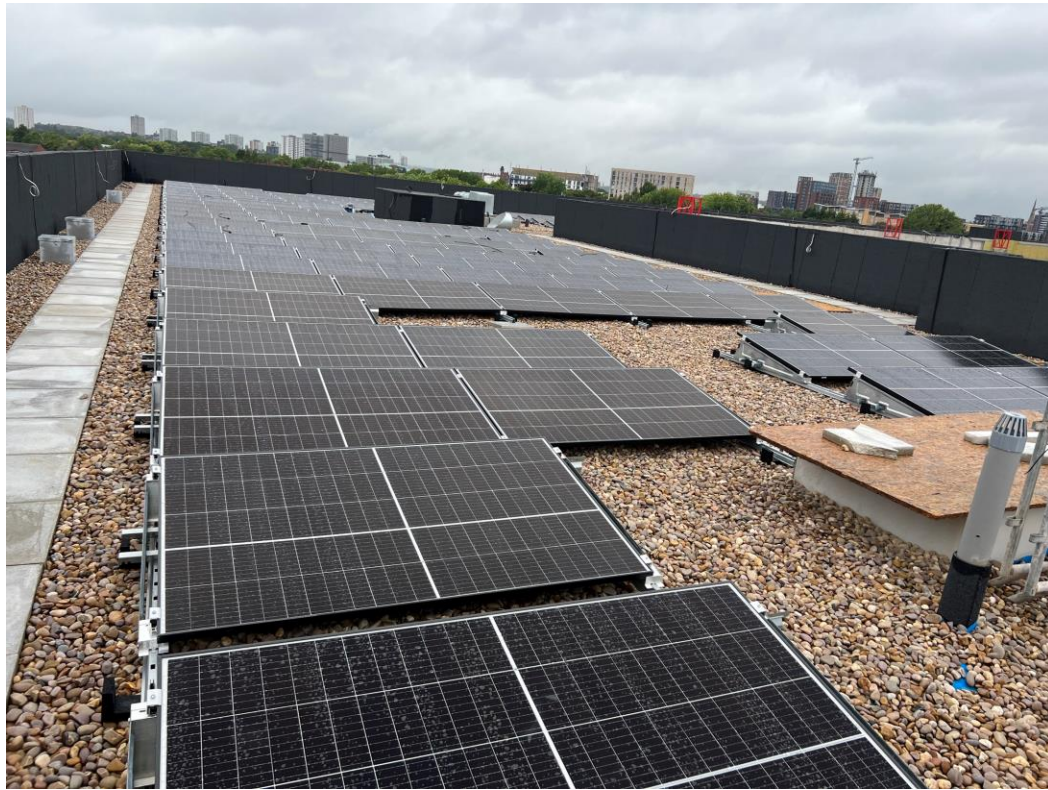
Block B PV solar panels
