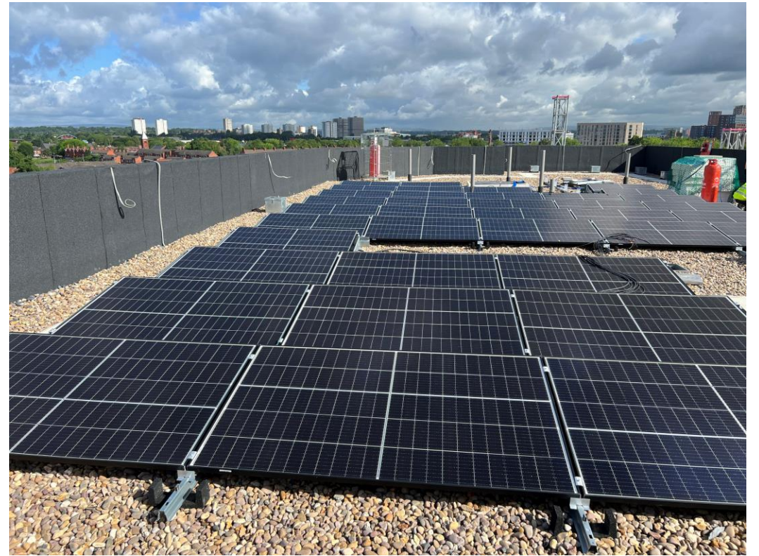
Block A PV panels installed
