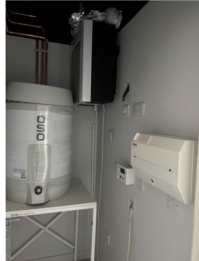
Level 2 – electric wall heater
