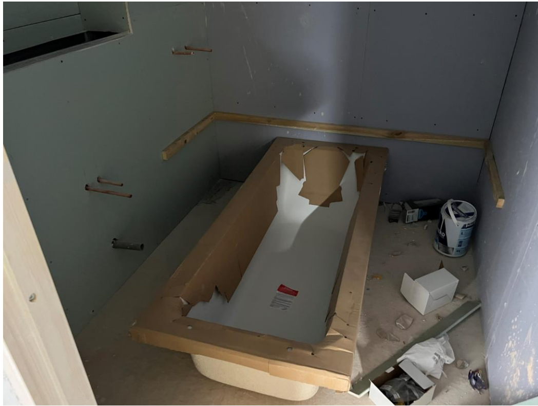
Level 6 – Sanitary installation
