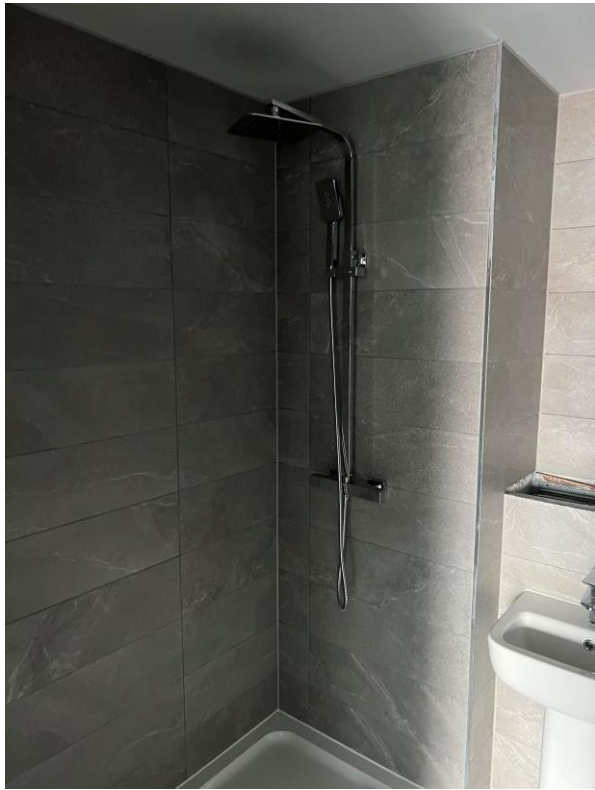
Level 1 – sanitary fittings
