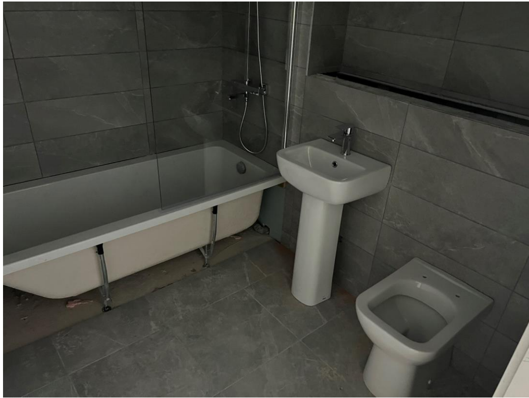
Level 1 – sanitary fittings
