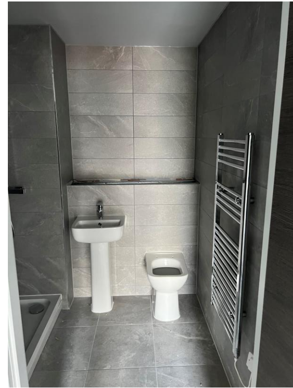
Level 1 – sanitary fittings
