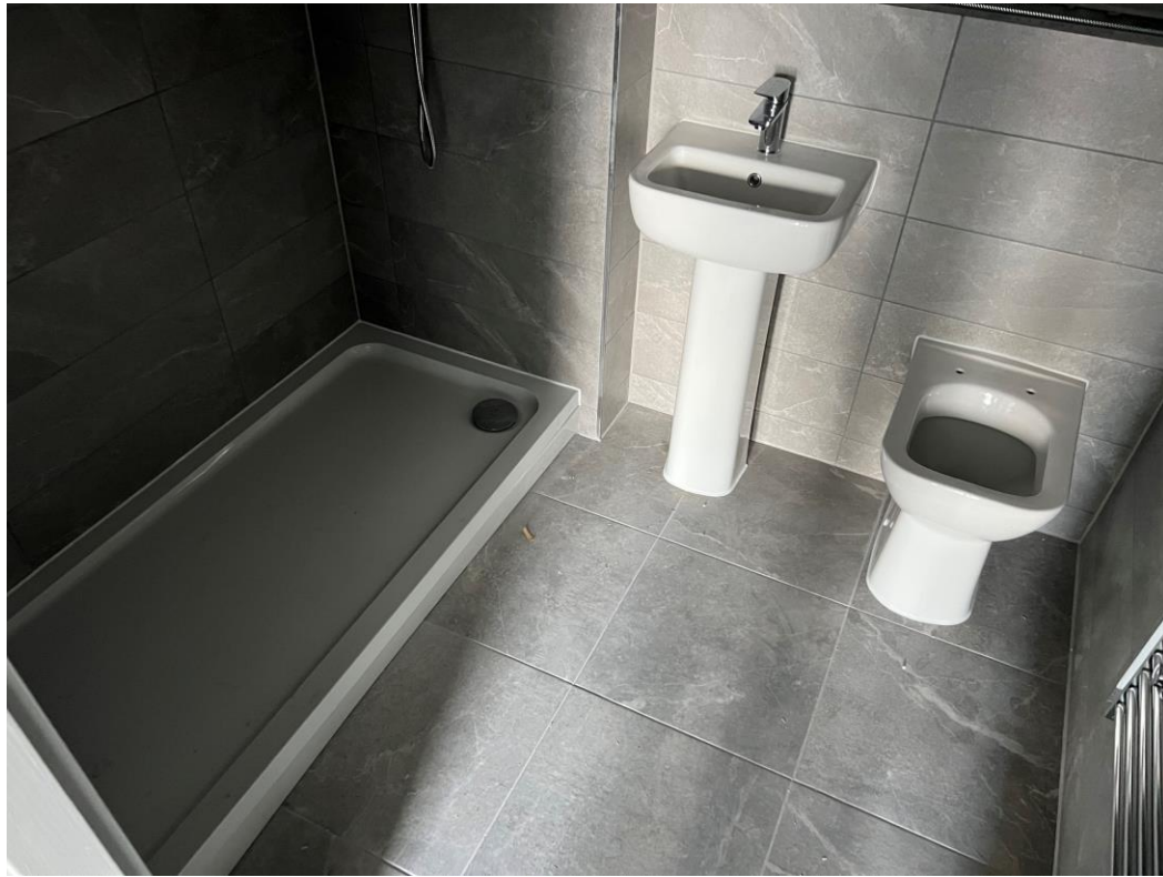
Level 1 – sanitary fittings
