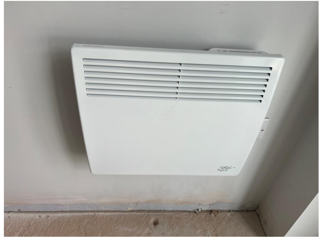
Level 3 – Electric wall heater
