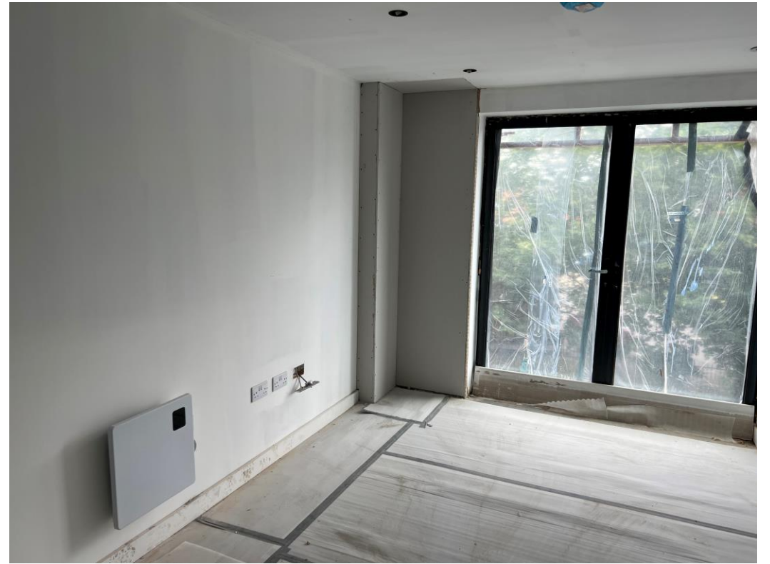
Level 2 – electric wall heater
