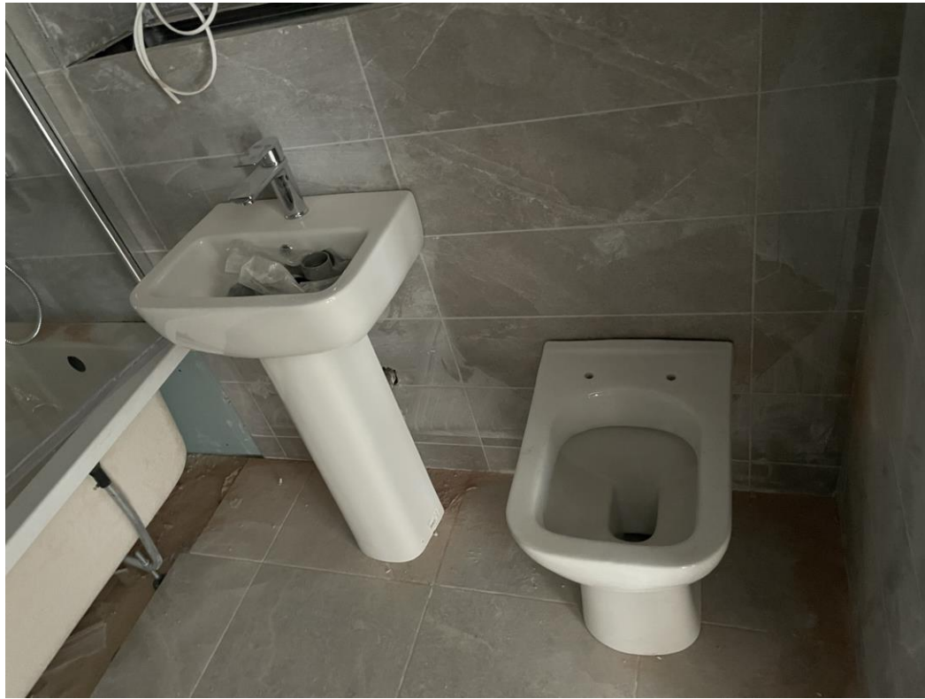
Level 2 – sanitary fittings
