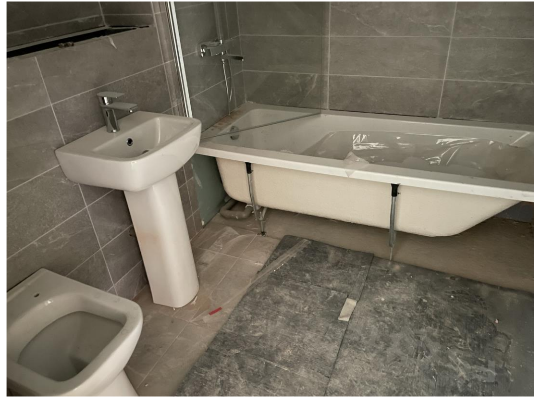
Level 2 – sanitary fittings
