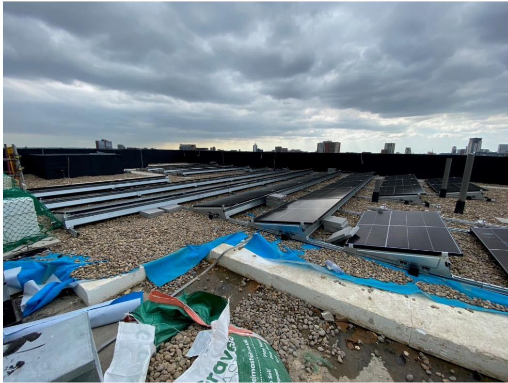
Block A PV panels installed
