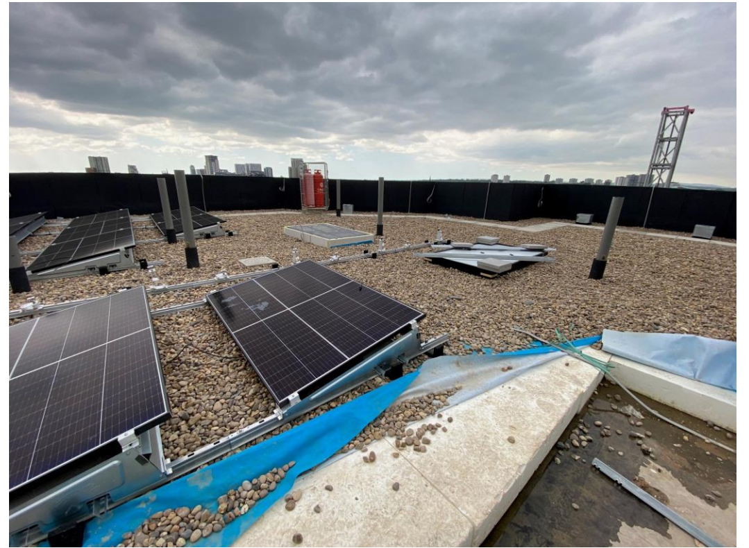
Block A PV panels installed
