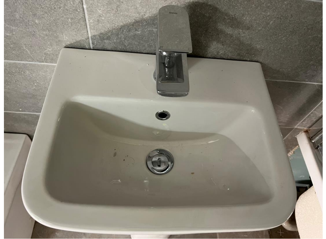
Sanitary fittings installed
