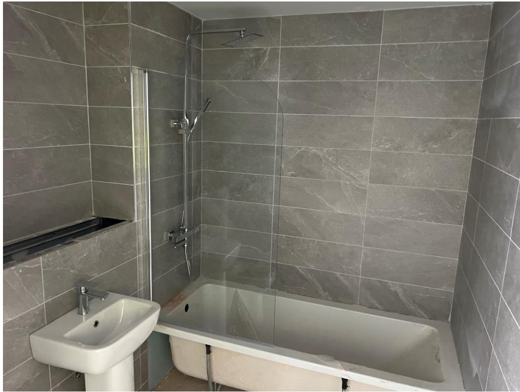
Sanitary fittings installed
