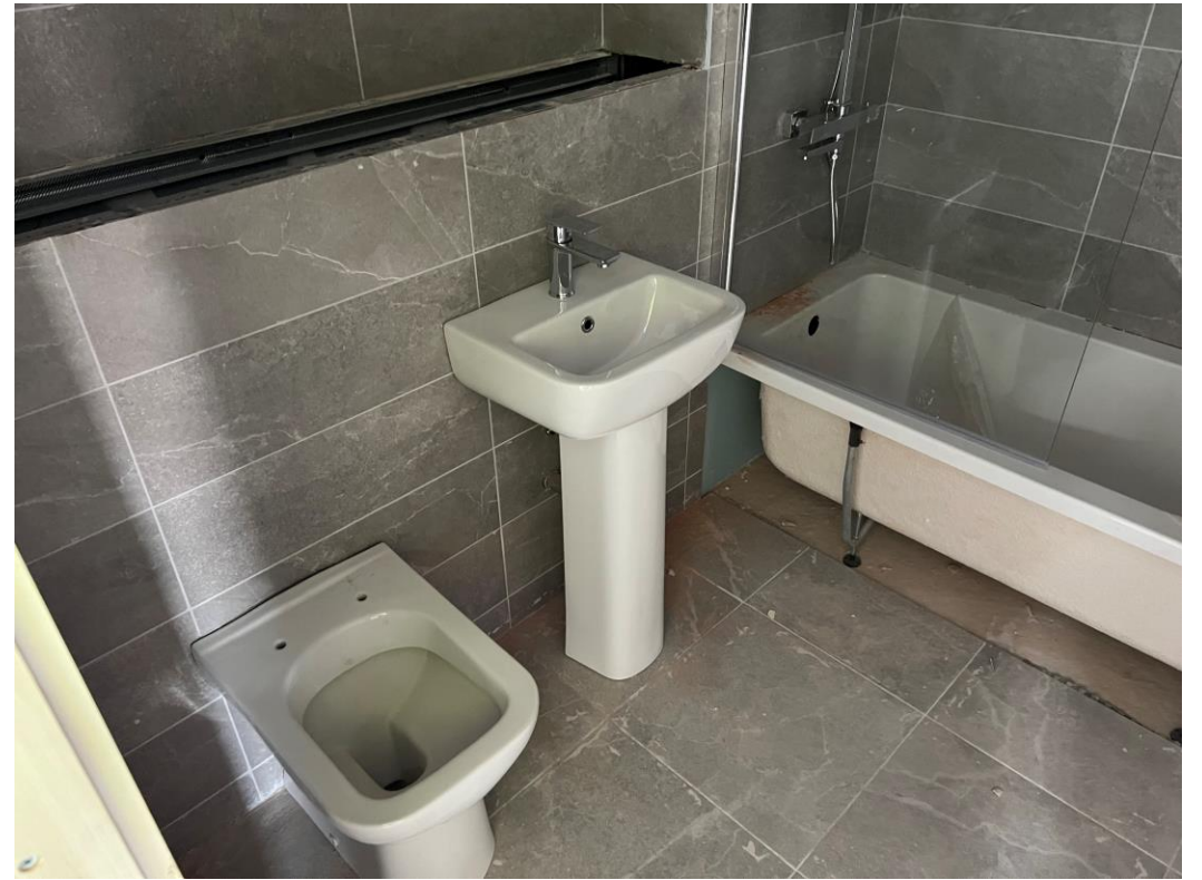
Sanitary fittings installed
