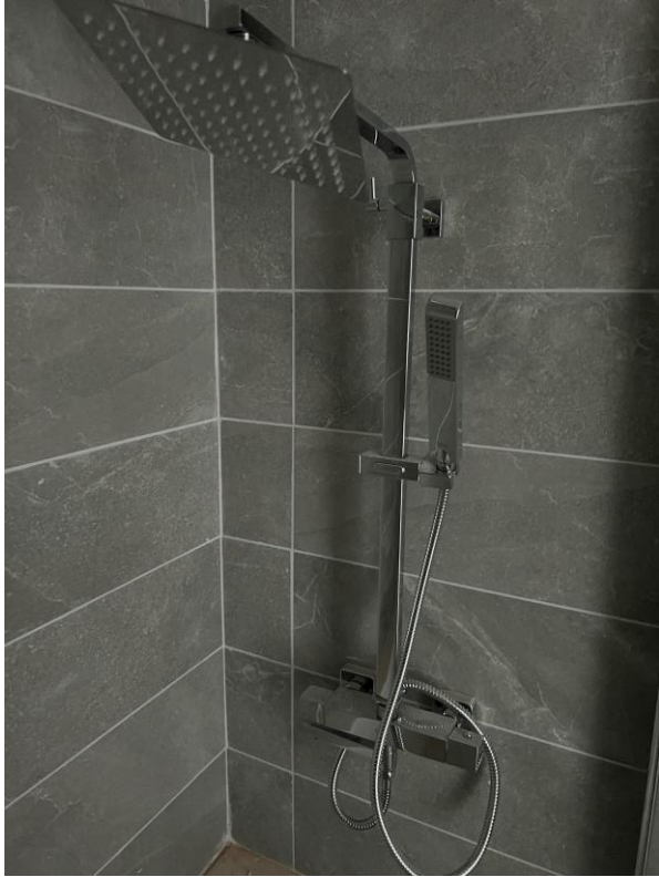
Sanitary fittings installed
