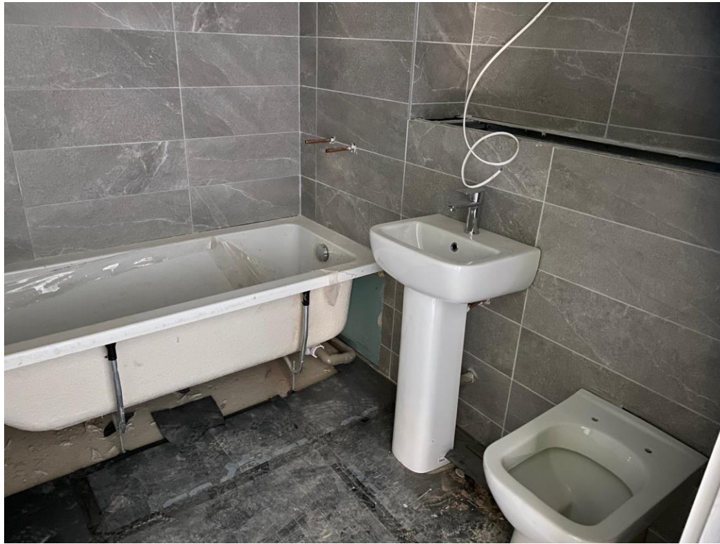
Sanitary fittings installed
