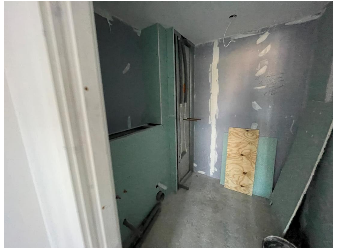
Apartment 1 st fix sanitary
