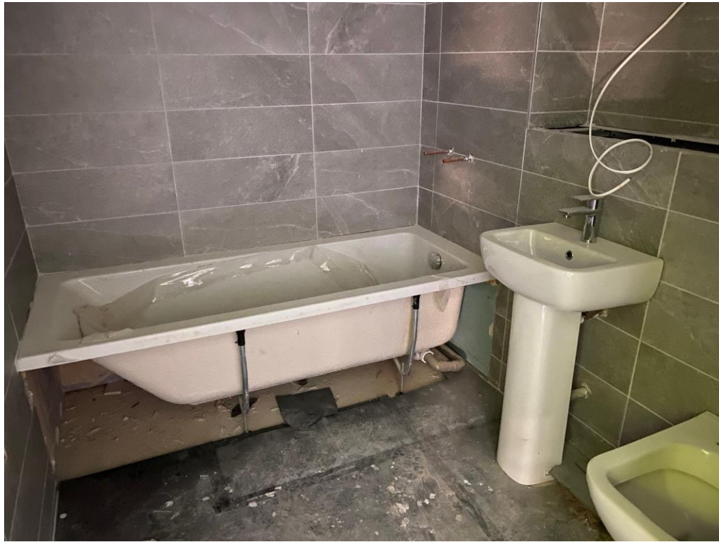
Sanitary fittings installed
