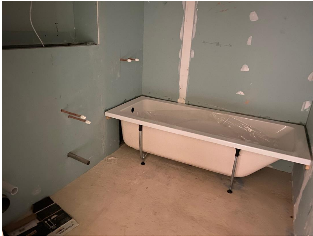
Apartment 1 st fix sanitary
