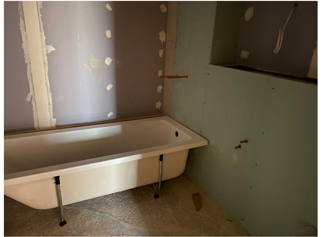
Apartment 1 st fix sanitary
