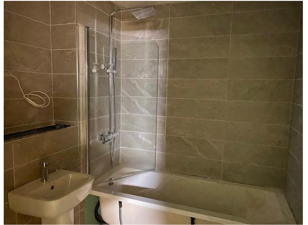
Sanitary fittings installed
