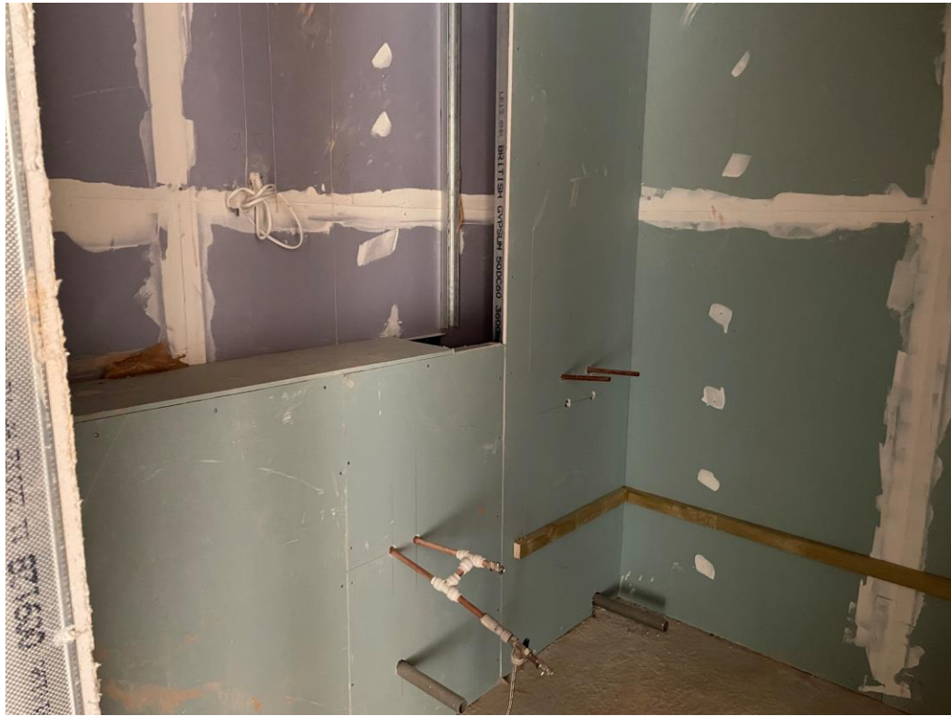
Apartment 1 st fix sanitary
