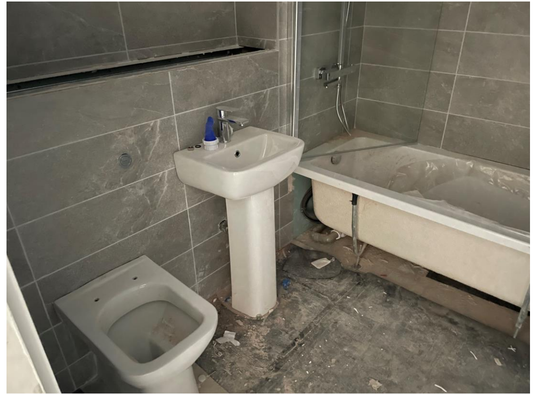
Sanitary fittings installed
