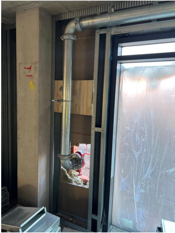
Dry riser to stairwell
