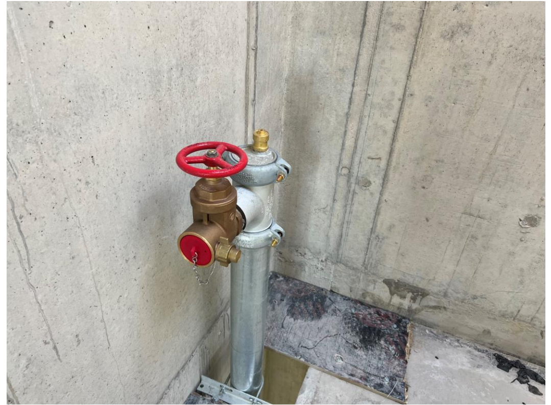
Dry riser to stairwell
