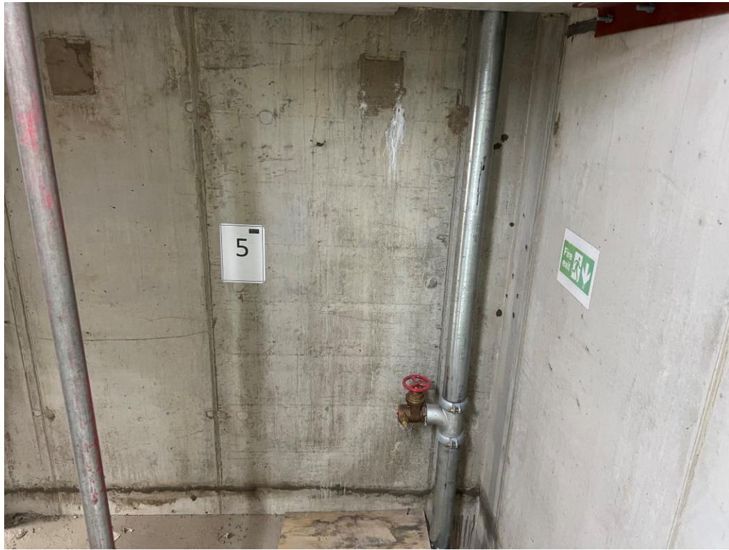
Dry riser to stairwell
