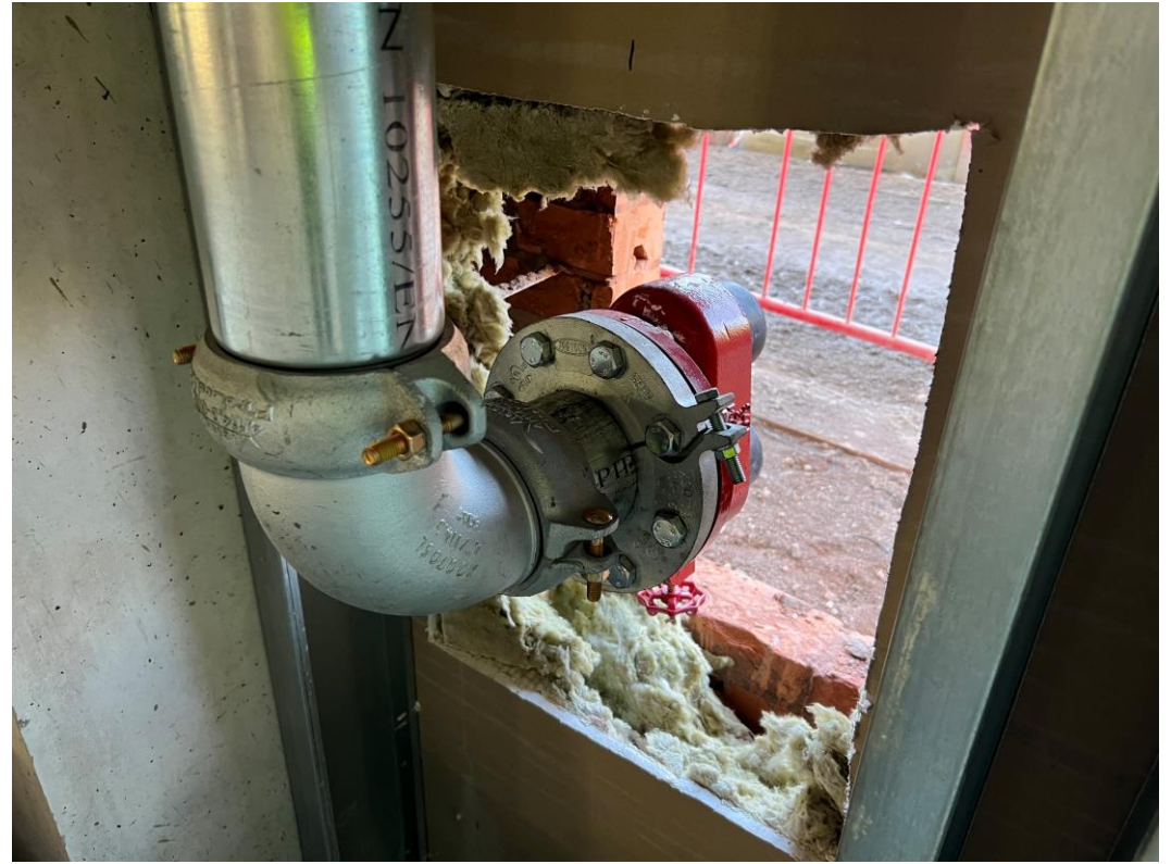
Dry riser to stairwell
