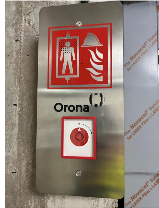
Fire Fighting Lift installed
