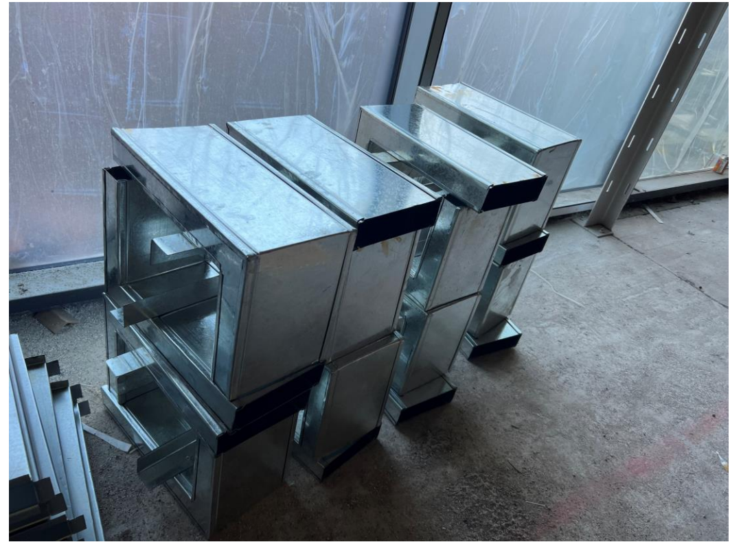
External vent duct plenum materials
