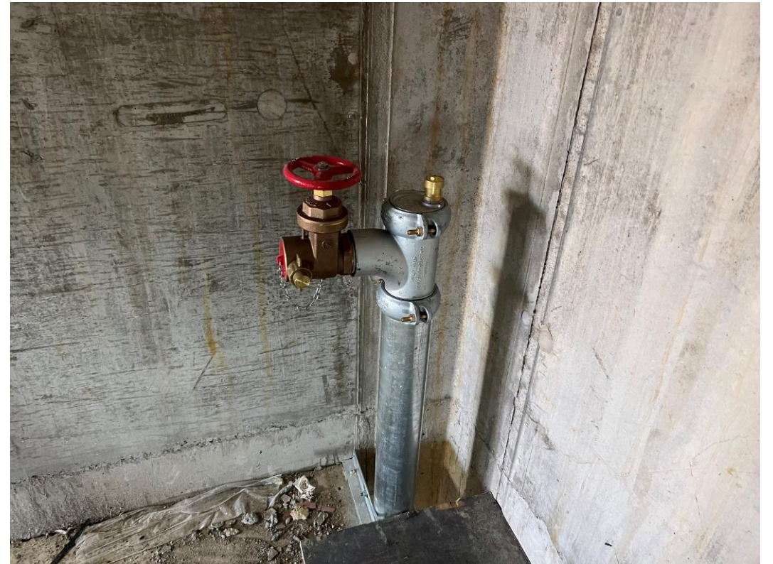
Dry riser to stairwell
