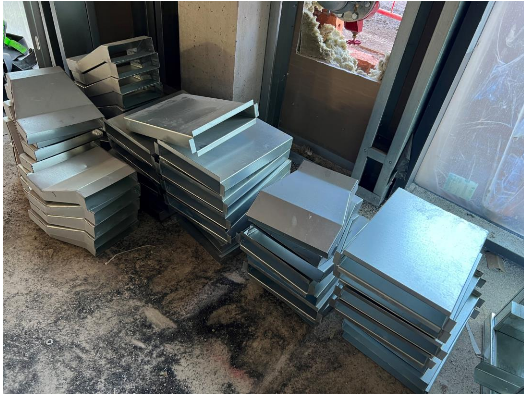
External vent duct plenum materials
