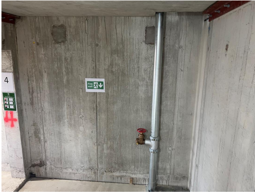
Dry riser to stairwell
