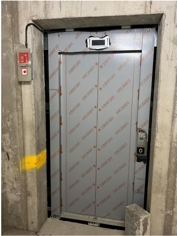
Fire Fighting Lift installed
