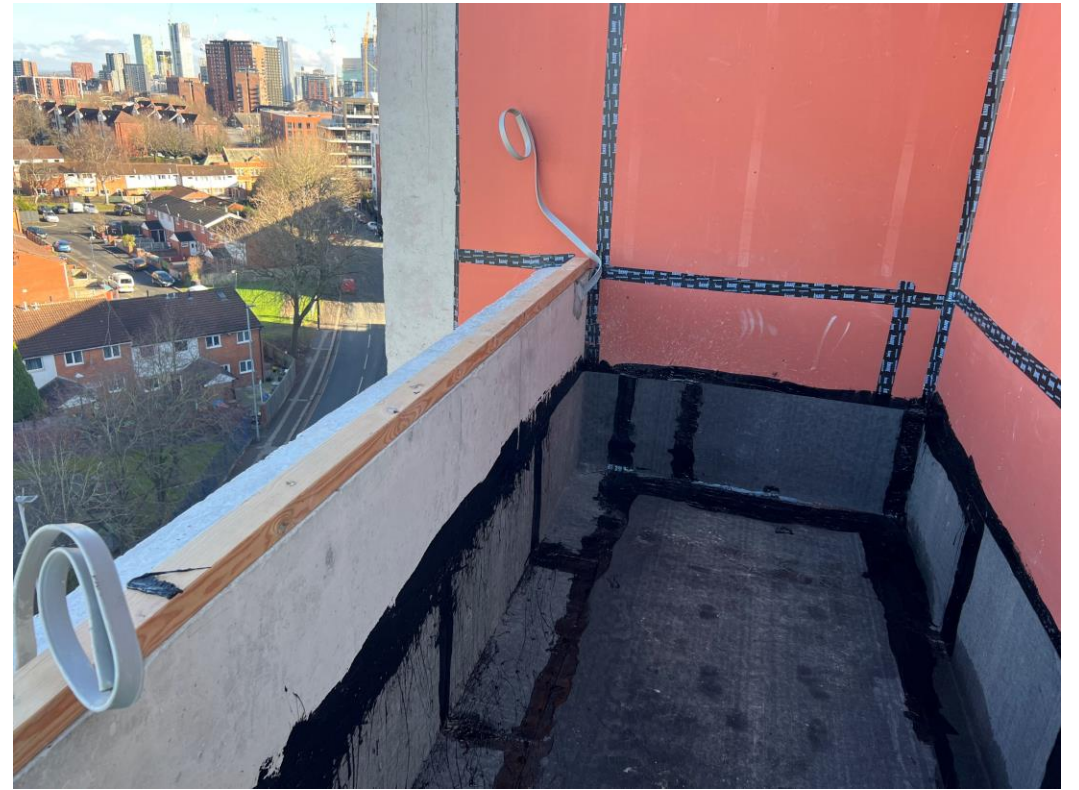
Block A lightning tape
