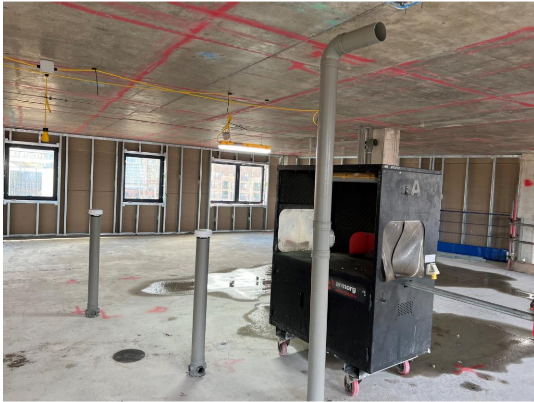
Upper level drainage pipework
