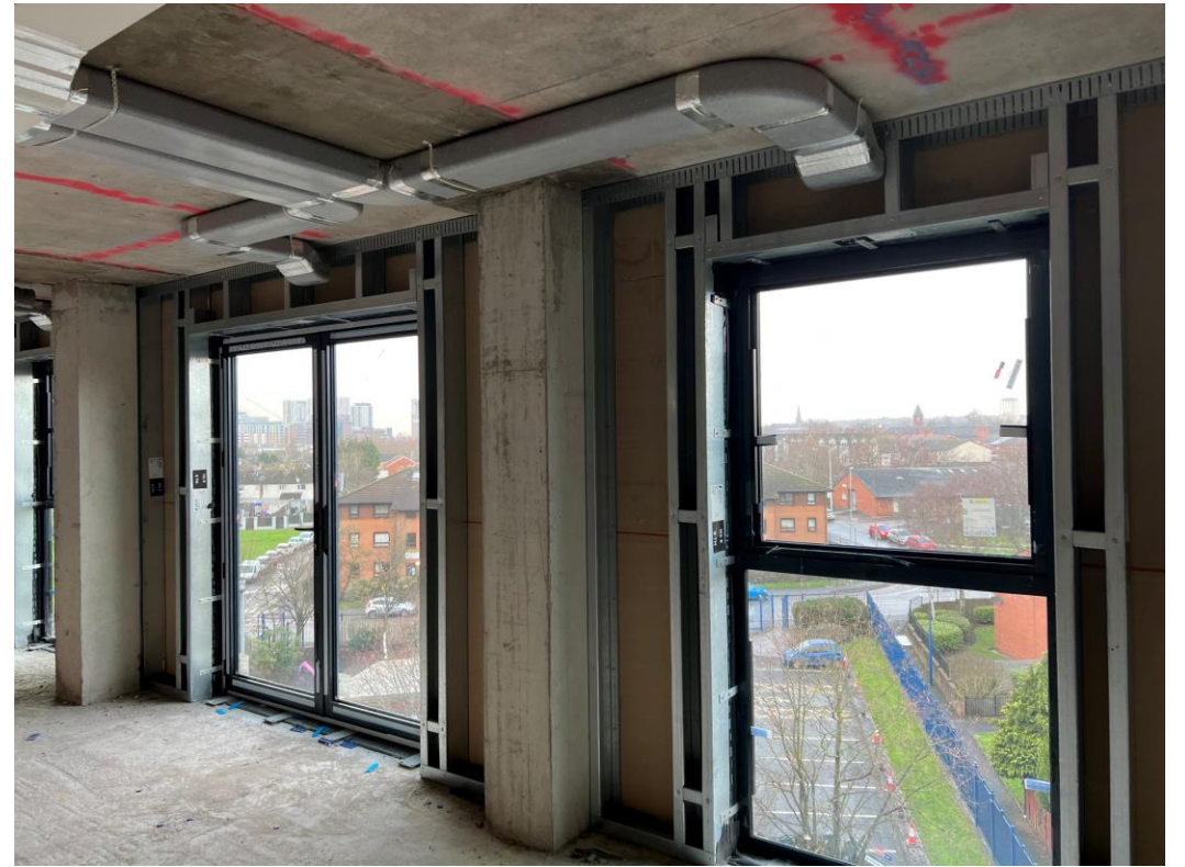
5 th Floor mechanical ducting
