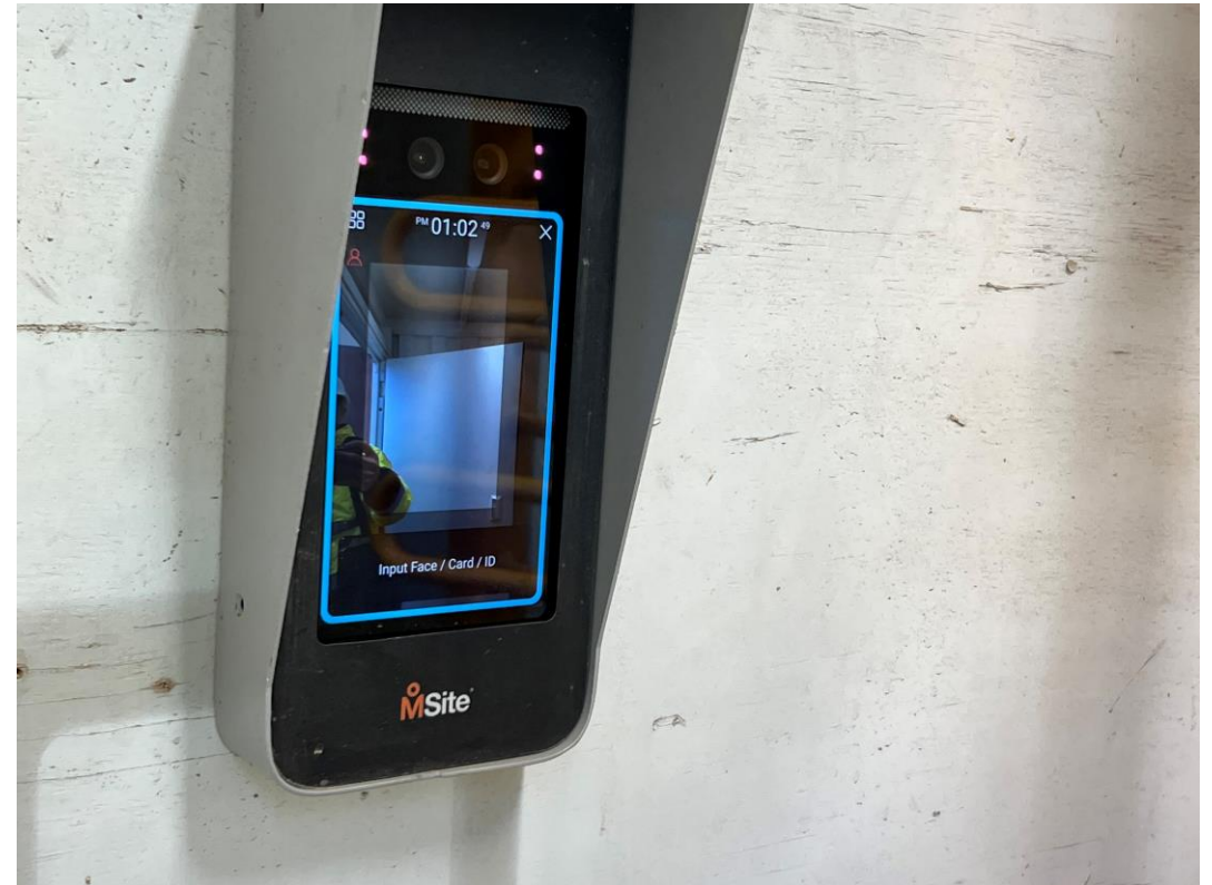
Worrall Street site entrance face recognition
