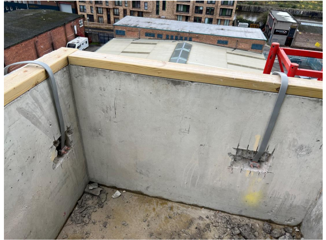
Block B – Parapet lightning tape
