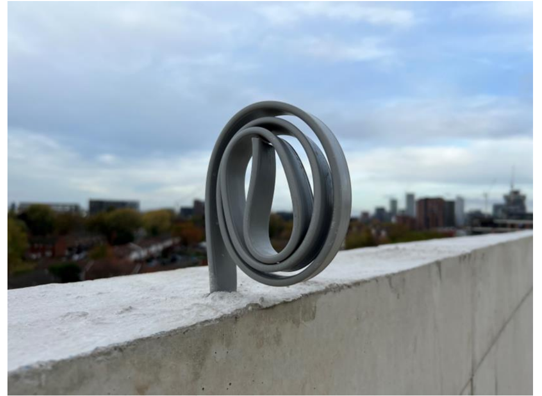
Block B – Lightning tape
