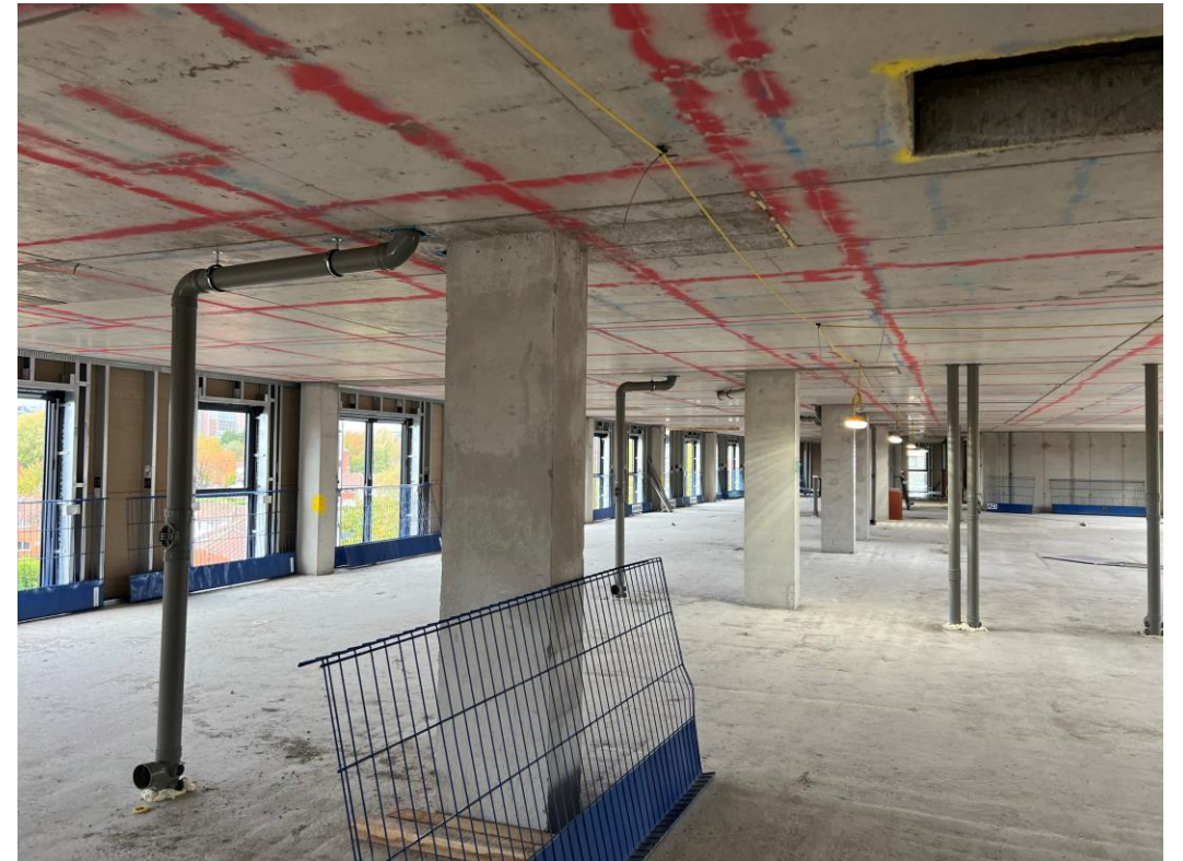
Upper floors drainage and mechanical ducting
