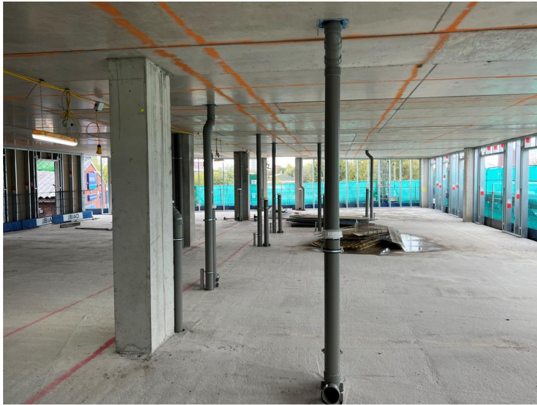
Upper floors above ground drainage
