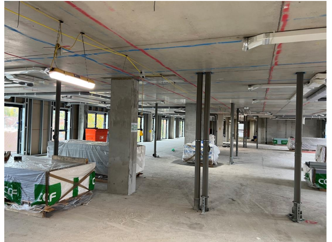
Upper floors drainage and mechanical ducting
