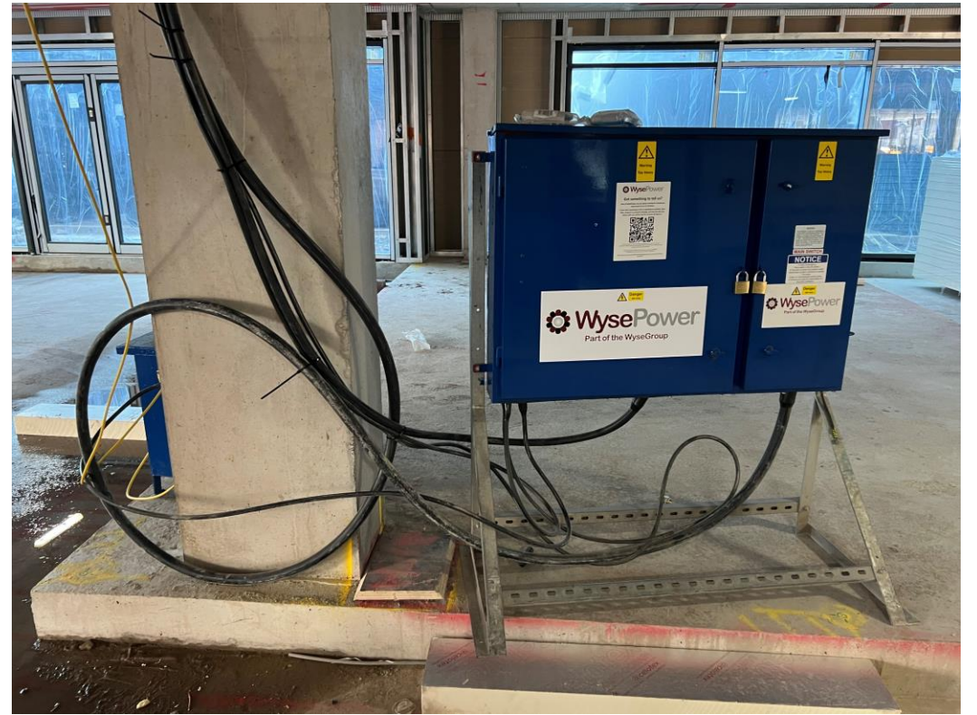
Block B temporary power
