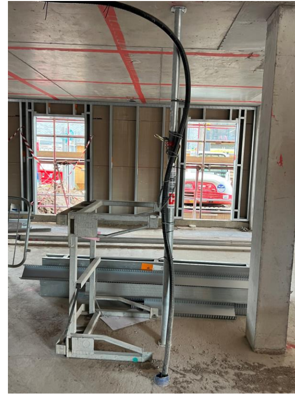
Block B electrical supply
