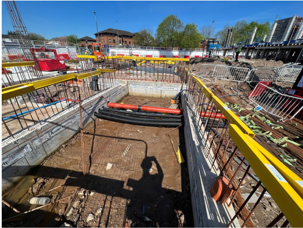
Block A underground services
