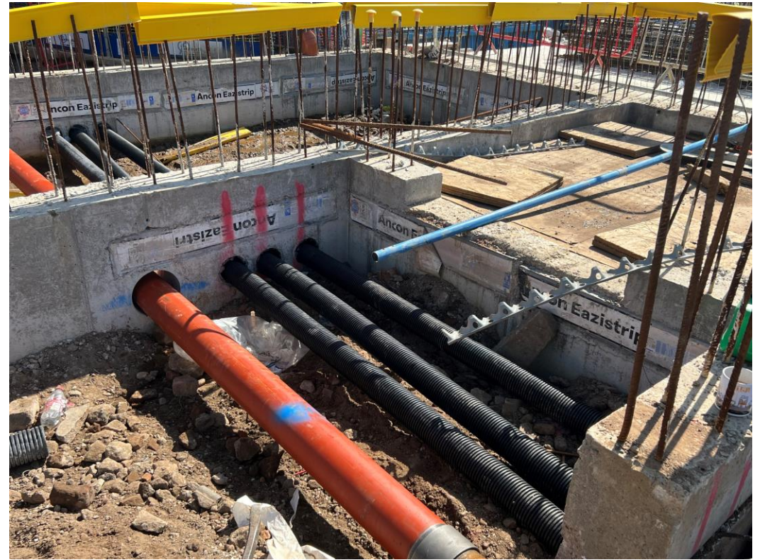
Block A underground services
