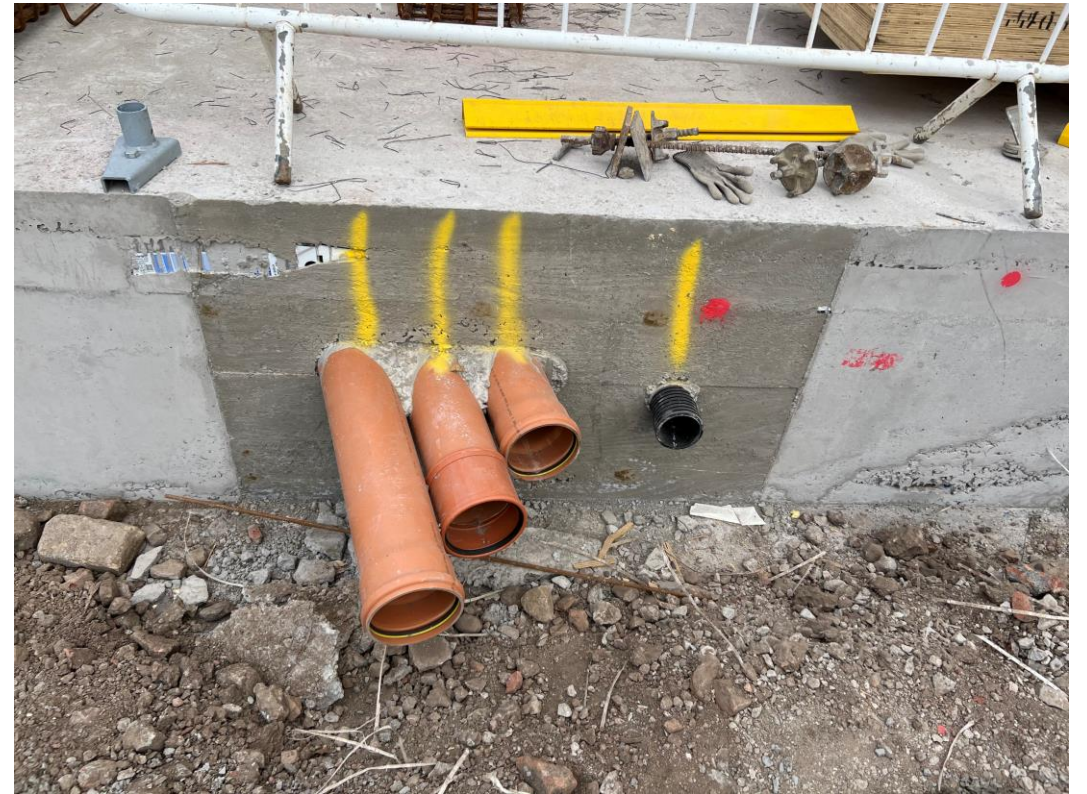
Block B concrete slab drainage
