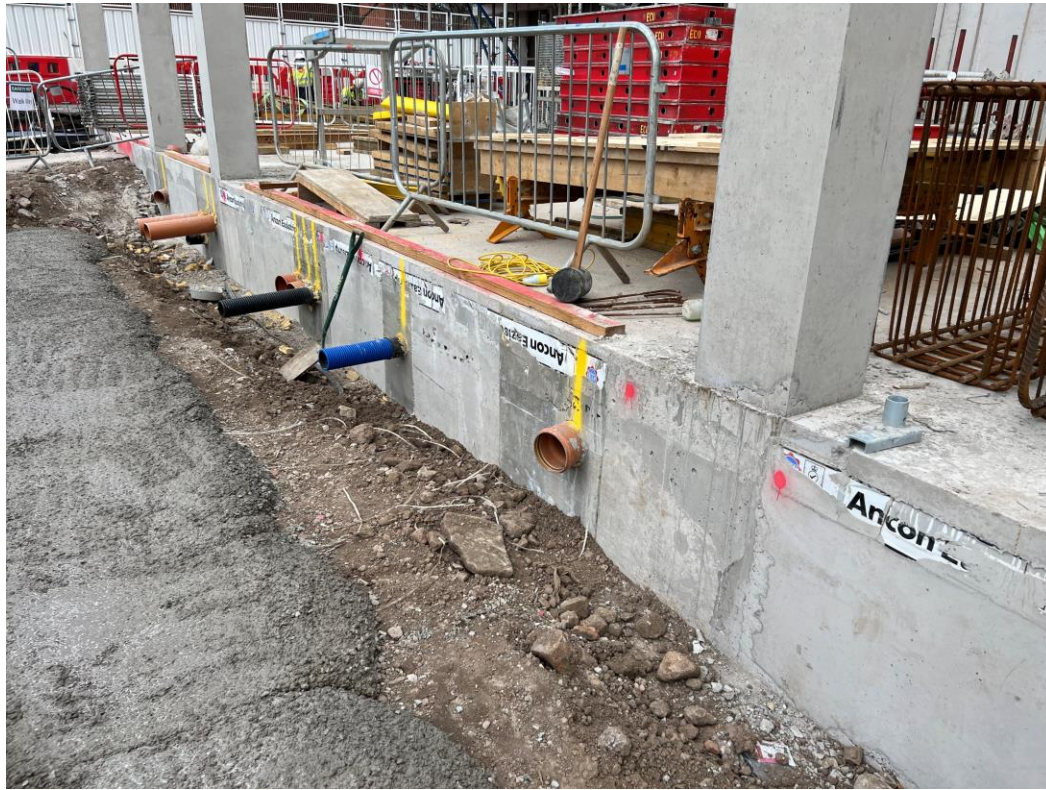
Block B concrete slab drainage
