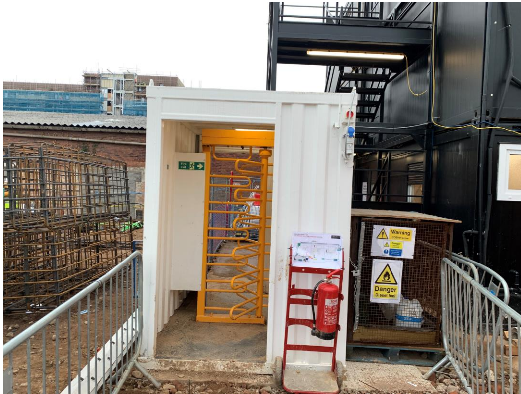
Face activate site access turnstile
