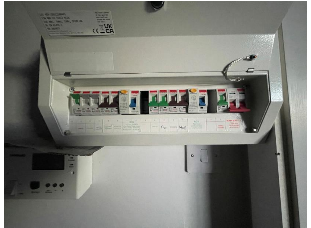
Level 6 – Electrical consumer unit
