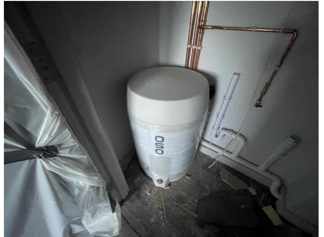
Level 6 – Mechanical appliances
