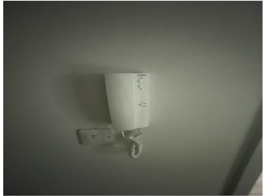
Level 6 – Telecom installed
