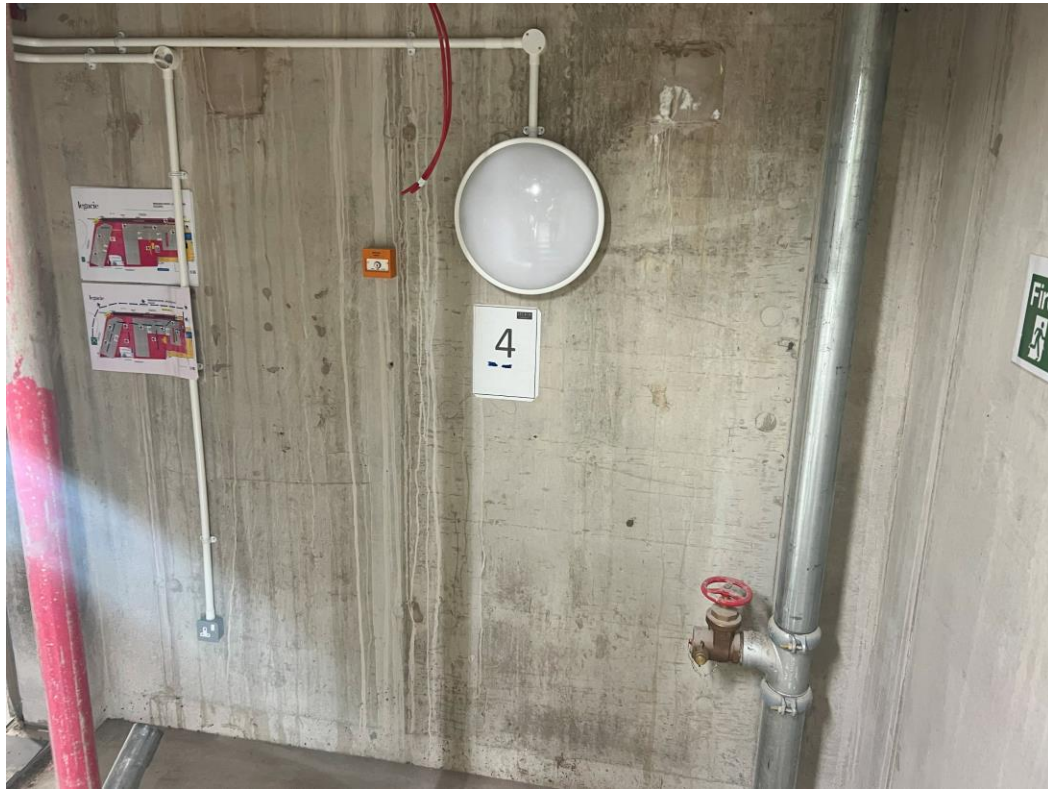
Stairwell lighting installed
