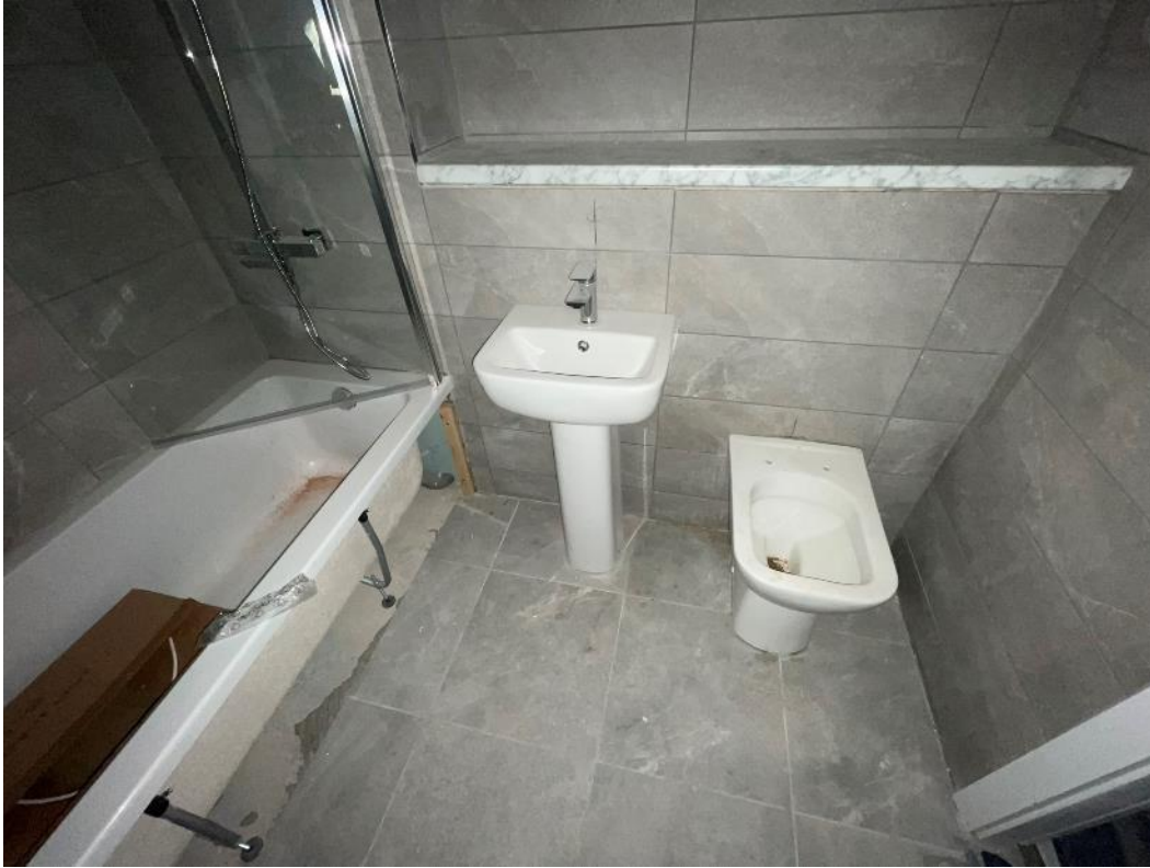
Level 5 – Sanitary items installed
