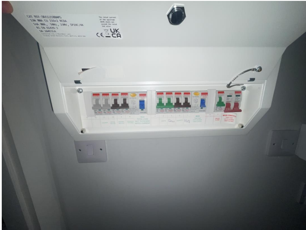
Level 1 – 2 nd fix electrical consumer unit
