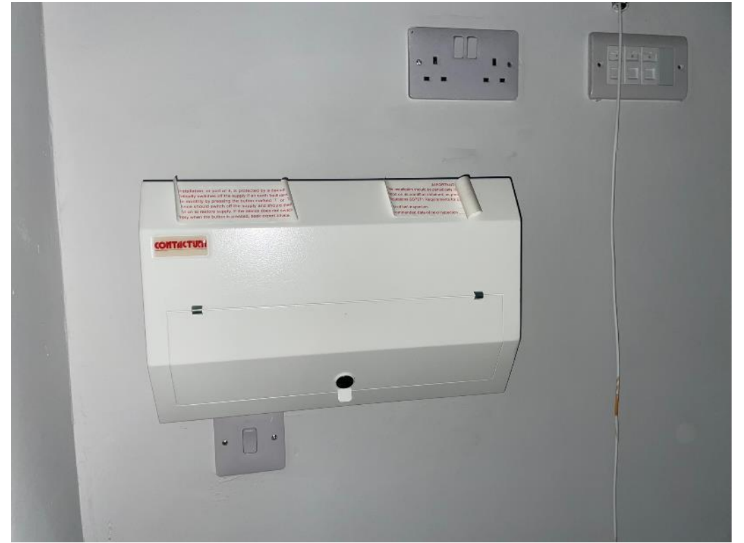
Level 2 – Electrical consumer unit
