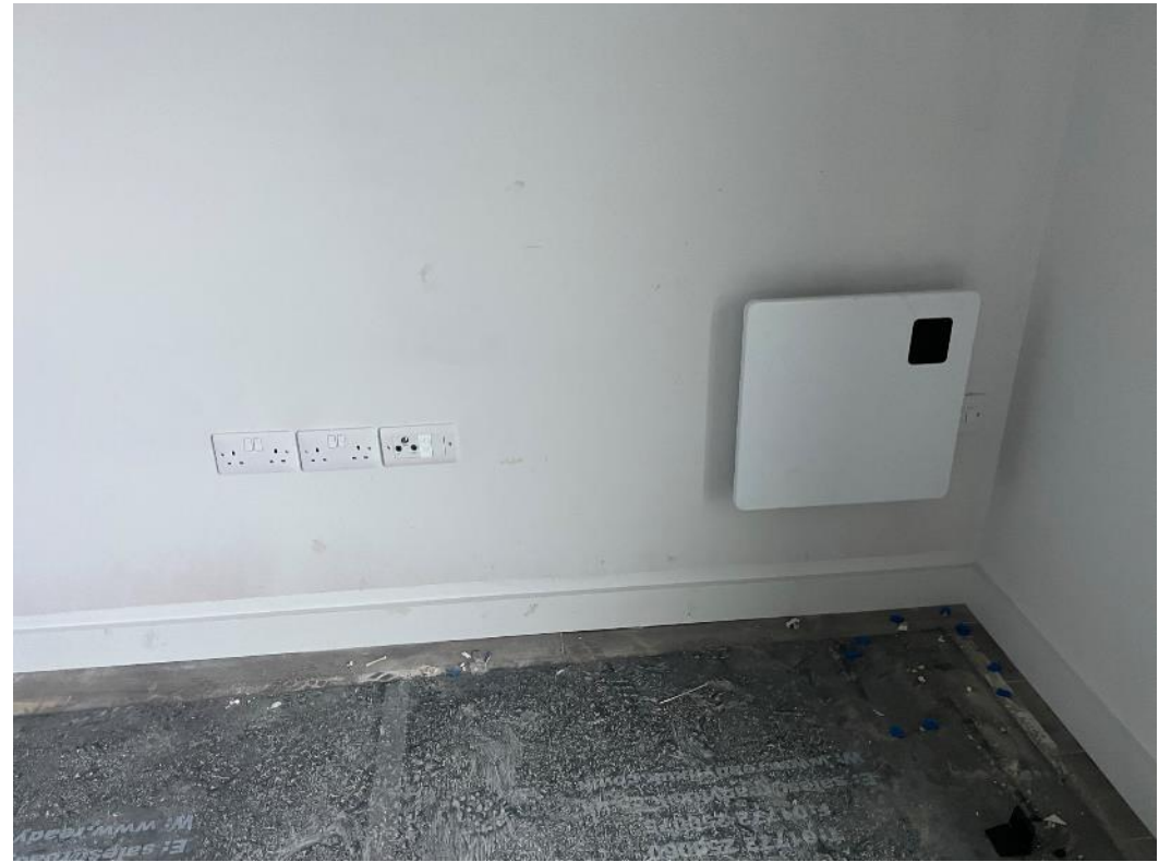
Level 8 – Mechanical appliances
