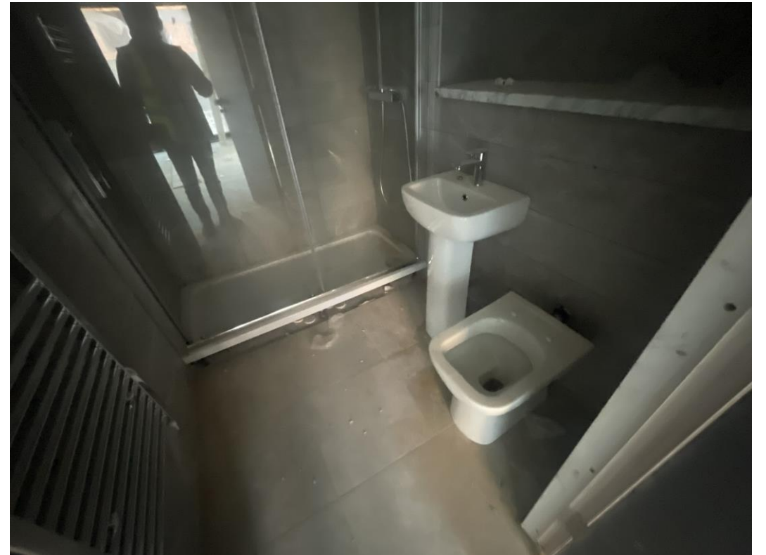
Level 1 – Sanitary fittings
