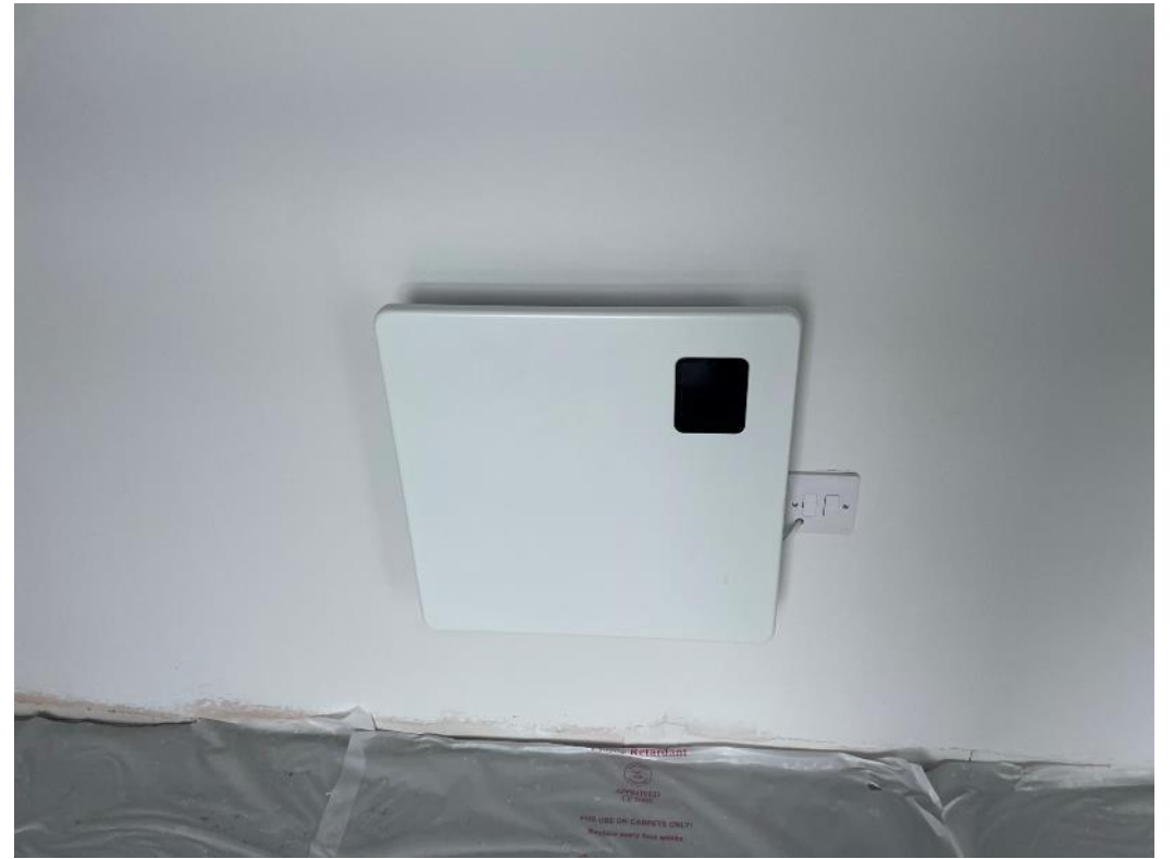
Level 4 – Wall panel heating
