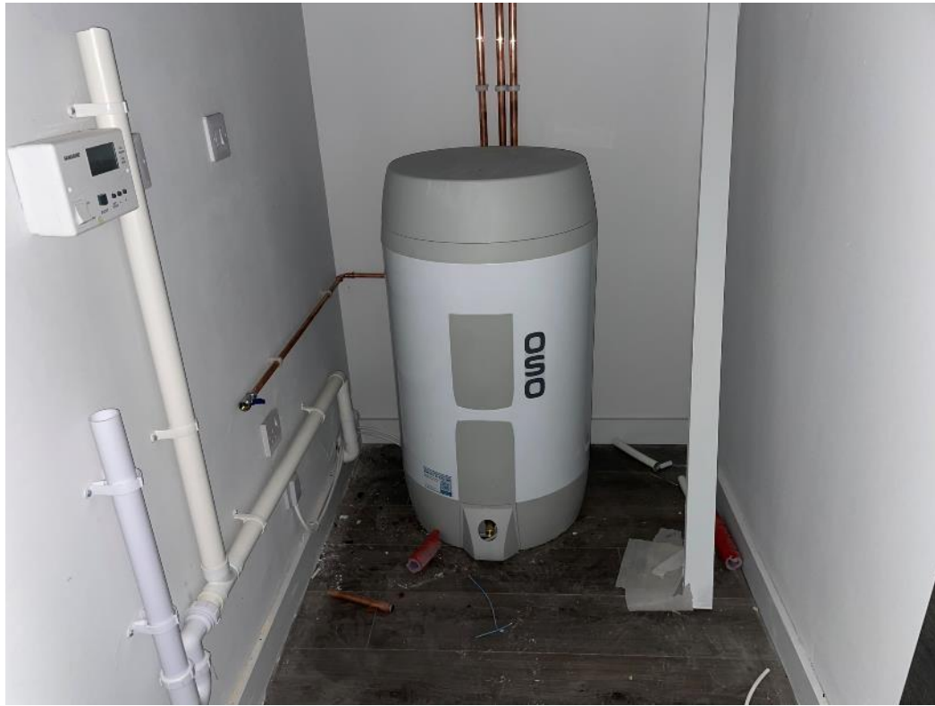
Level 2 – Mechanical appliances
