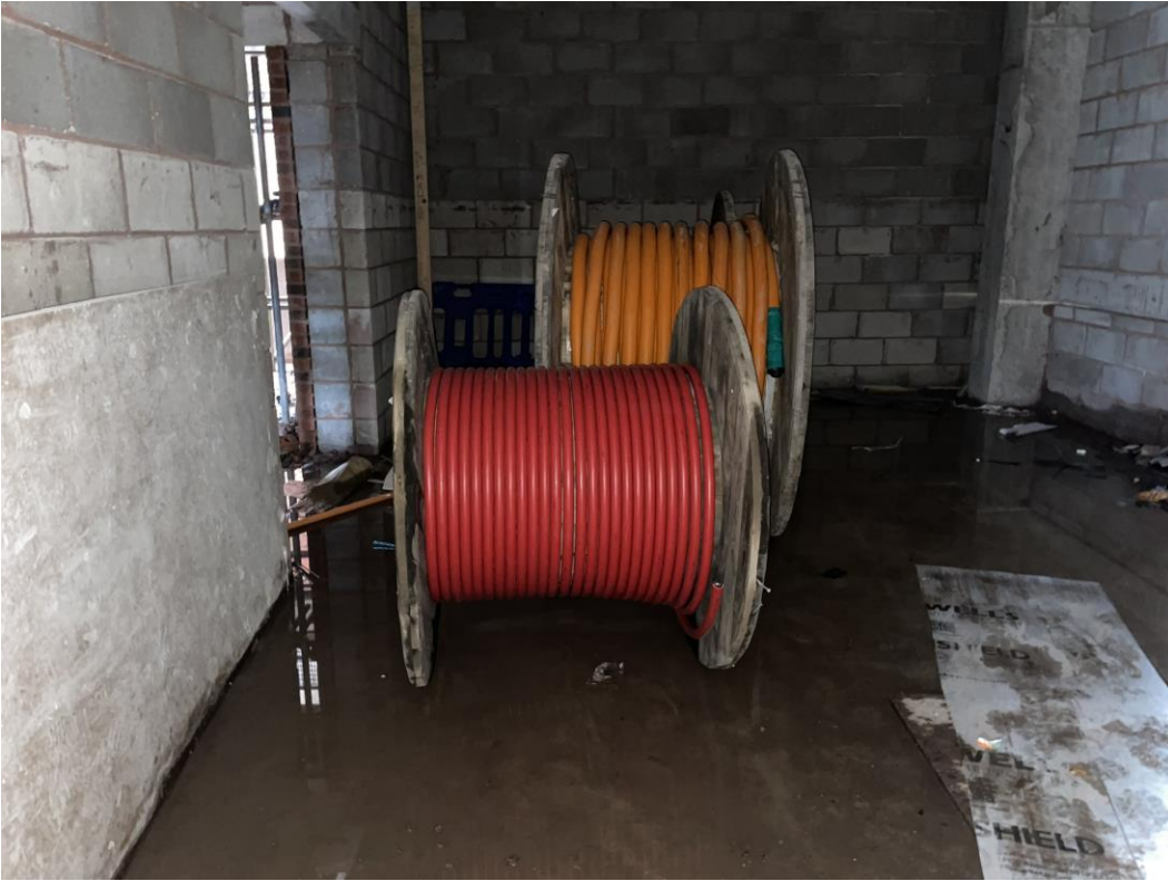
Electrical cables onsite for mains connection
