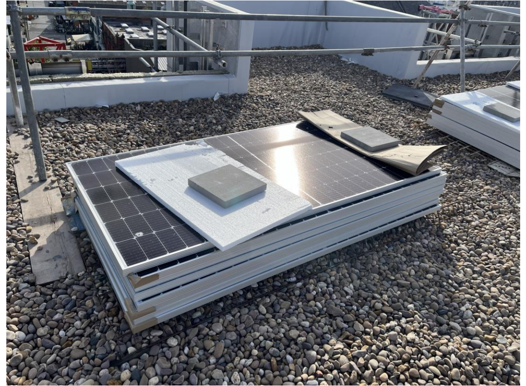
Block D Section B – Photovoltaics on site
