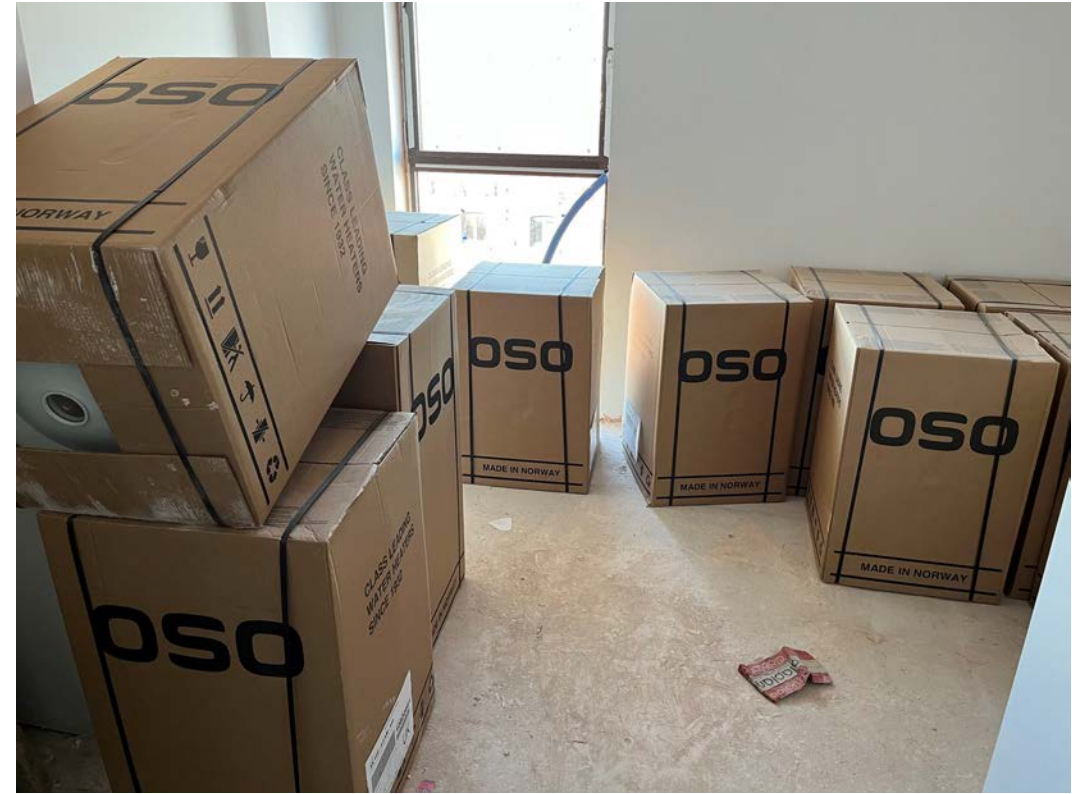
Hot water tanks on site
