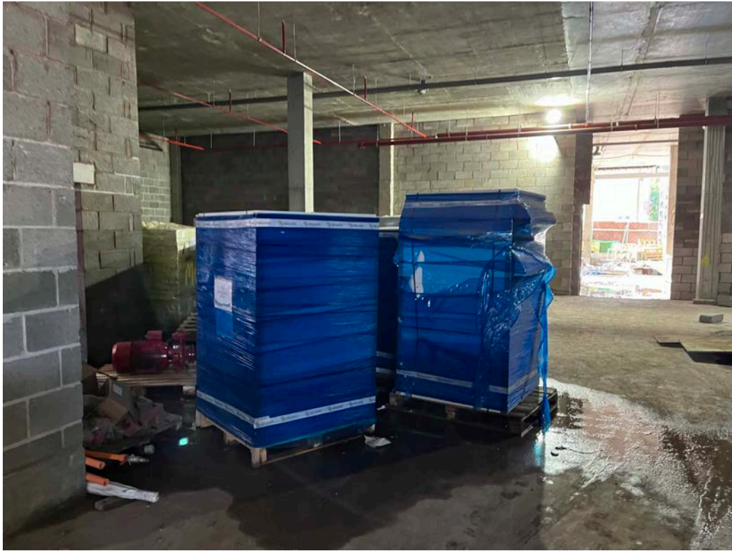
Sprinkler water tank on site
