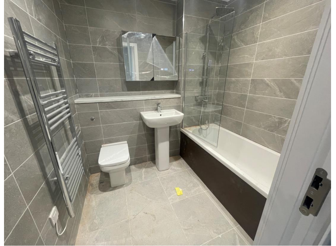
Sanitary appliances installed
