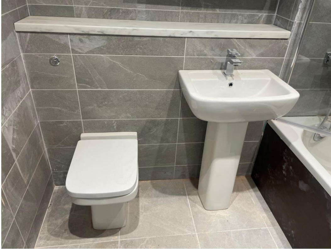
Sanitary appliances installed
