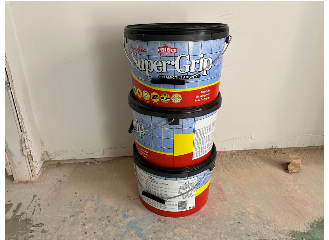
Ceramic tile adhesive onsite
