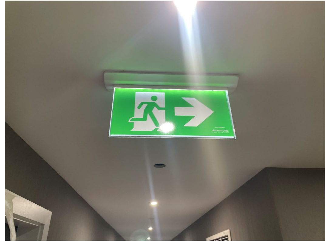
Escape signage installed
