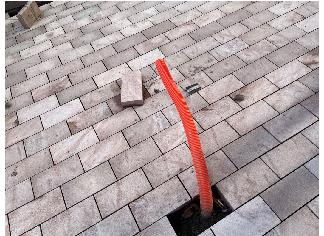
Ductwork for street lights
