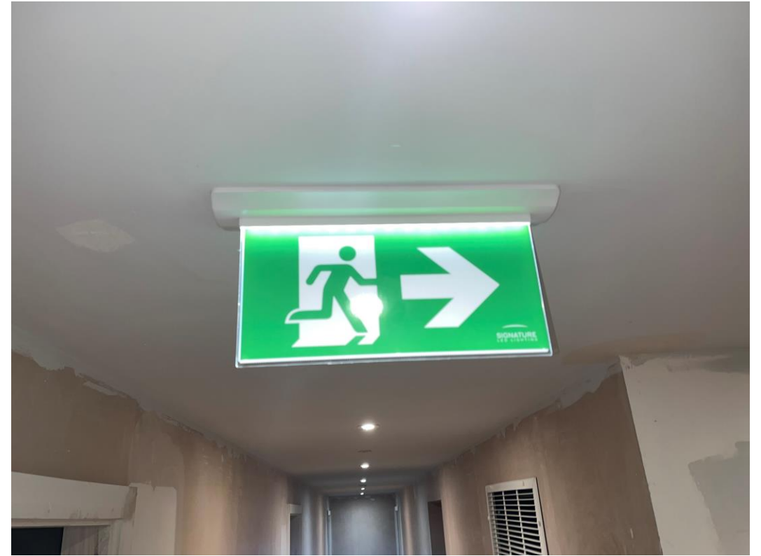
Emergency exit signs installed
