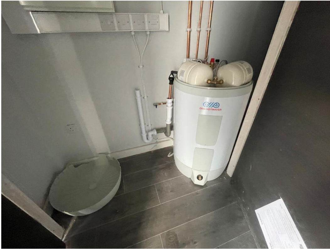
Water cylinder installed
