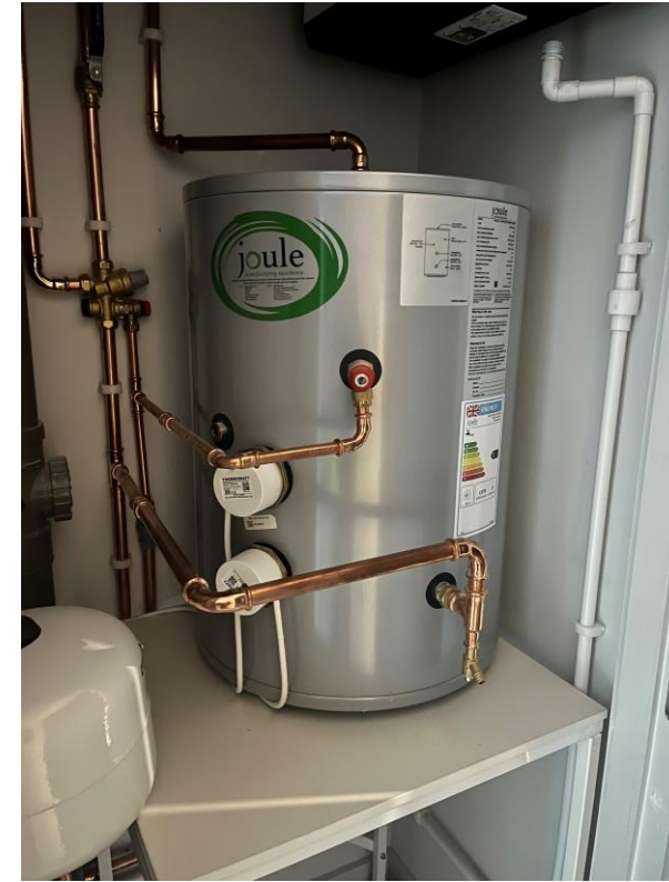
Water cylinder installed
