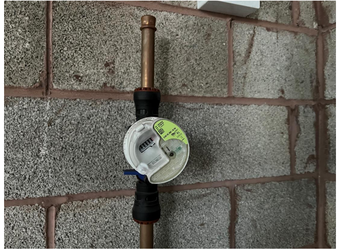
Commercial unit water meter installed
