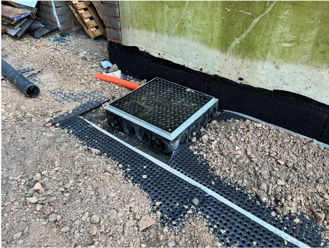
Electrical junction box installed
