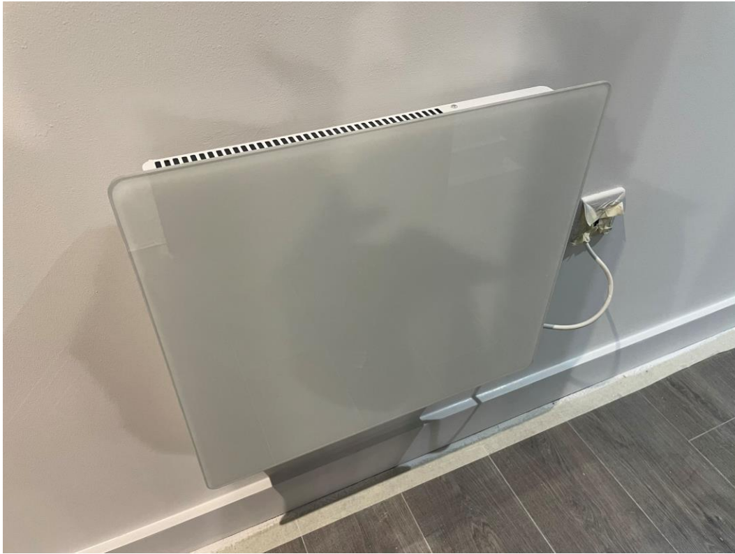
Electric wall heater installed
