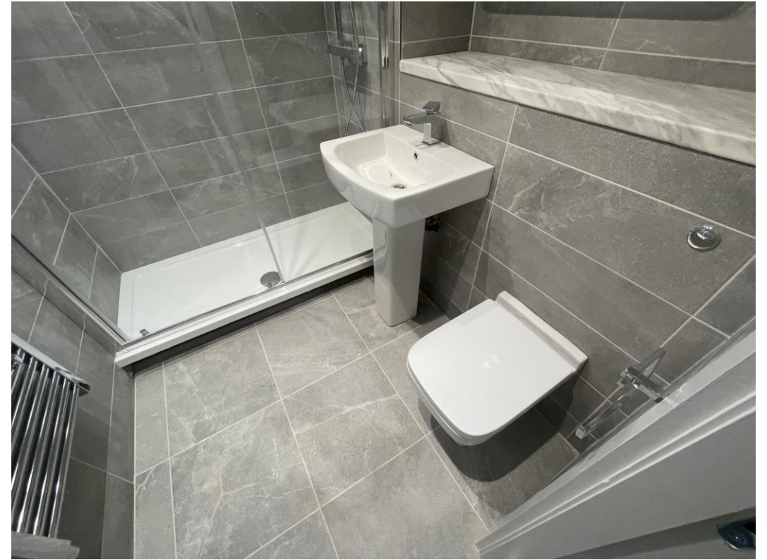
Ensuite sanitary items installed
