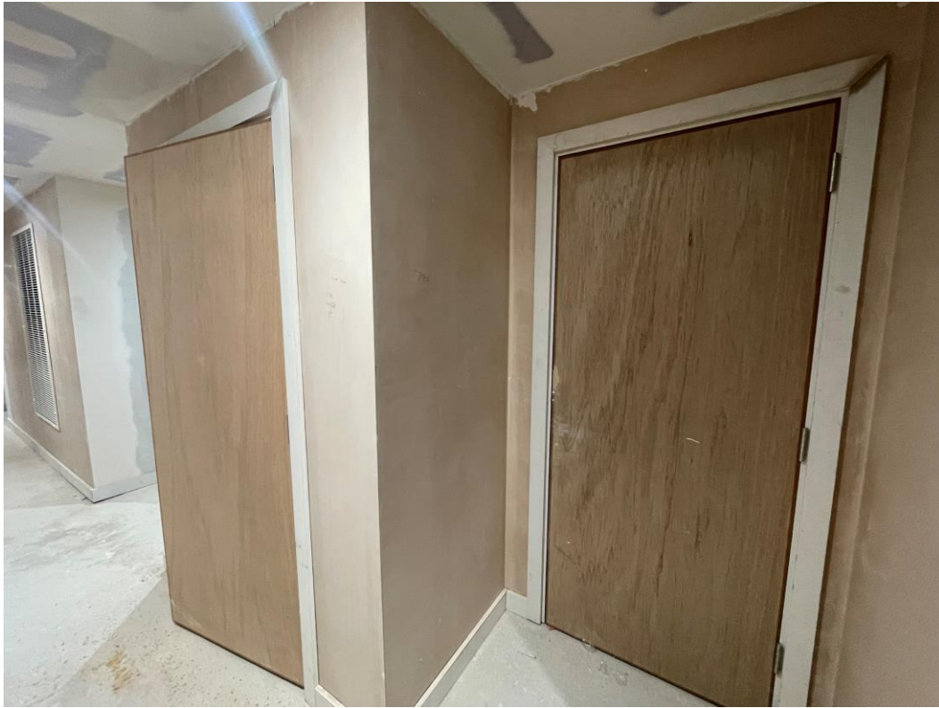
Doors installed to water distribution cupboard
