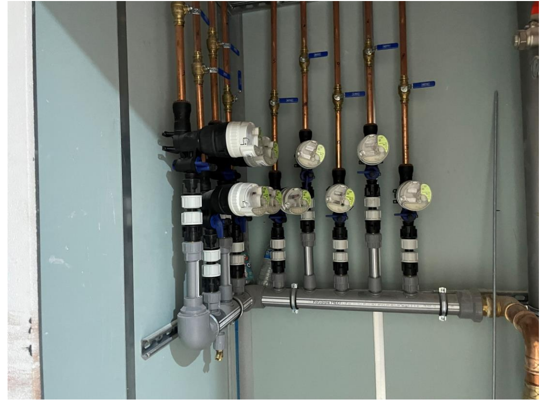
Water meters installed
