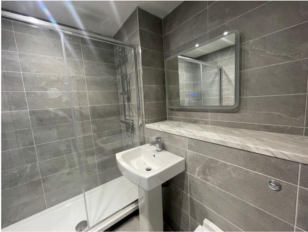
Ensuite mirrors installed
