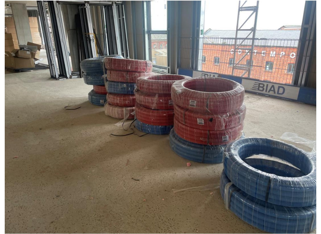
Apartment water distribution pipeworkk
