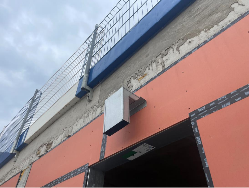
Block D – External mechanical ventilation
