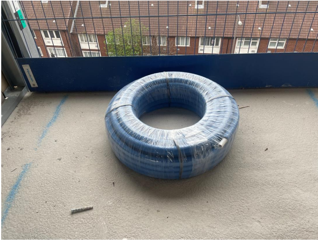
Apartment water distribution pipeworkk
