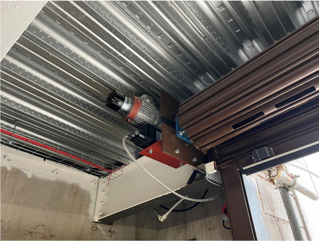
Roller shutter motor installed
