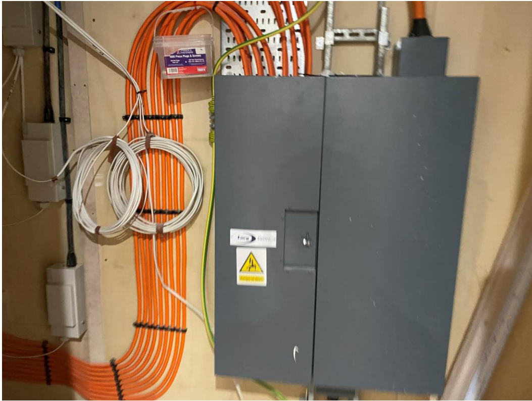
Electrical distribution board installed
