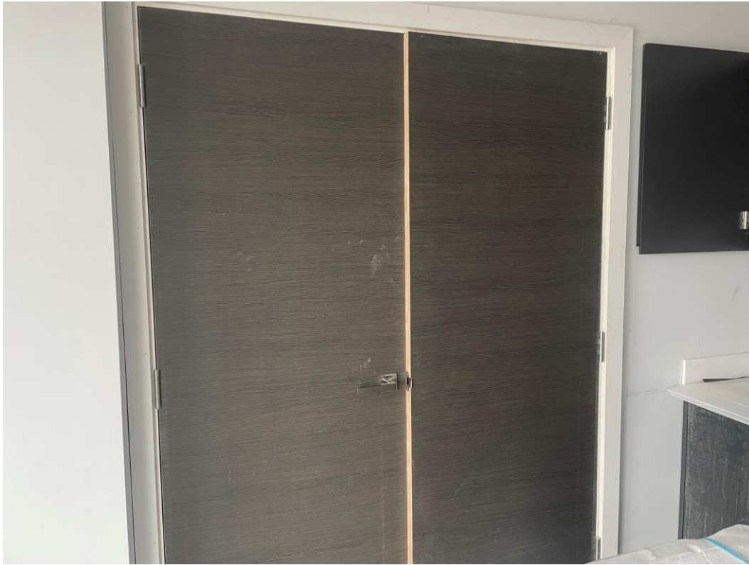
Apartment doors & ironmongery
