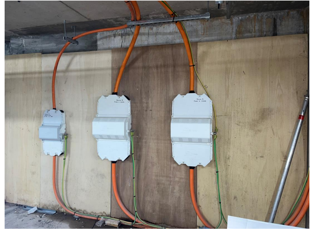
Mains electrical supply
