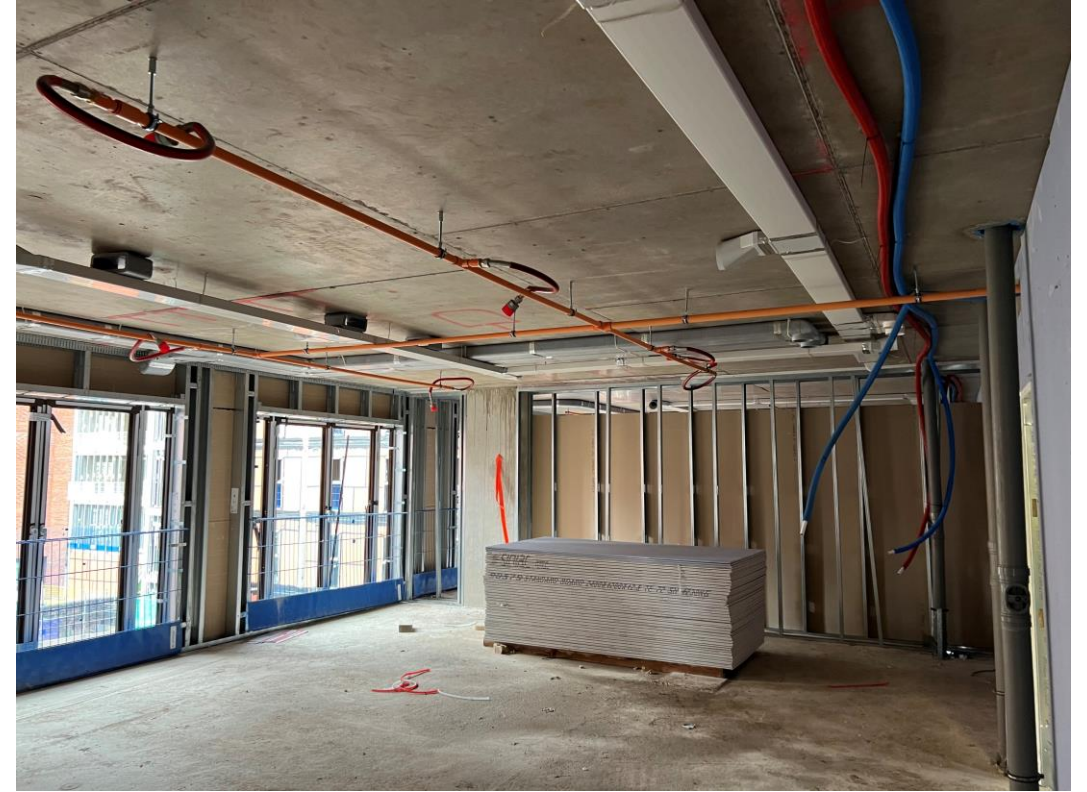
Sprinkler system pipe work installed
