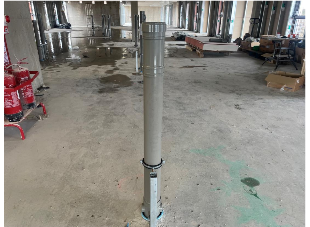
Above ground drainage
