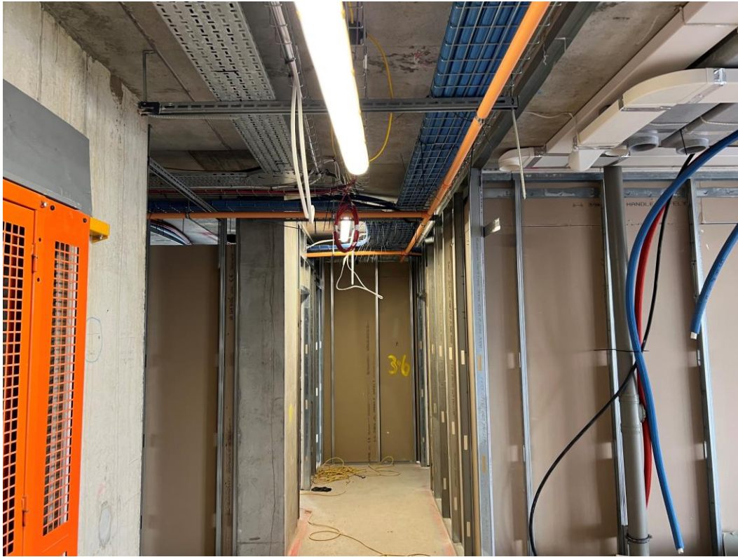
Sprinkler system pipe work installed
