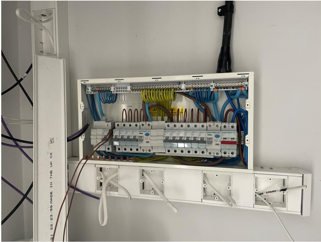
Electric consumer unit installed
