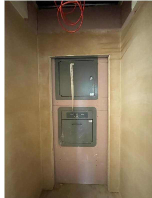
Bin shoot installation
