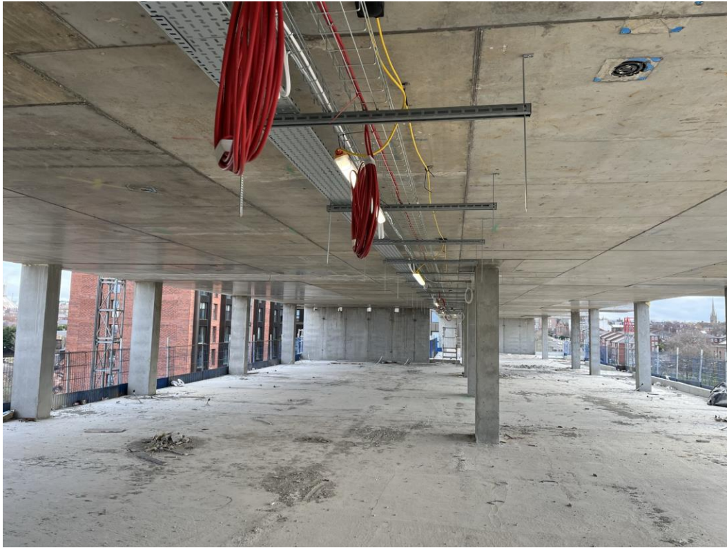
Electrical containment in place
