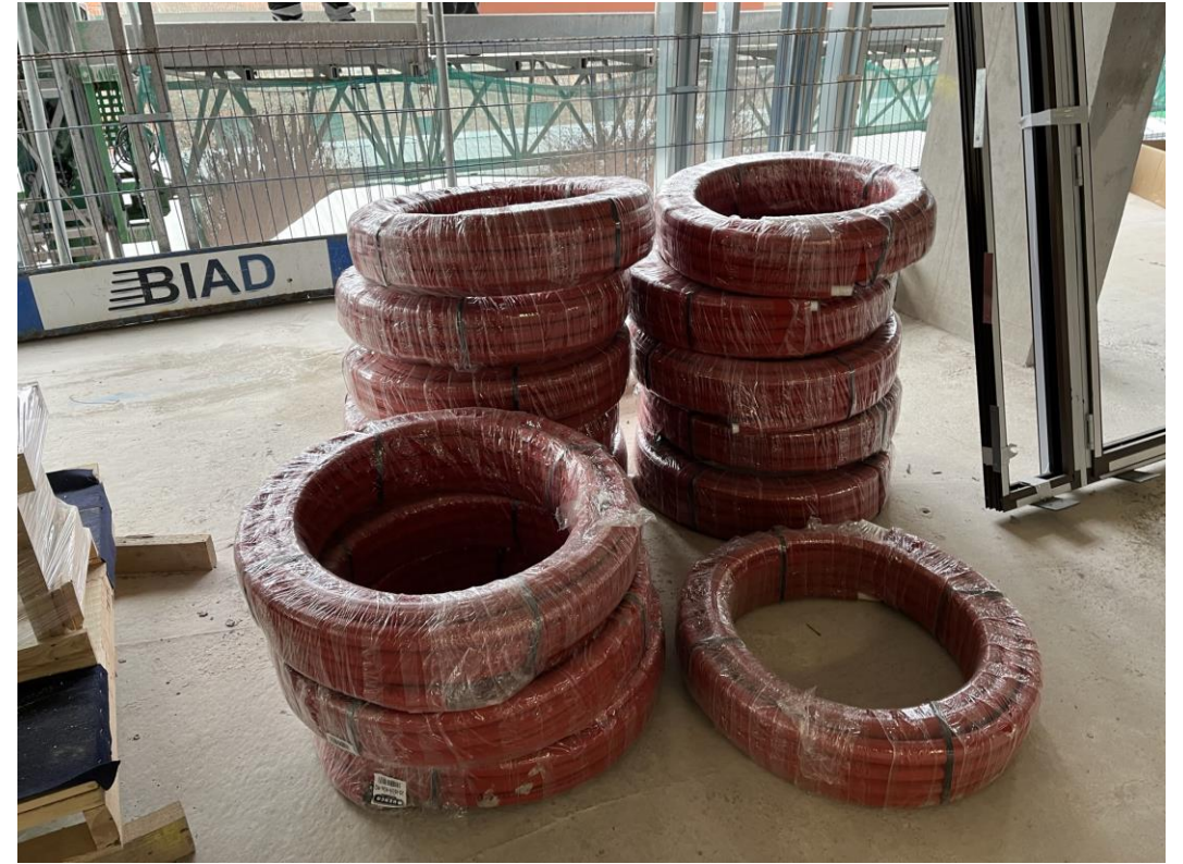
Hot water distribution pipework
