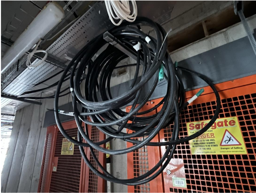
Electrical mains distribution in place
