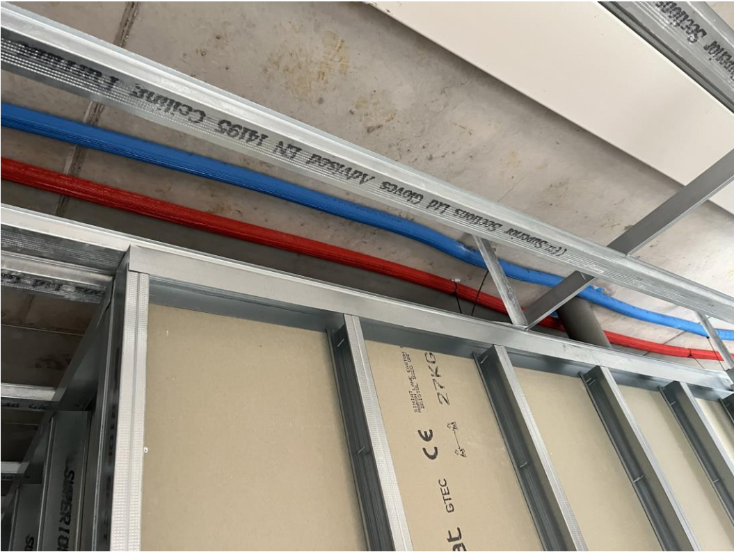
Water distribution to apartments
