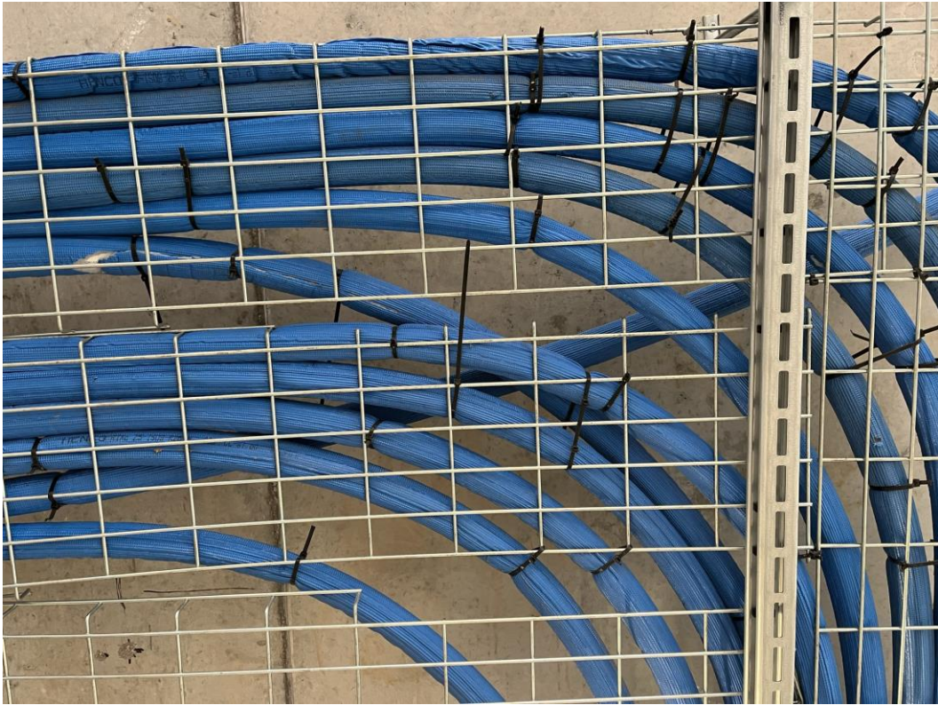
Water distribution to apartments
