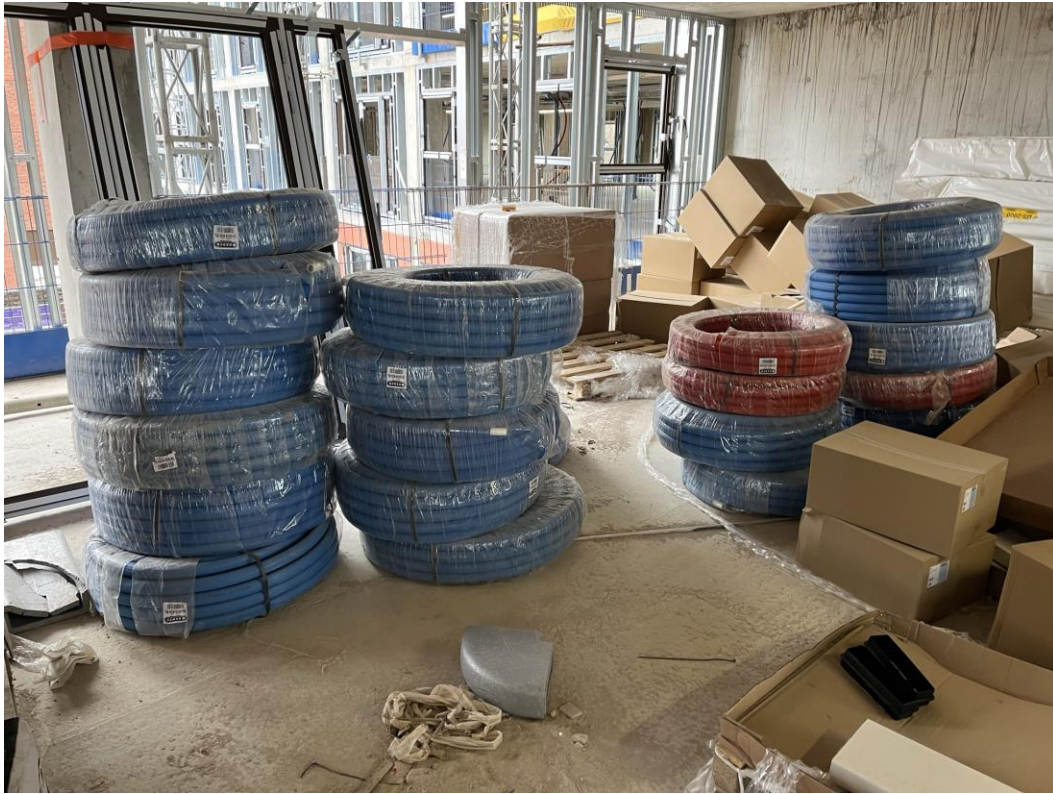
Cold water distribution pipework
