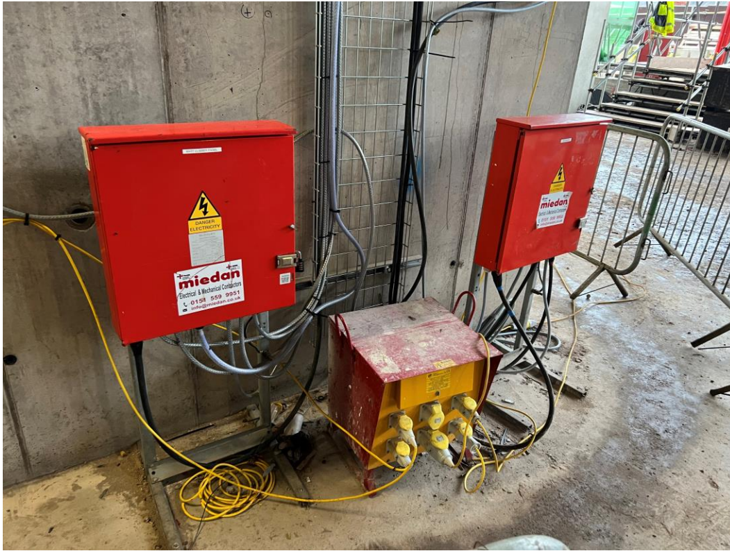
Temporary power live
