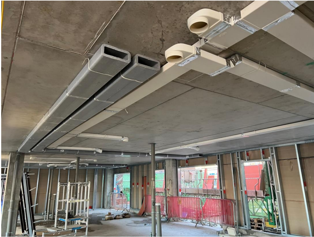
Block D Section A – Ductwork
