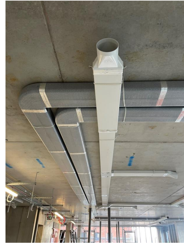
Block D Section A – Ductwork
