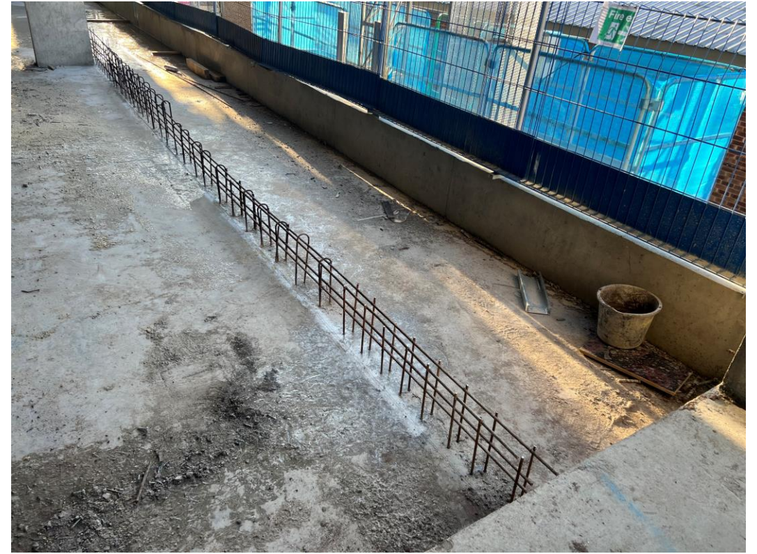
Block D Section C – Reinforcement in place for formation of concrete upstand
