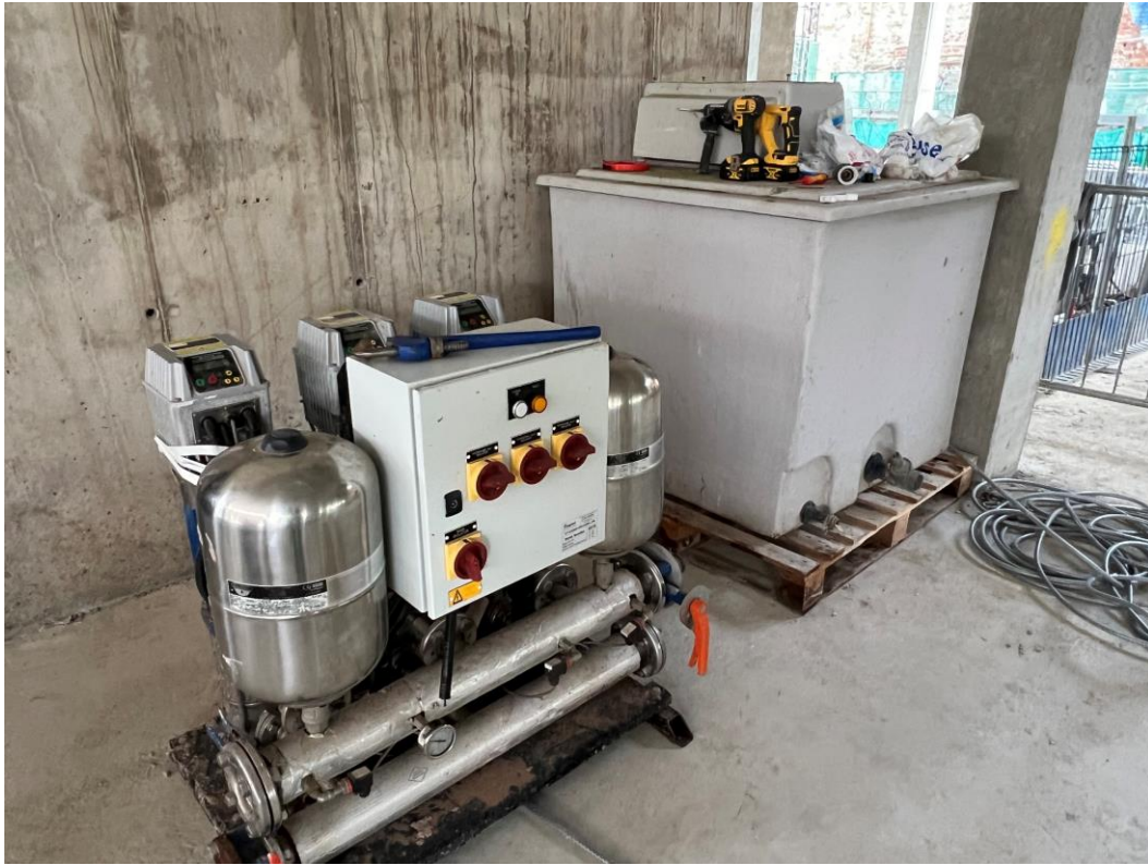
Plant onsite for installation
