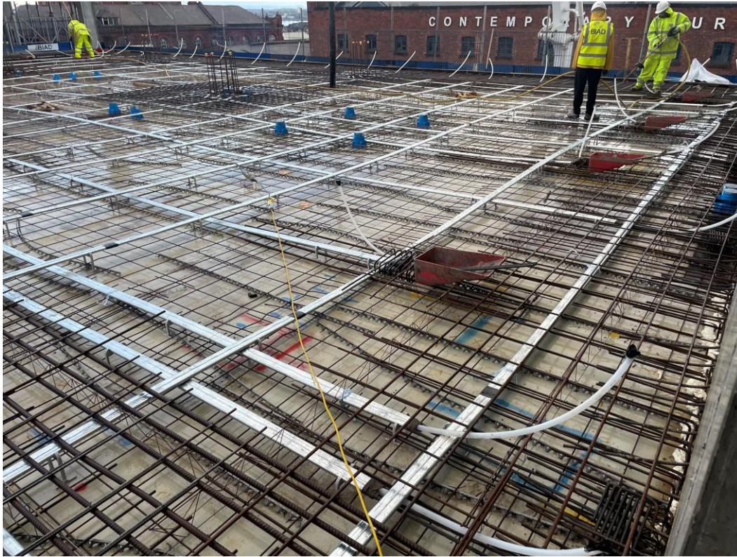
Section C – Preparation works ongoing for Level 4 concrete pour with reinforcement laid
