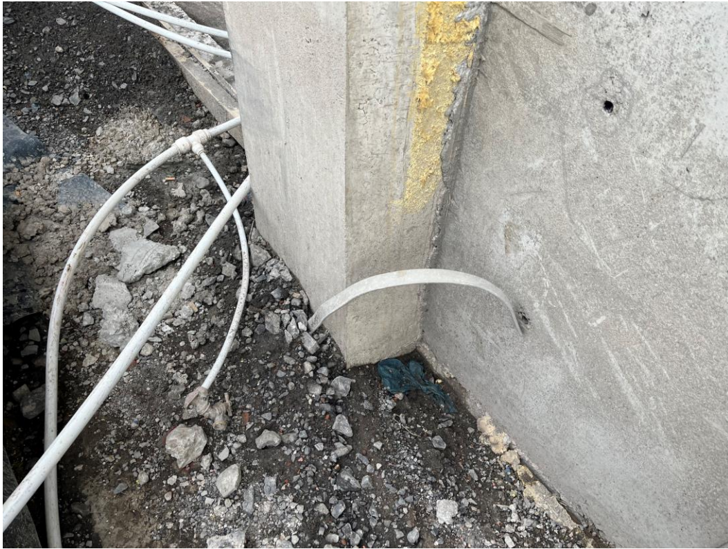
Lightning Conductor Cable in place
