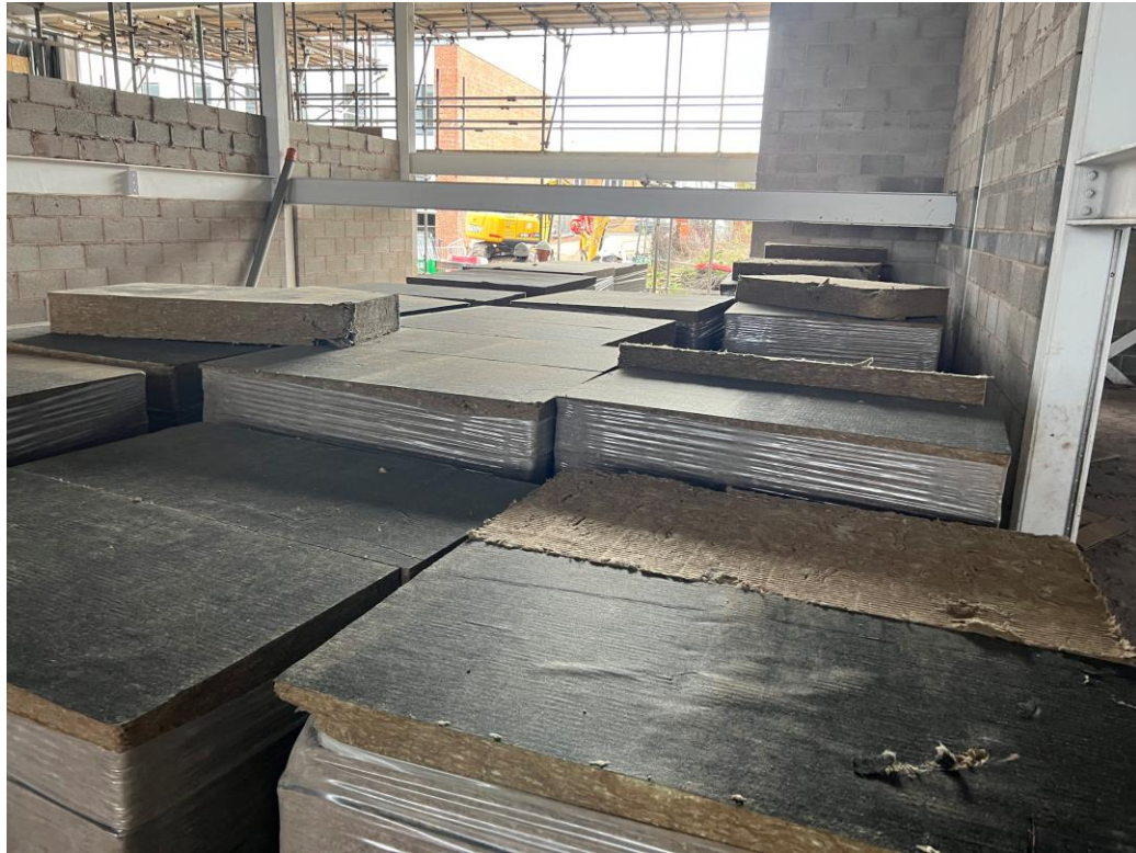
Commercial block ceiling insulation
