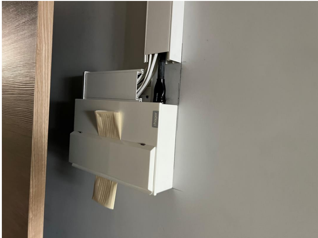
Student Wing – Consumer unit installation
