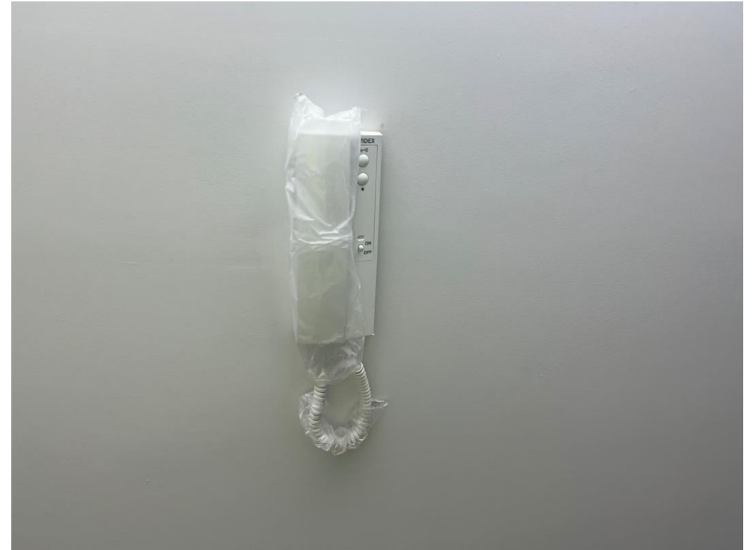
Student Wing – Telephone Intercom
