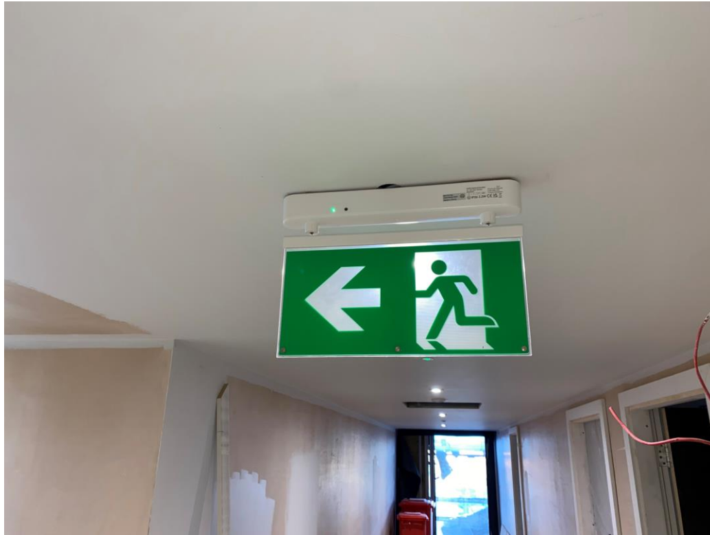
Residential Block – Fire exit signage
