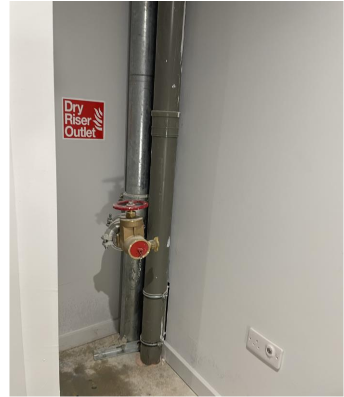
Residential Wing – Dry riser
