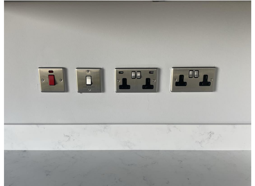
Residential Wing – Electrical sockets & switches
