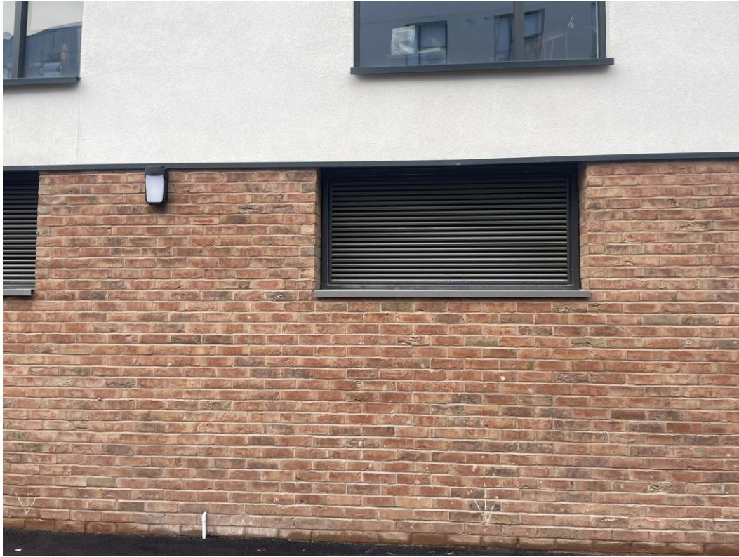
Louvre ventilation grills
