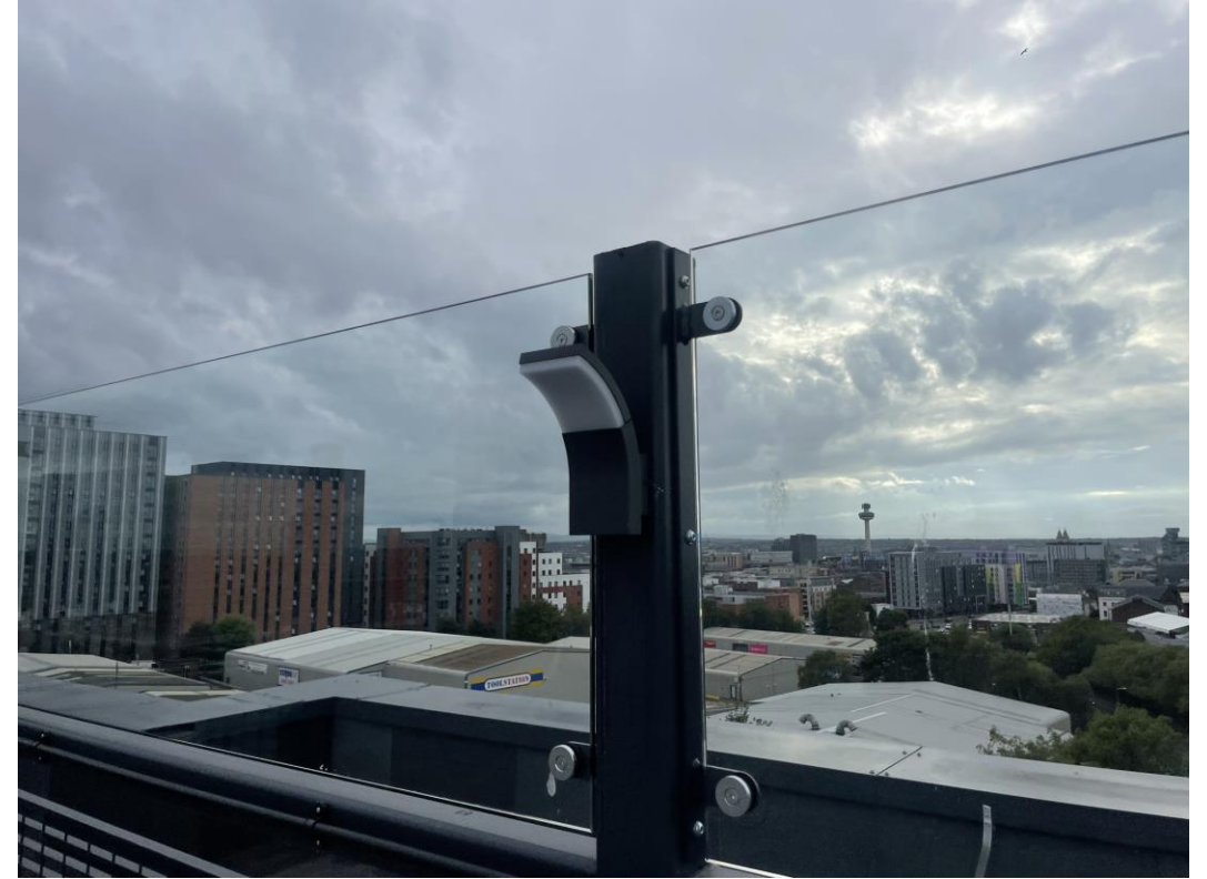
Residential Block – Light fittings installed
