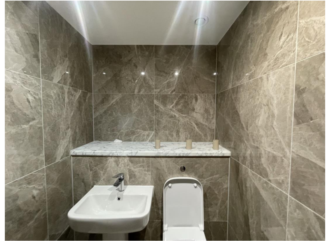
Ground Floor WC – Sanitary Items
